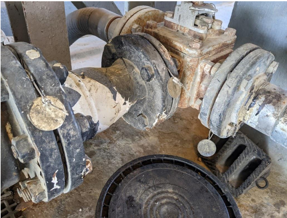
Photograph 2 of 6: Illegible Tags on Ancillary Equipment Subject to Subpart BB
