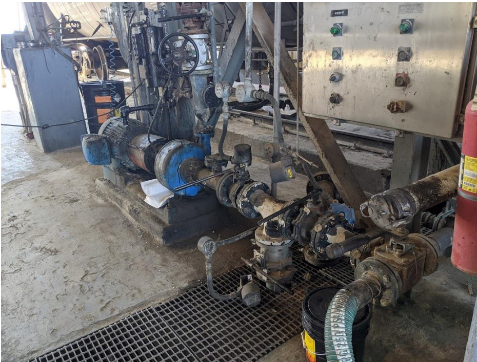
Photograph 3 of 6: Ancillary Equipment Managing Waste Subject to Subpart BB
