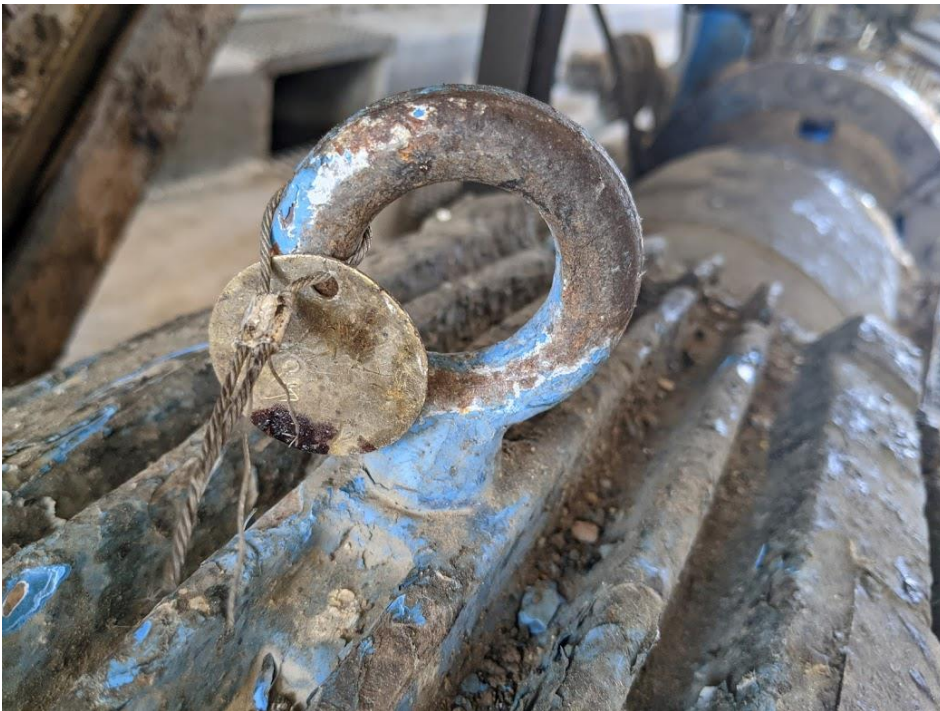
Photograph 1 of 6: Illegible Tag on Ancillary Equipment Subject to Subpart BB
