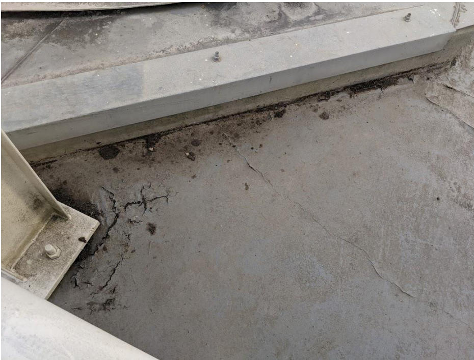
Photograph 6 of 6: Cracks in Secondary Containment for Hazardous Waste Storage
