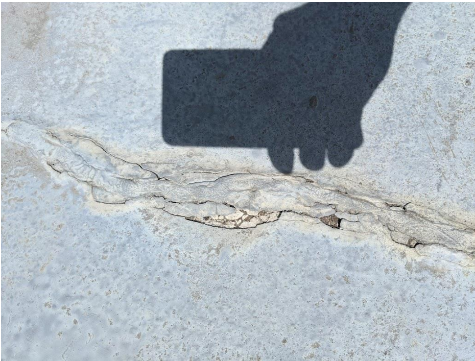
Photograph 5 of 6: Cracks in Secondary Containment for Hazardous Waste Storage
