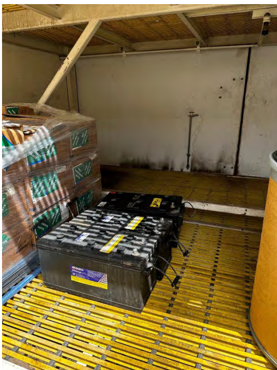
Photograph 8: UW batteries at the UW Storage Area.
