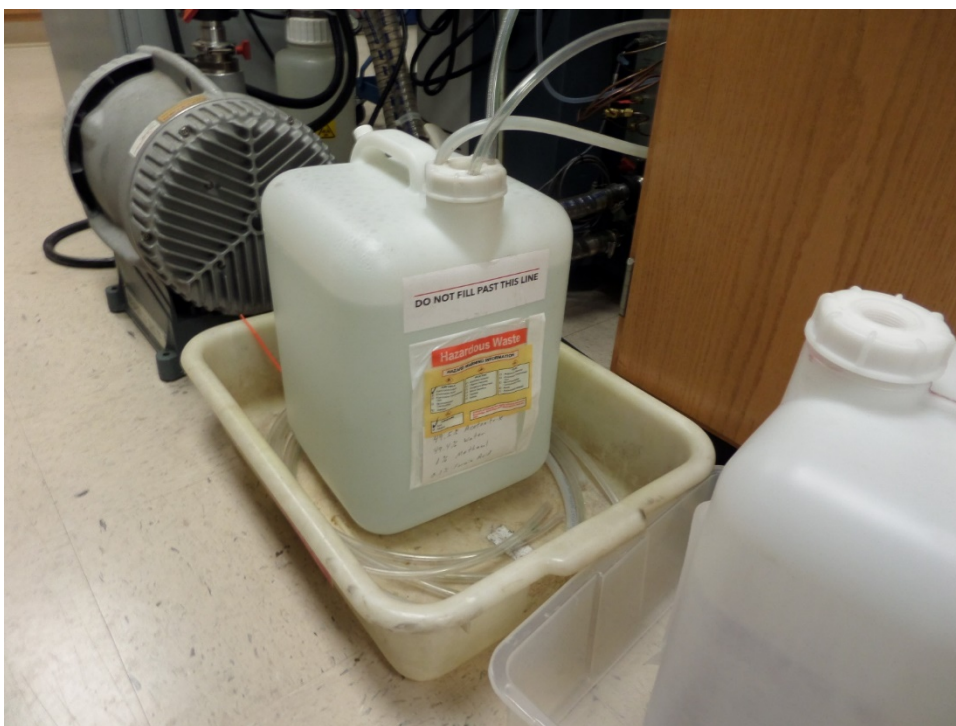
Photograph 13: Hazardous wastes accumulation container observed in Room 201, operated by the USDA.
