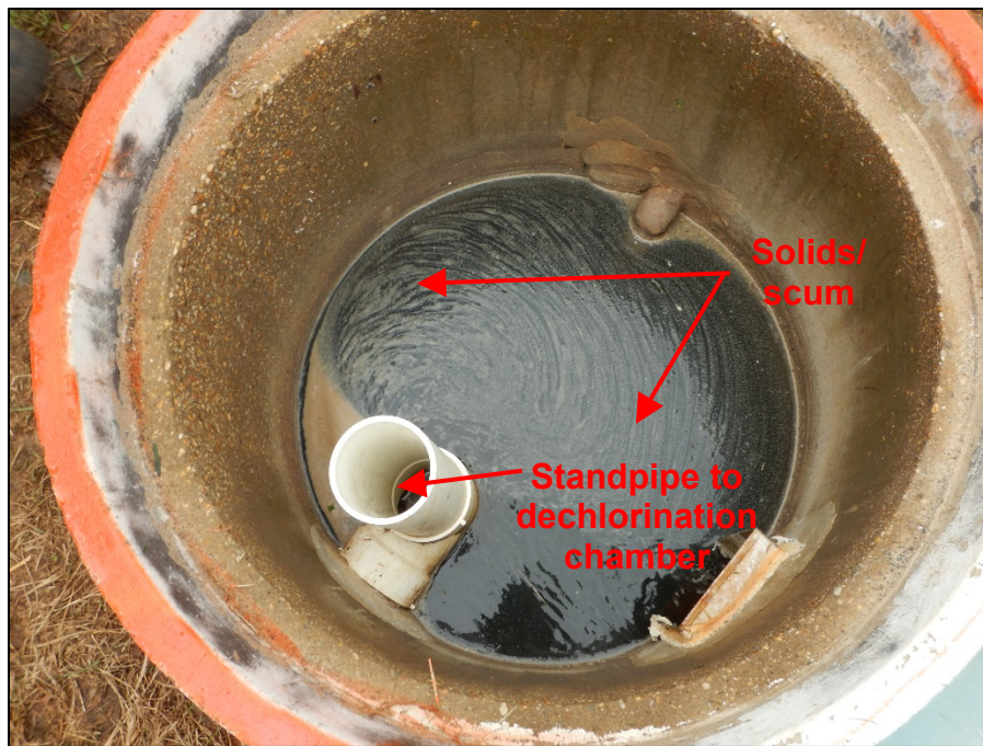
Photograph 11. View of chlorine contact chamber. Note that solids and scum was observed on the water's surface. The solids and scum did not appear to be getting into the standpipe and were not noticeable in the post aeration basin or at Outfall 001.
