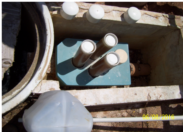
5. Chlorine contact tank
