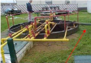
Treatment Plant - See Line to Beds
