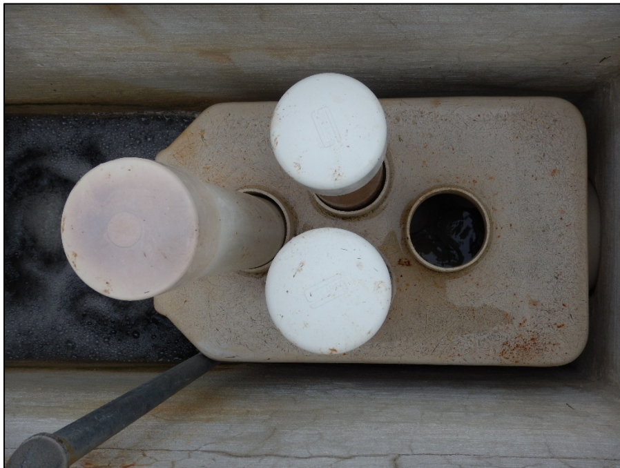
Photograph 12. View of tubes used for delivering sodium bisulfite tablets to the effluent.
