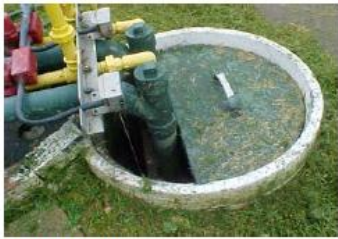
Air Lift Tank
