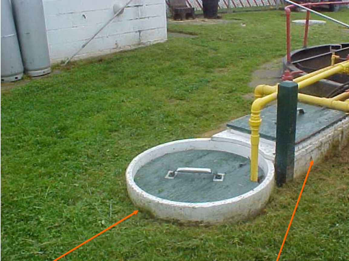
Chlorine Contact w/ Post Aeration
