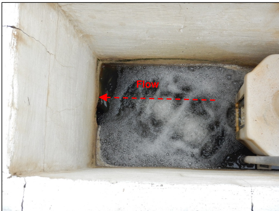
Photograph 13. View inside the post aeration basin.
