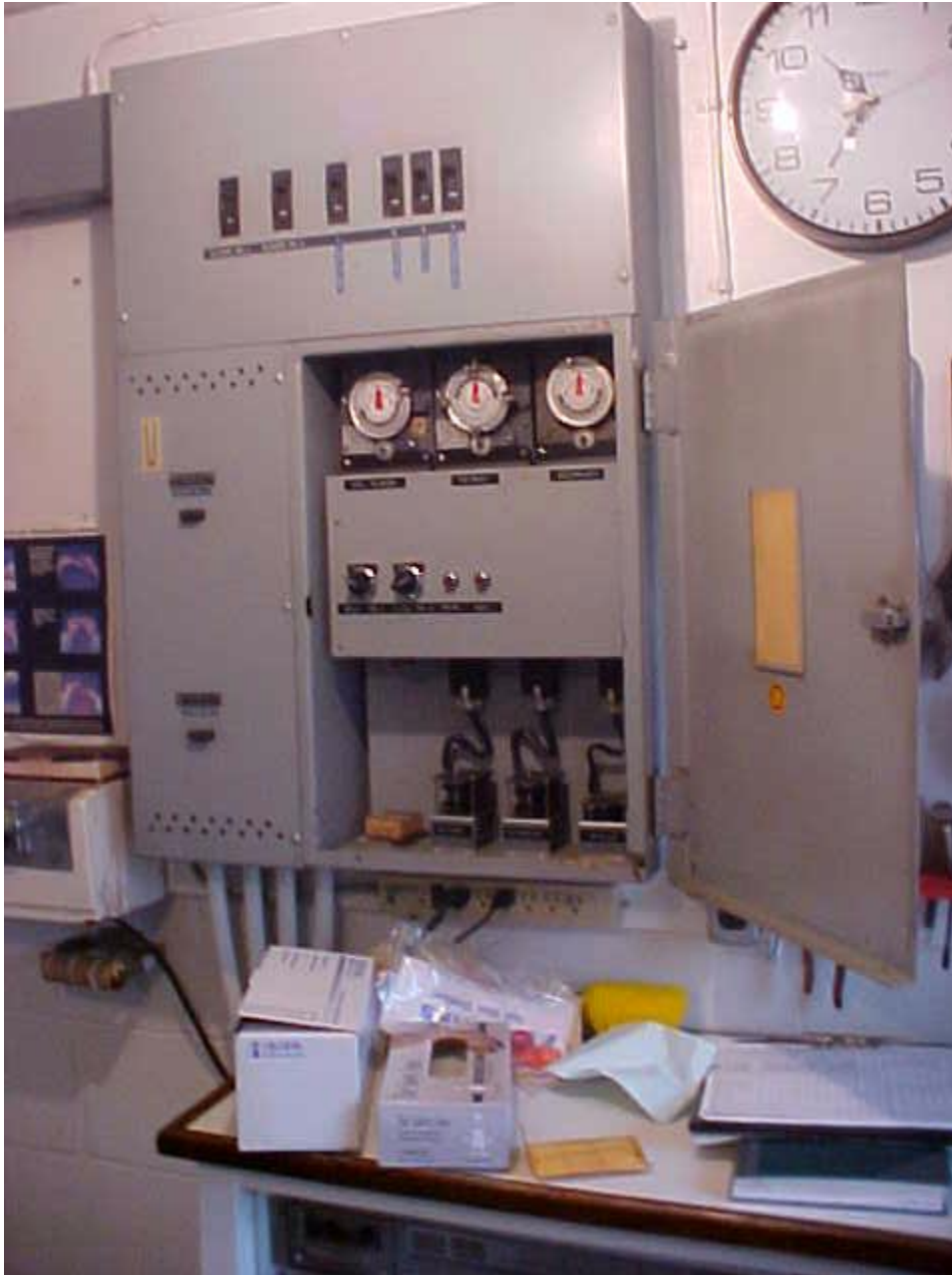
Control Panel for Plant – In Lab/Control Building
