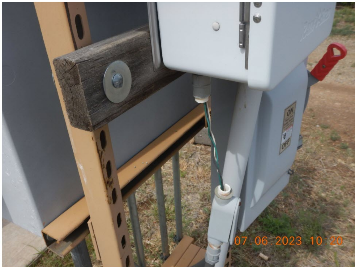
View of the Oshara Village WRF individual lift station electrical box. Note: the exposed wiring (no conduit). (DSCN2556) Photographed by D. Esparza
