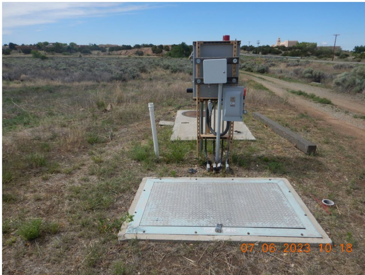
View of the Oshara Village WRF individual lift station located approximately 600-feet Northwest the WRF Facility. Note: the lack of perimeter fencing and the locked hatchway. (DSCN2552) Photographed by D. Esparza
