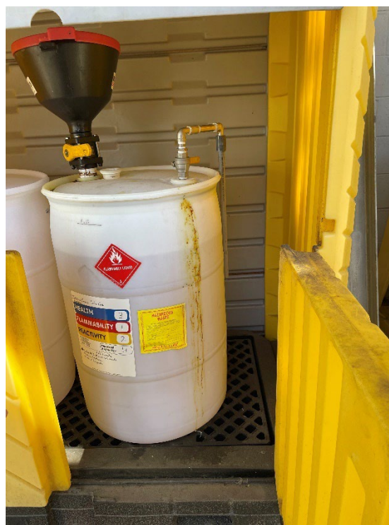
Figure 24: IMG_3267.jpg – Picture of the piping on the container
