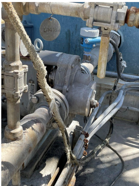
Figure 9: IMG_3252.jpg – Ancillary Equipment to T50
