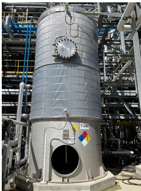
Figure 2: IMG_3245.jpg – Hazardous Waste Tank T-090
