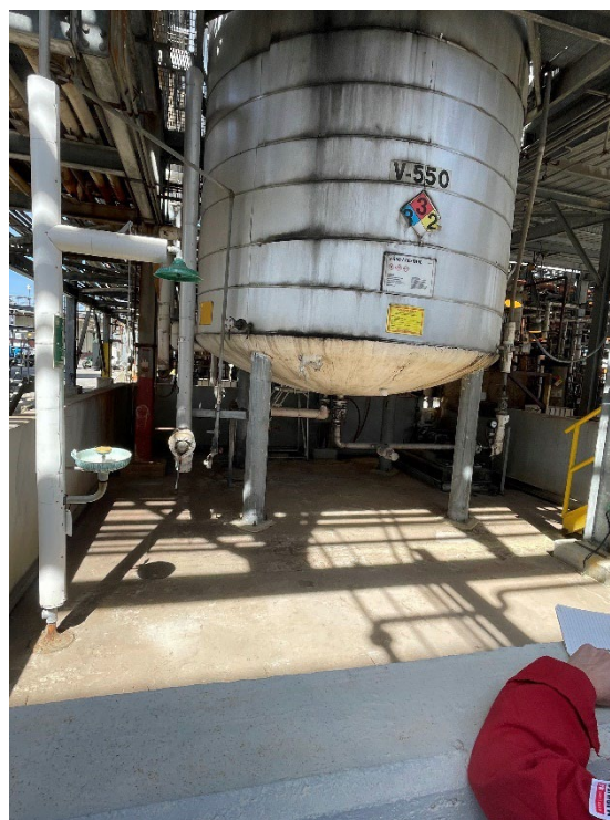
Figure 14: IMG_3257.jpg – Hazardous Waste Tank V-550
