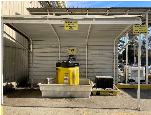
Figure 45: IMG_3287.jpg – Used oil tank
