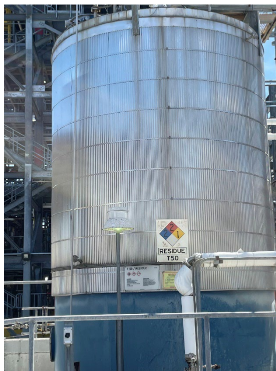
Figure 6: IMG_3249.jpg – Hazardous Waste Tank T50
