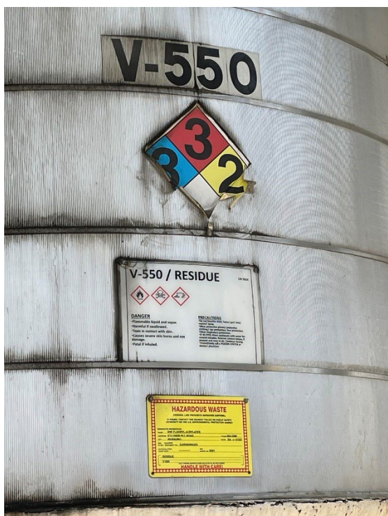
Figure 13: IMG_3256.jpg – Hazardous Waste Tank V-550
