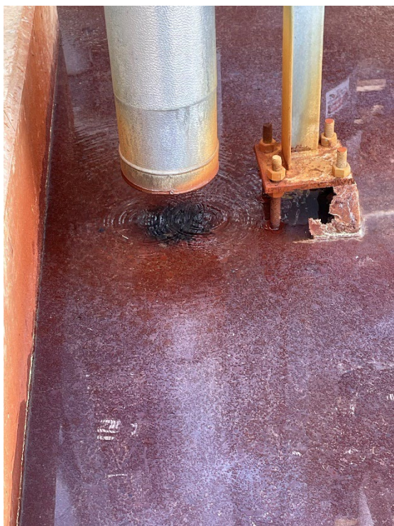
Figure 1: IMG_3244.jpg – Damage to secondary containment at T-345.
