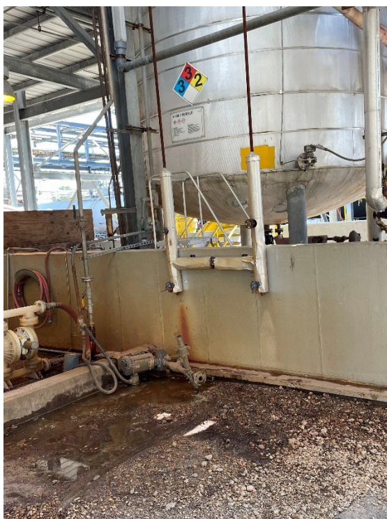
Figure 11: IMG_3254.jpg – Hazardous Waste Tank V-550
