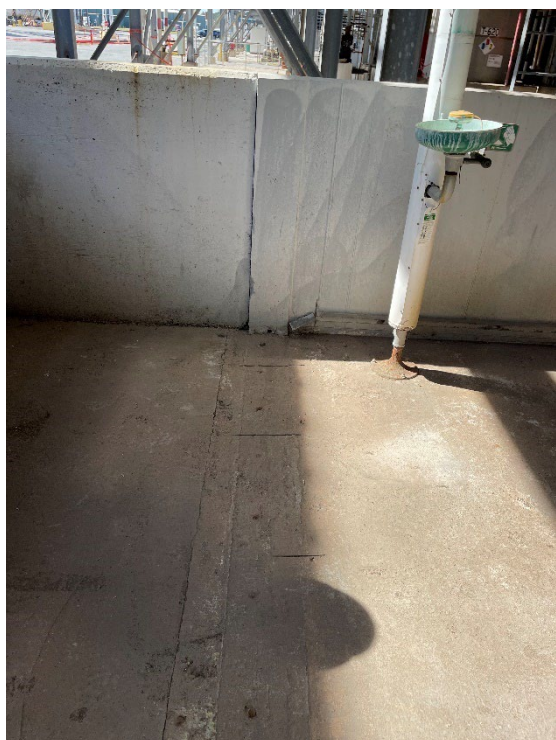
Figure 15: IMG_3258.jpg - V-550 secondary containment
