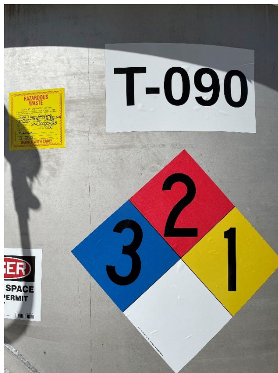
Figure 4: IMG_3247.jpg – Hazardous Waste Tank T-090
