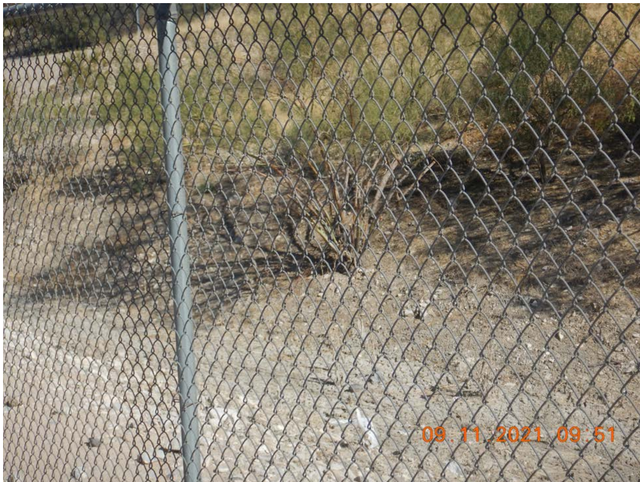
Additional view of earthen ditch along east side of wire fabric fencing. Note: stressed vegetation, staining and SSO debris. (DSCN2018) Photographed by D. Esparza
