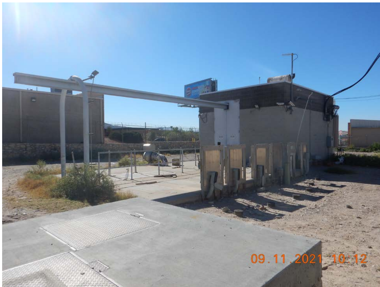
View of the Sunland Park Lift Station located west of the Doniphan Park Circle dual 30-inch force main failure. (DSCN2025). Photographed by D. Esparza
