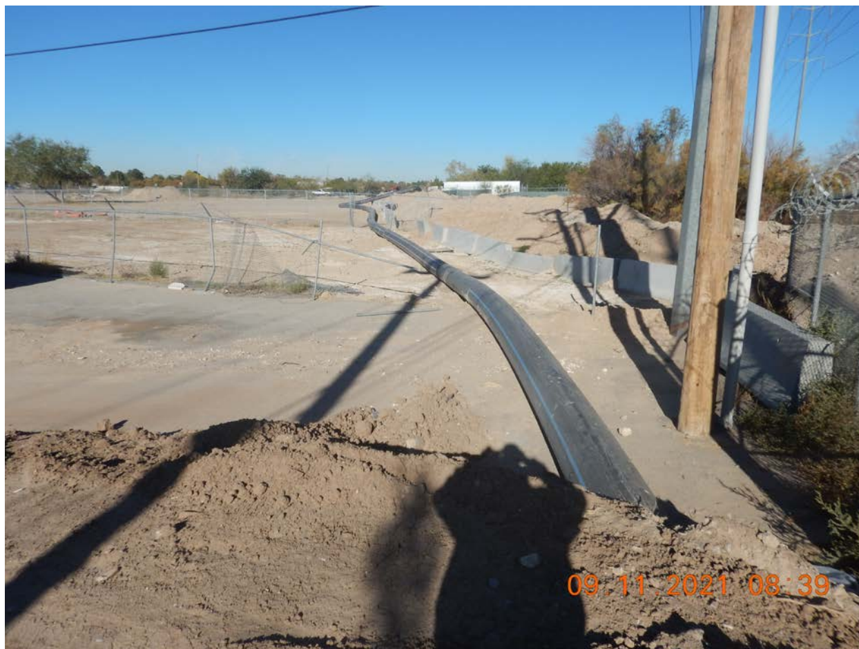
View of temporary above ground piping. (DSCN1998). Photographed by D. Esparza
