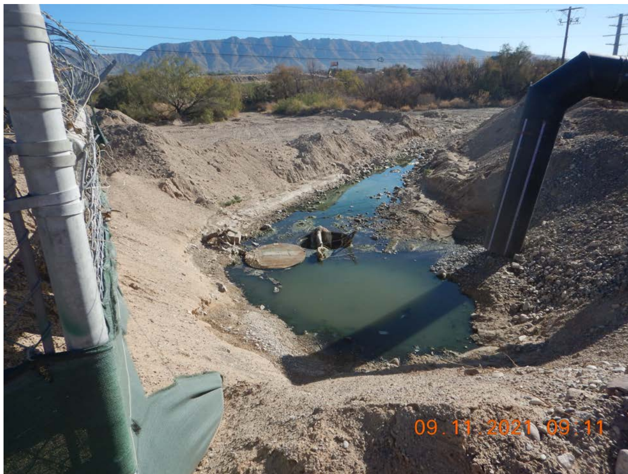
View of the temporary above ground piping (left side of photograph) and stormwater drop inlet. (DSCN2007). Photographed by D. Esparza
