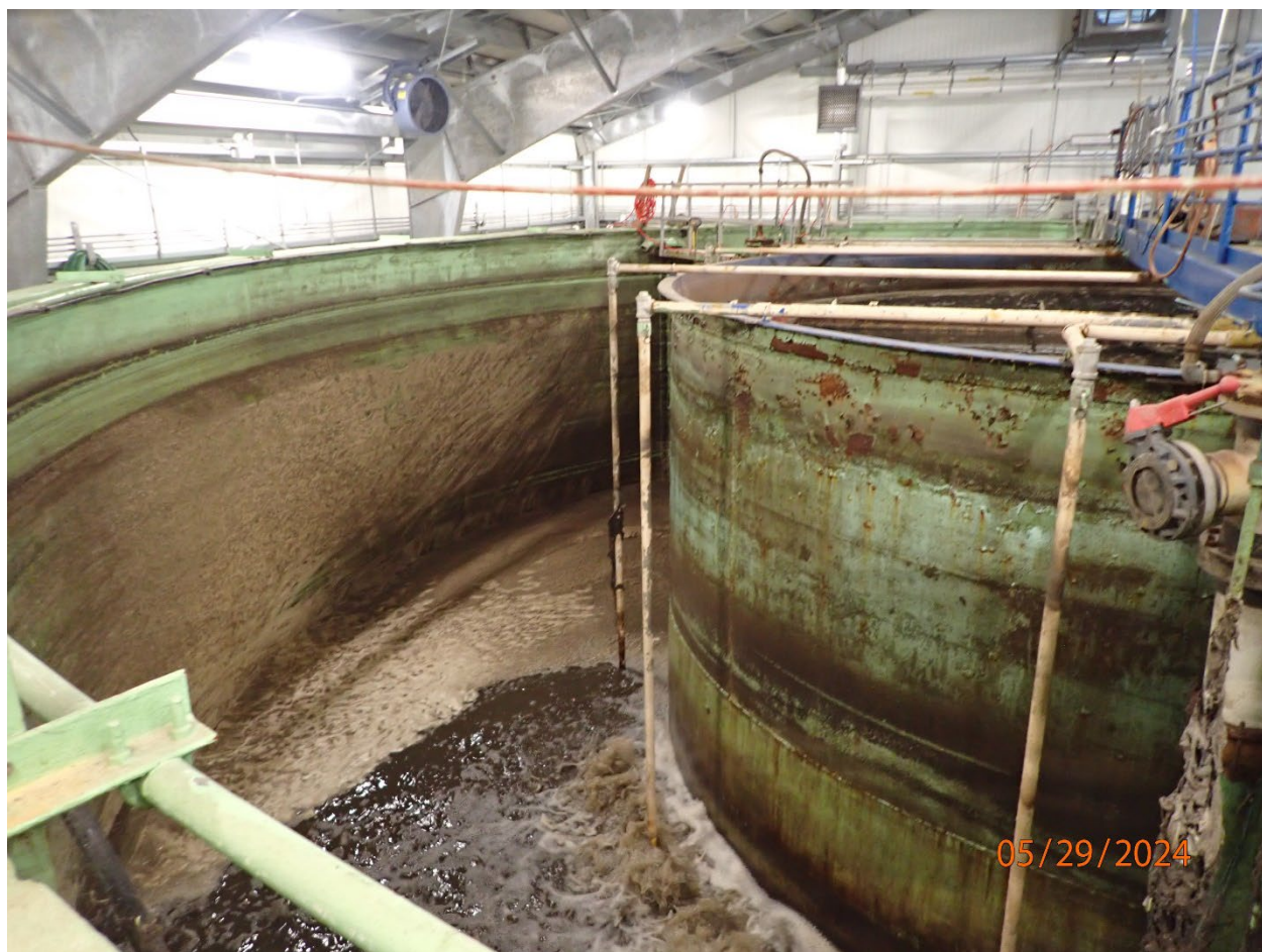
Photo 4 - Aerobic digester (right outside clarifier)
