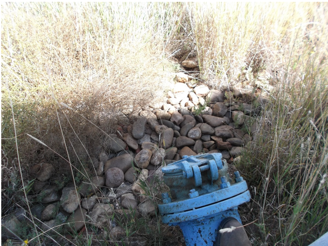
Photo 4. Grizzle Tank overflow valve.
