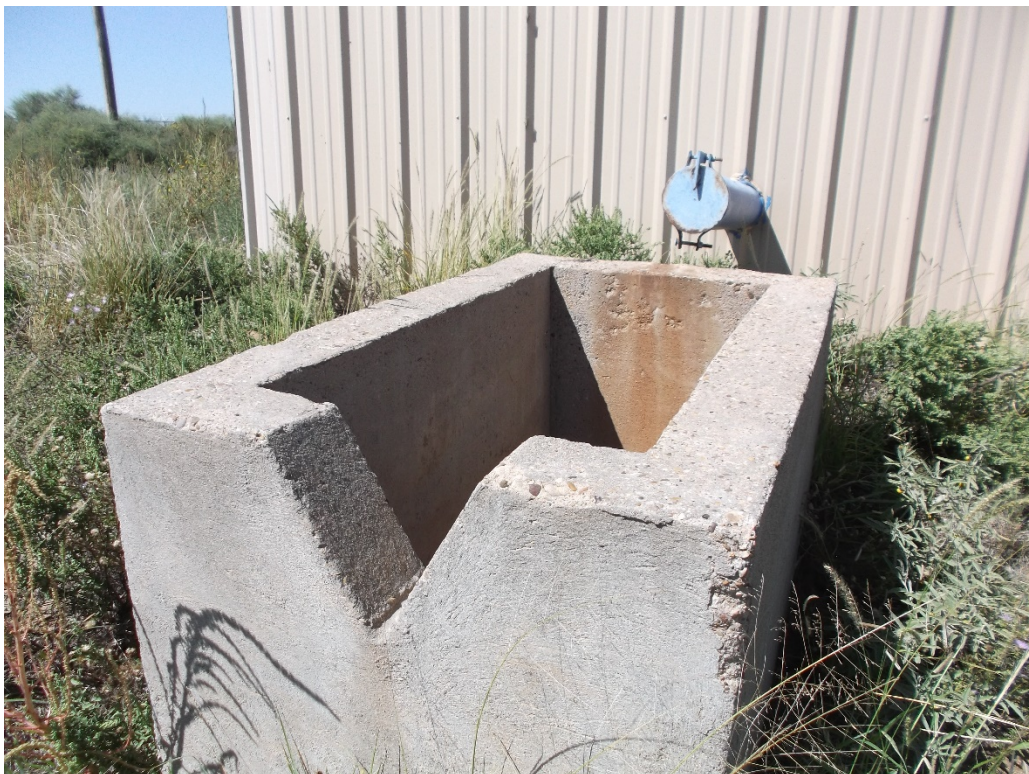
Photo #12. The flush line directly to the Grizzle well has no gasket or other protection for the flapper valve
