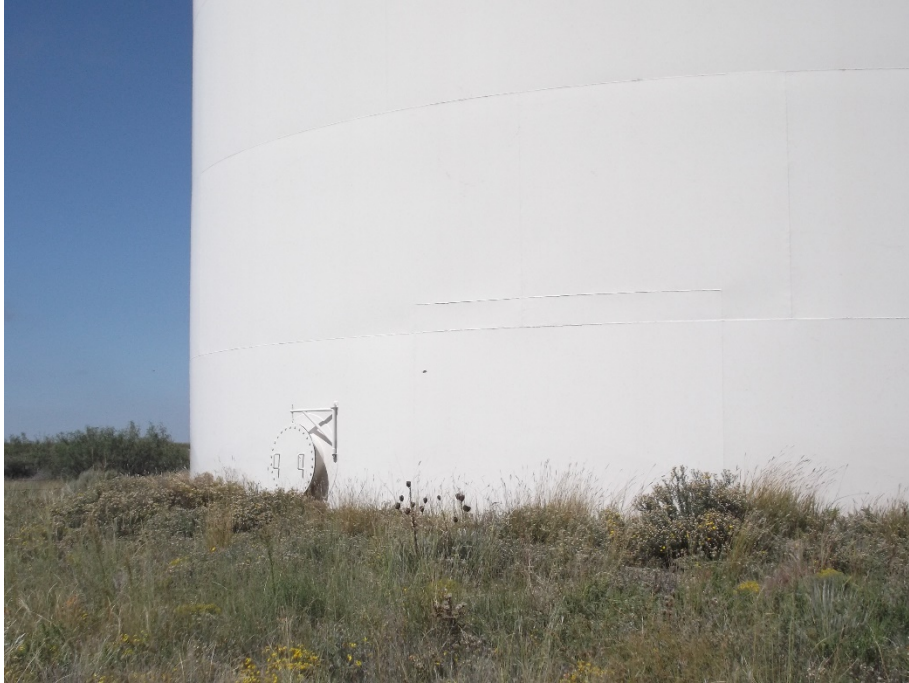
Photo 3. Grizzle Tank area overrun with vegetation, making it difficult (and potentially hazardous) to observe problems and perform maintenance
