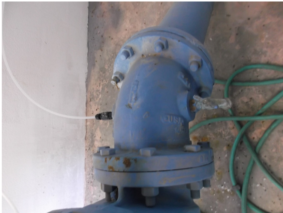
Photo #9. Raw water sample port in-line with the chlorine injection location.
