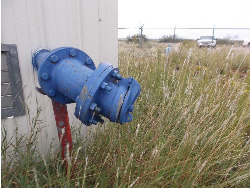
Photo 1: Overflow valve for Mac Well, not seating properly and vegetation not managed
