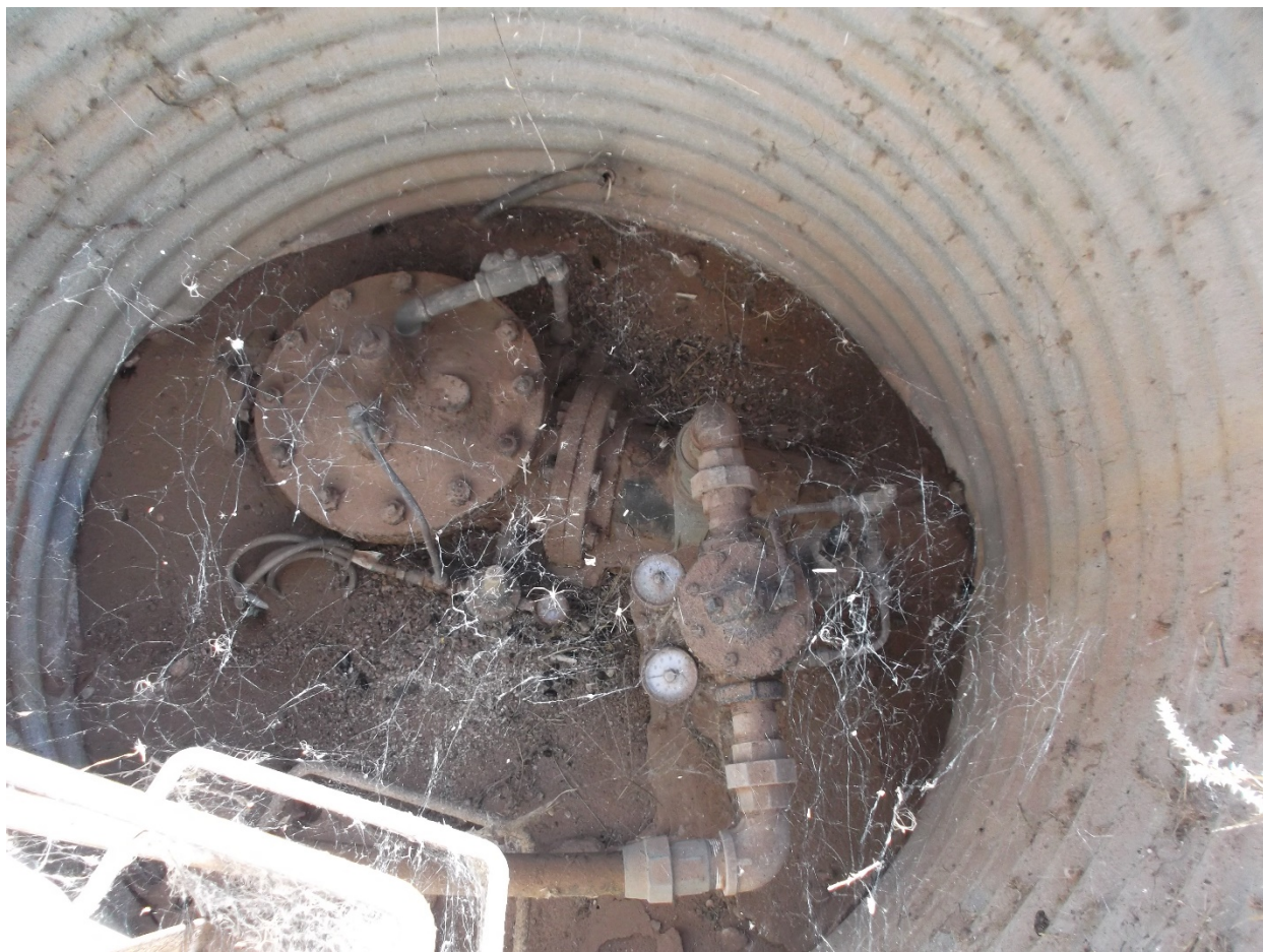
Photo #15. (1 of 2) Pressure Reducing Valves. Some corrosion, electrical open, subject to flooding, no vent.
