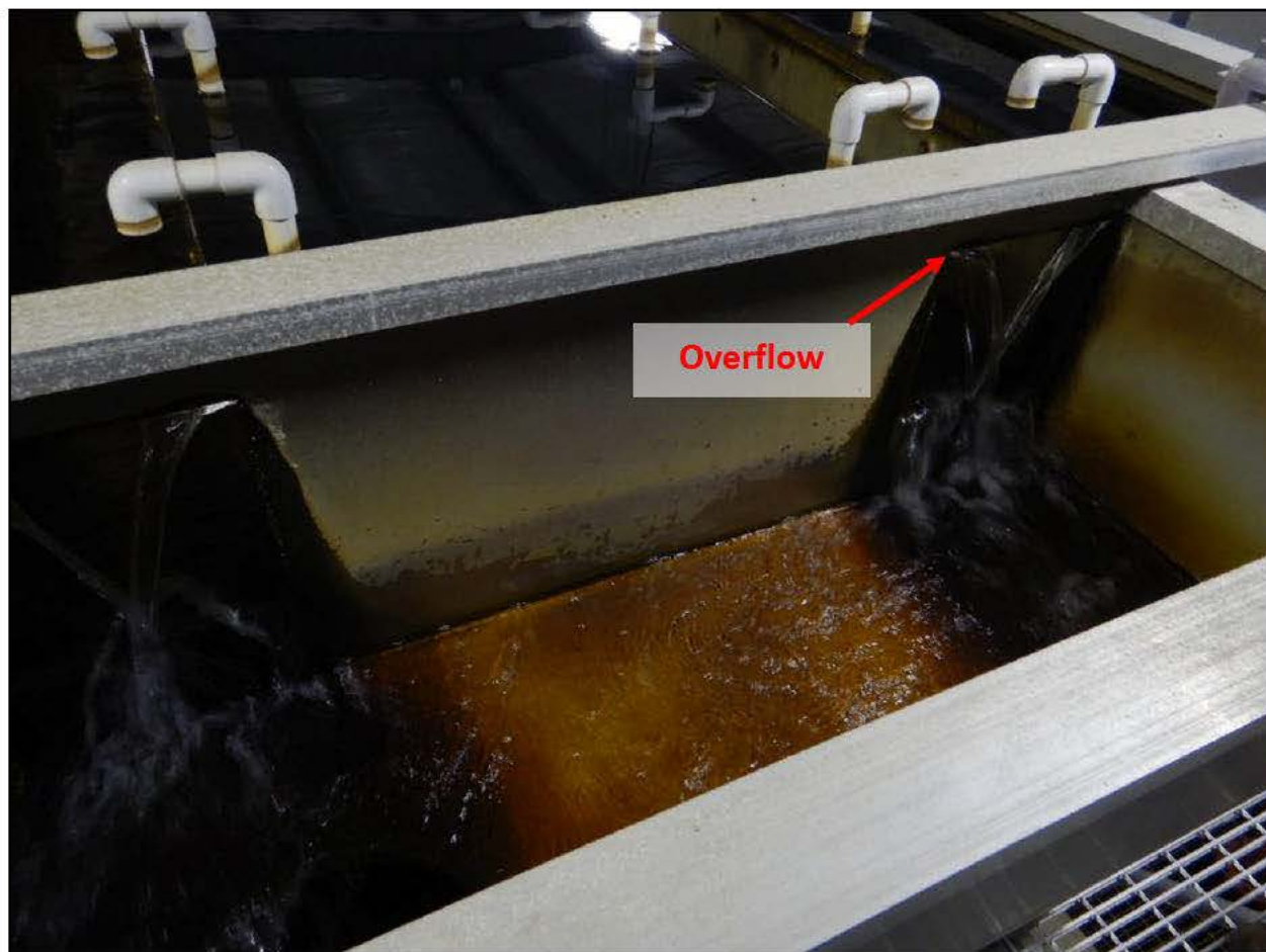
Photograph 16. Treatment Train #2 Tank, Hector WTP View of the water overflowing into the backwash basin due to a high water level in the tank.
