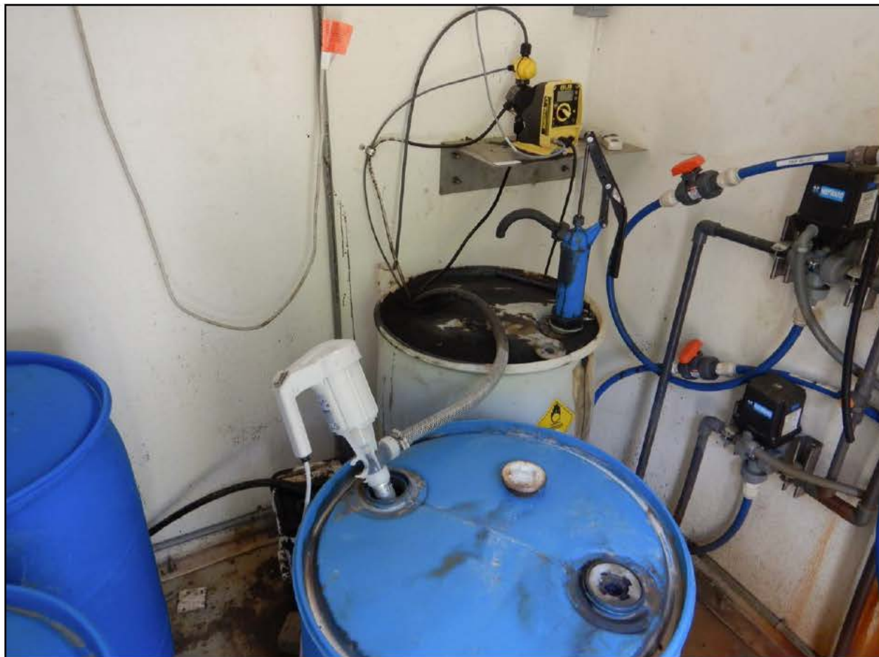
Photograph 12. Raw Water Chemical Feed Building, Hector WTP View of the inside of the raw water chemical feed building [REDACTED]
