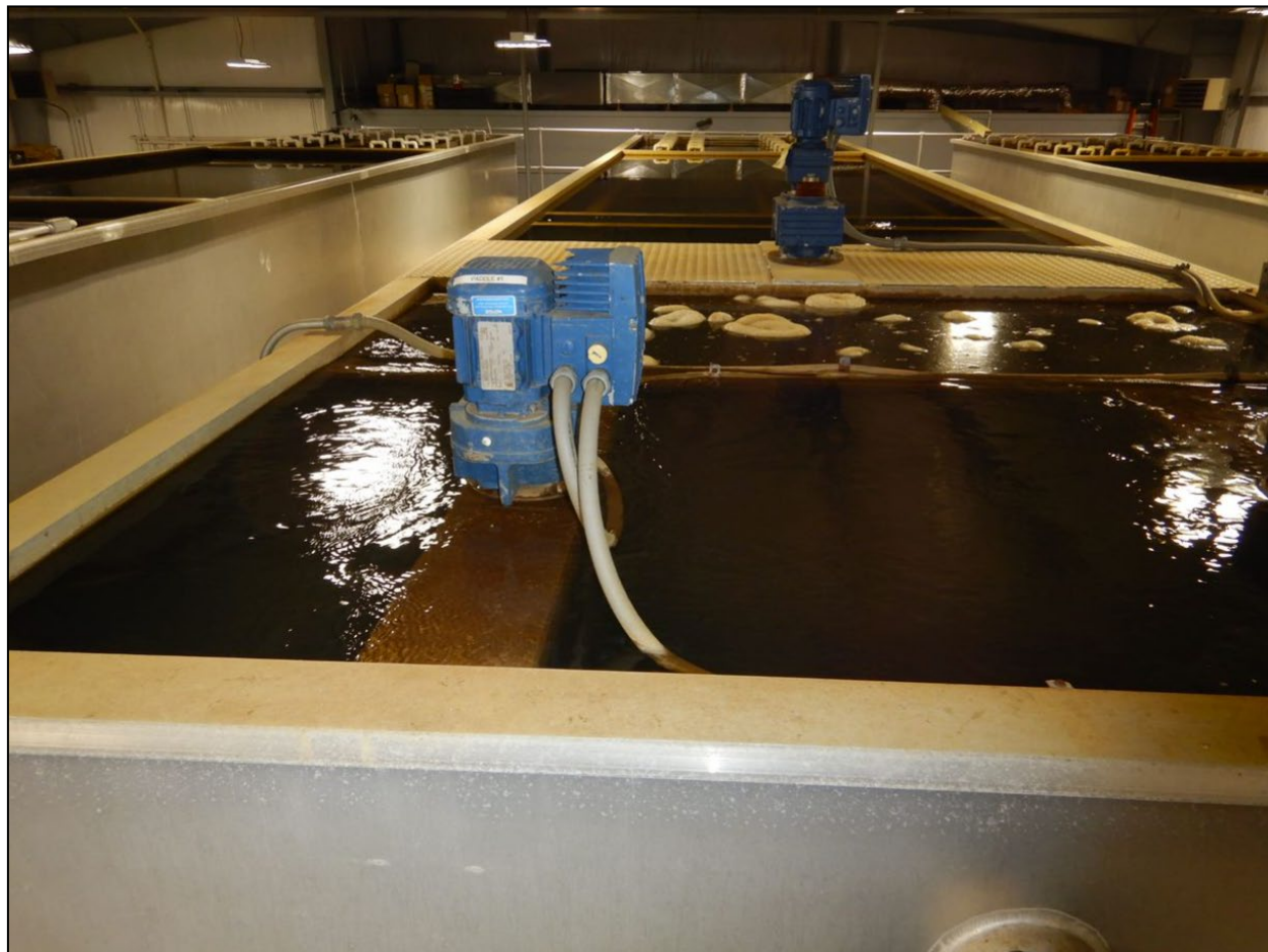
Photograph 15. Treatment Train #2 Tank, Hector WTP View of the Train #2 treatment tank at the Hector WTP. When the EPA Inspection Team arrived, the water level was approximately two inches below the edge of the tank. Once operators reset the level sensor, the water level lowered.
