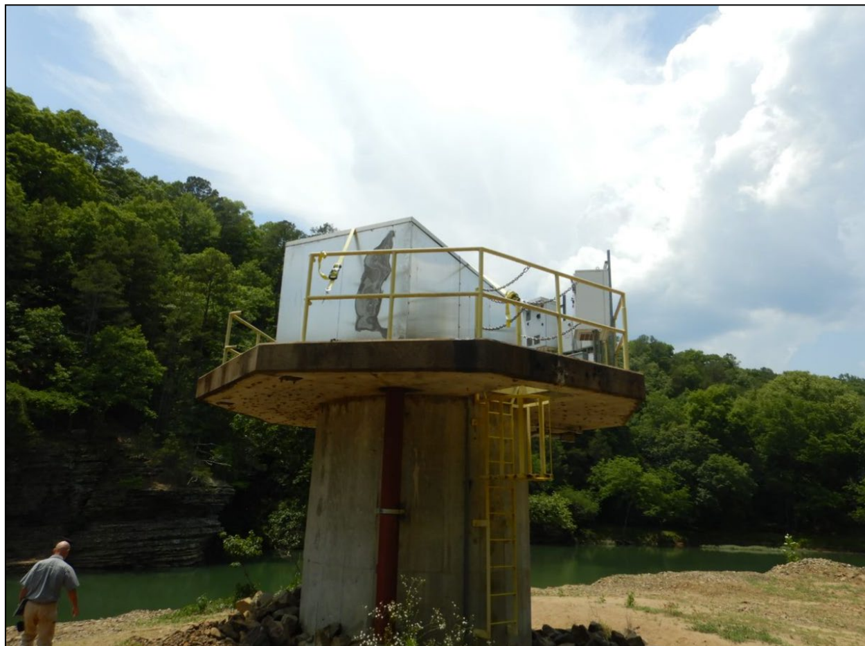
Photograph 10. Pump Structure, Hector WTP Intake View of the pump structure at the intake for the Hector WTP. The intake is located in the Illinois Bayou. Tri-County owns the land surrounding the intake, which is a protection barrier for the surface water quality and an extra layer of security for the water plant intake structure.
