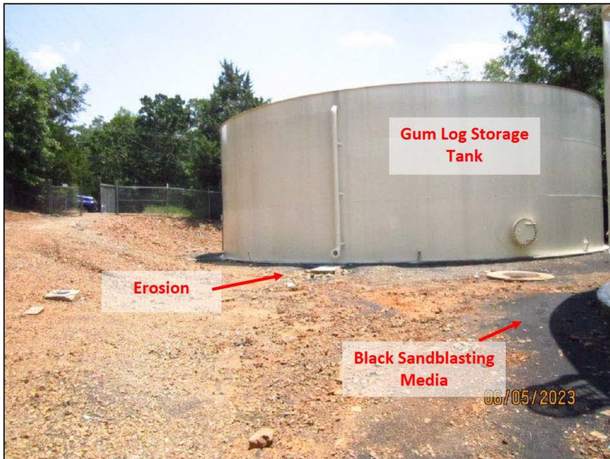
Photograph 4. Gum Log Storage Tank View of one of the two, 256,000-gallon Gum Log storage tanks. In this image, erosion can be seen beneath the overflow line, and black sandblasting media from the resurfacing of the tank can also be observed.
