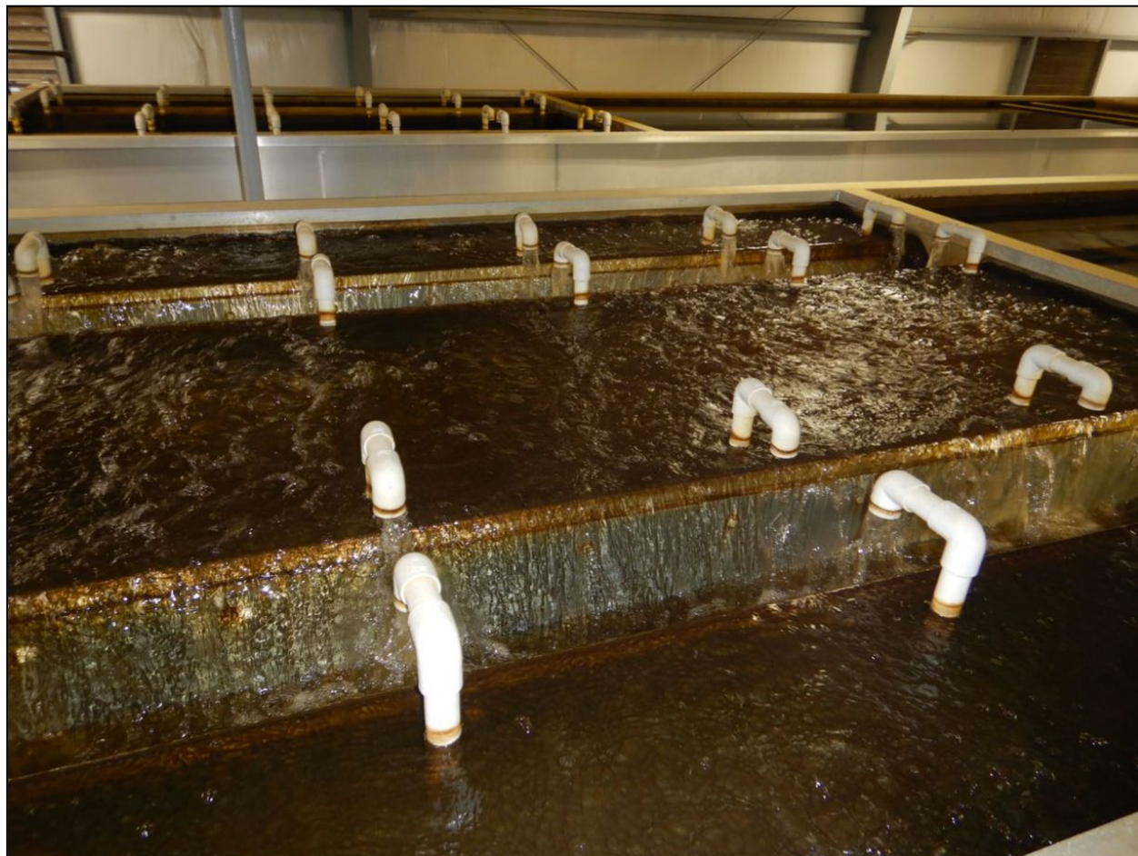
Photograph 17. Filter Backwash, Hector WTP View of the air scour that took place during the filter backwash in treatment Train #2.
