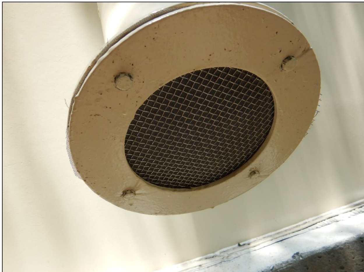
Photograph 7. Overflow Line, Gum Log Storage Tank View the end of the overflow line at one of the Gum Log Storage Tanks. The opening was covered by a 24-inch mesh screen, as well as an additional coarse screen. The second tank contained an overflow line and a screen that was similar to this one.
