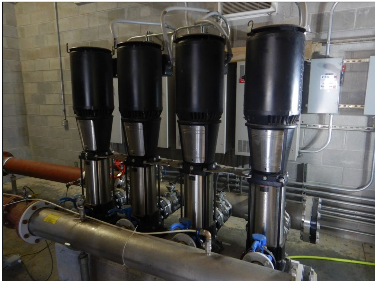
Photograph 20. High Service Pump Station, Hector WTP View of the four VFD pumps at the HS Pump Station. This pump station delivers finished water to the distribution system following treatment at the Hector WTP.
