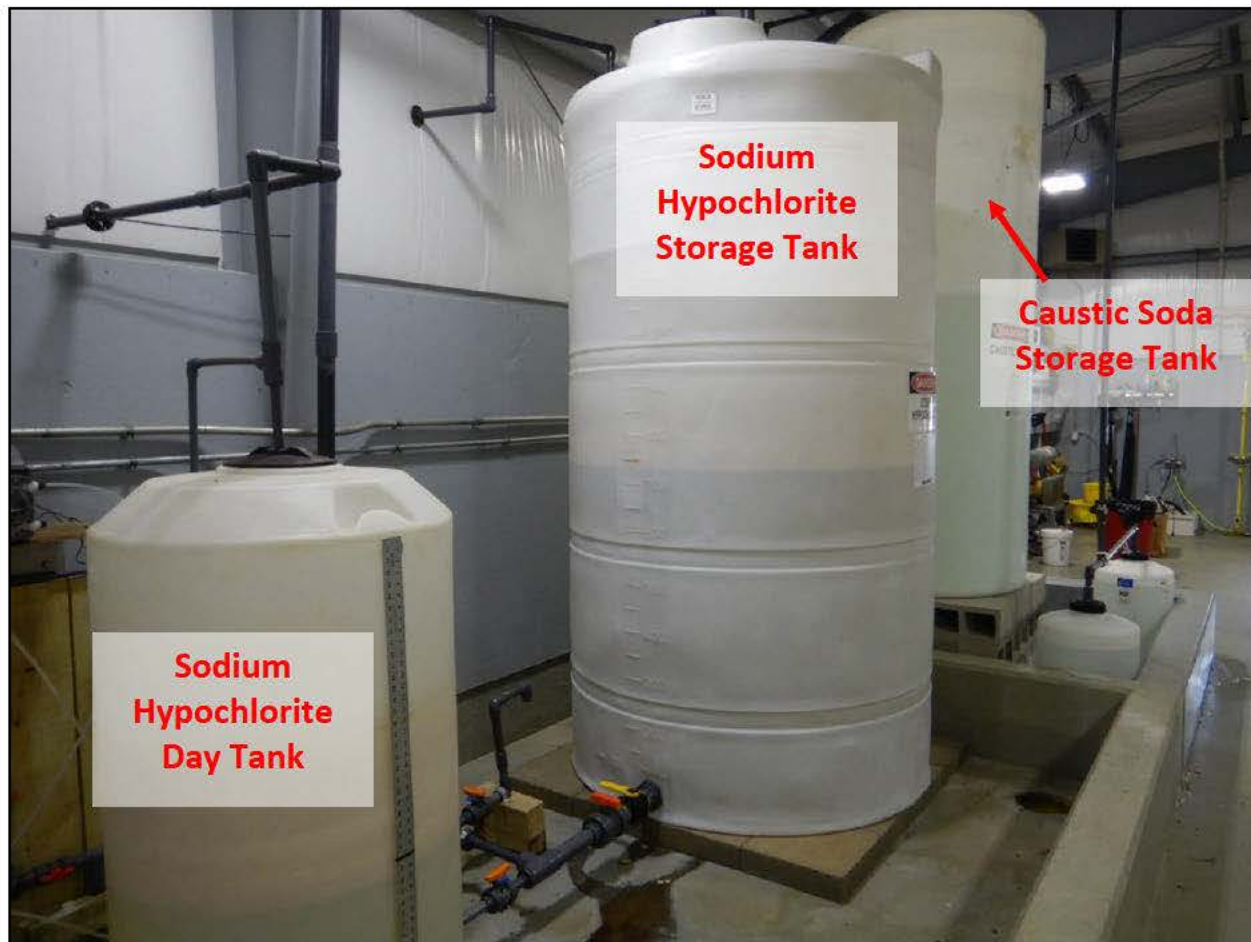
Photograph 14. Sodium Hypochlorite and Caustic Soda Storage Tanks, [REDACTED] View of the sodium hypochlorite and caustic soda storage tanks and the sodium hypochlorite day tank [REDACTED]
