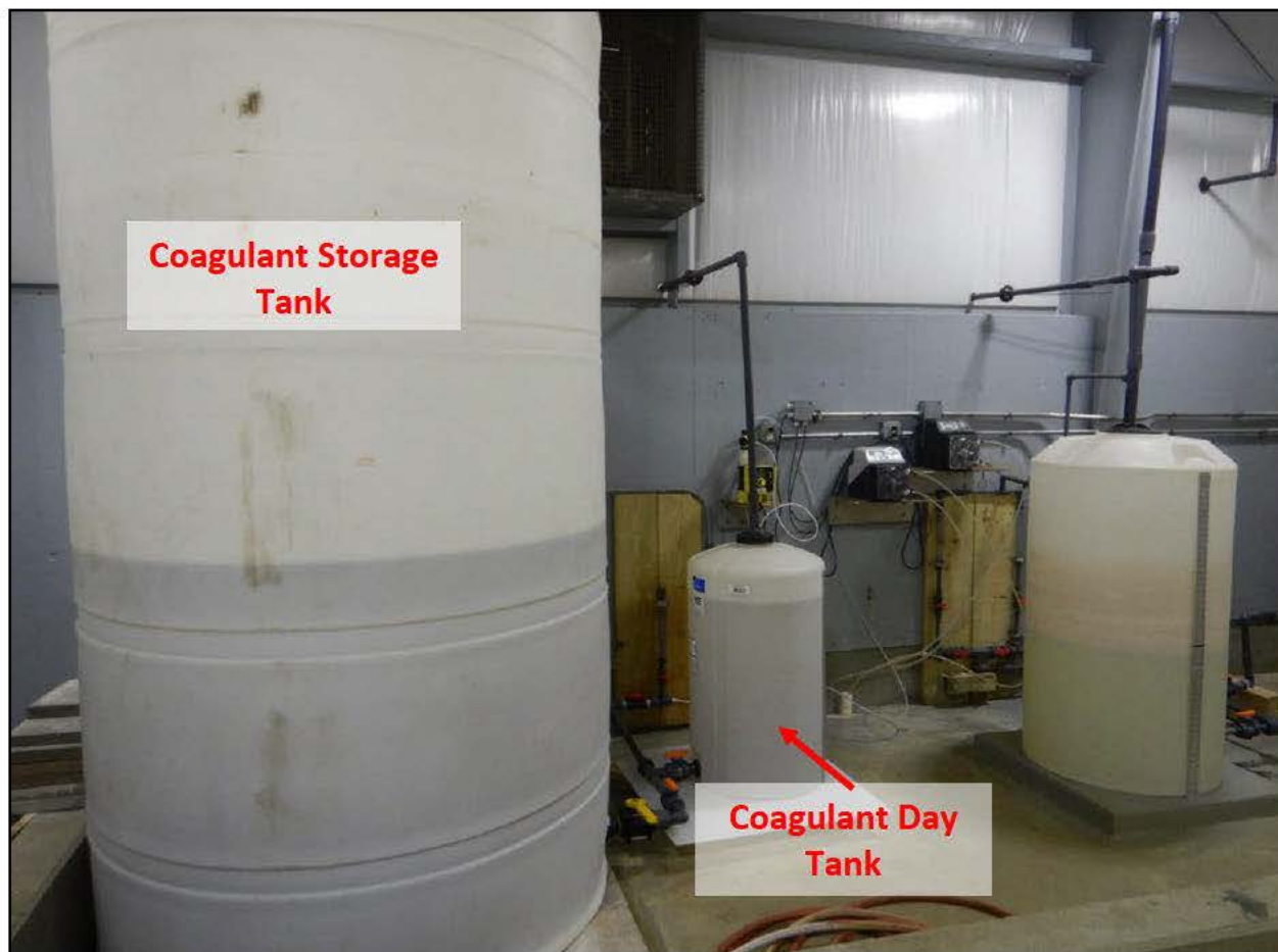
Photograph 13. Coagulant Tank, [REDACTED] View of the Coagulant storage and day tanks [REDACTED] [REDACTED] The coagulant tank did not have a label when the EPA Inspection Team arrived onsite, but a label was placed on the tank once operators became aware of this.
