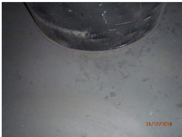
Picture 24 – Robovent Baghouse dust release to floor
