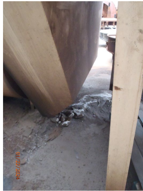
Picture 3 – Internal Blast Booth SAA –baghouse dust released to the ground
