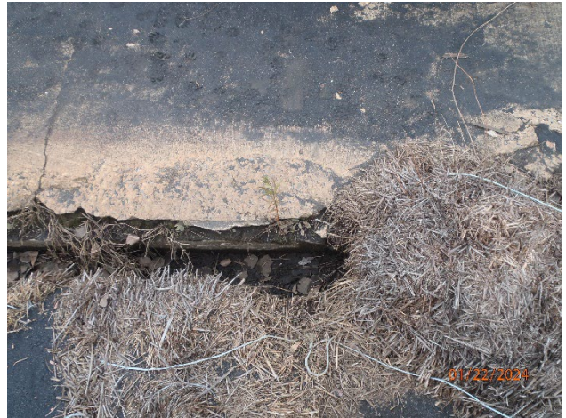
Picture 9 – External Blast Media – non-hazardous black beauty media released to storm water drain
