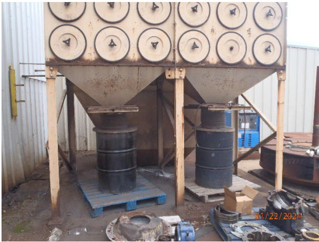
Picture 1 – Internal Blast Booth SAA drums not labeled
