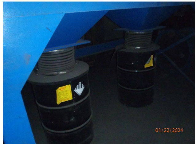
Picture 21 – Robovent Baghouse SAA drums
