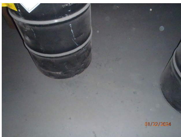
Picture 23 – Robovent Baghouse dust release to floor
