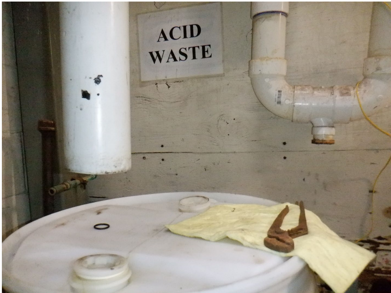
(Figure 12: Showing corrosion of the piping system above)
