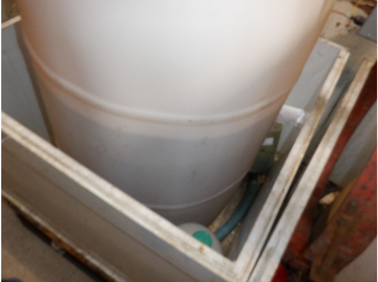
(Figure 14: Showing hazardous waste located inside the secondary containers with no label and date)
