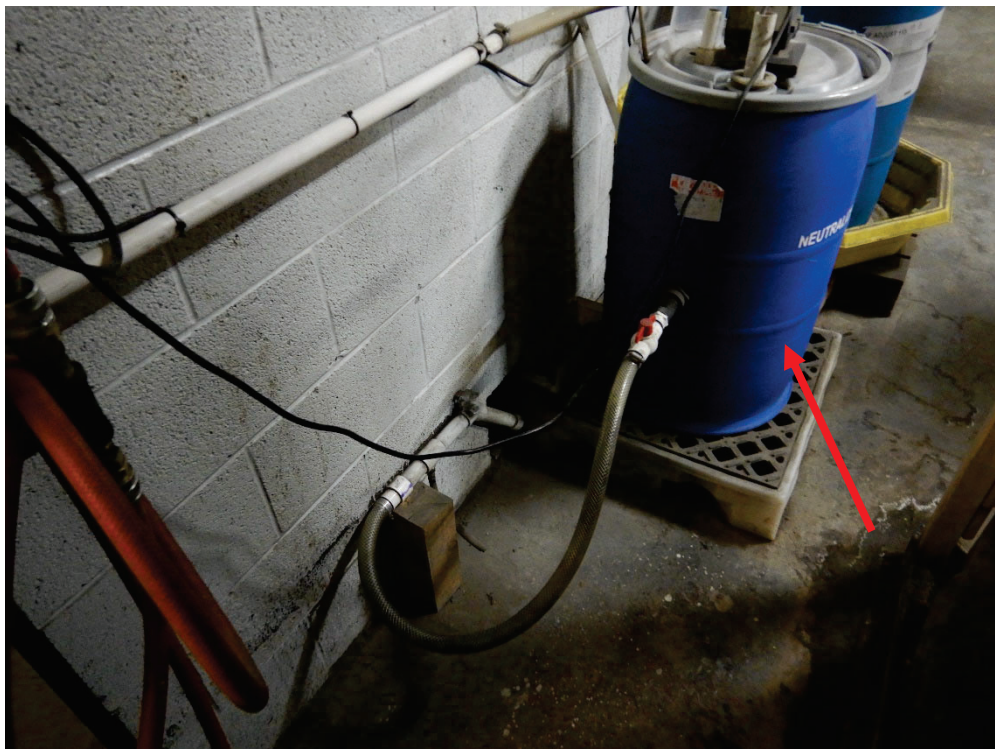
Photograph 4: Another view of the final discharge tank. Wastewater gravity flows from the tank through the hose identified by the red arrow.
