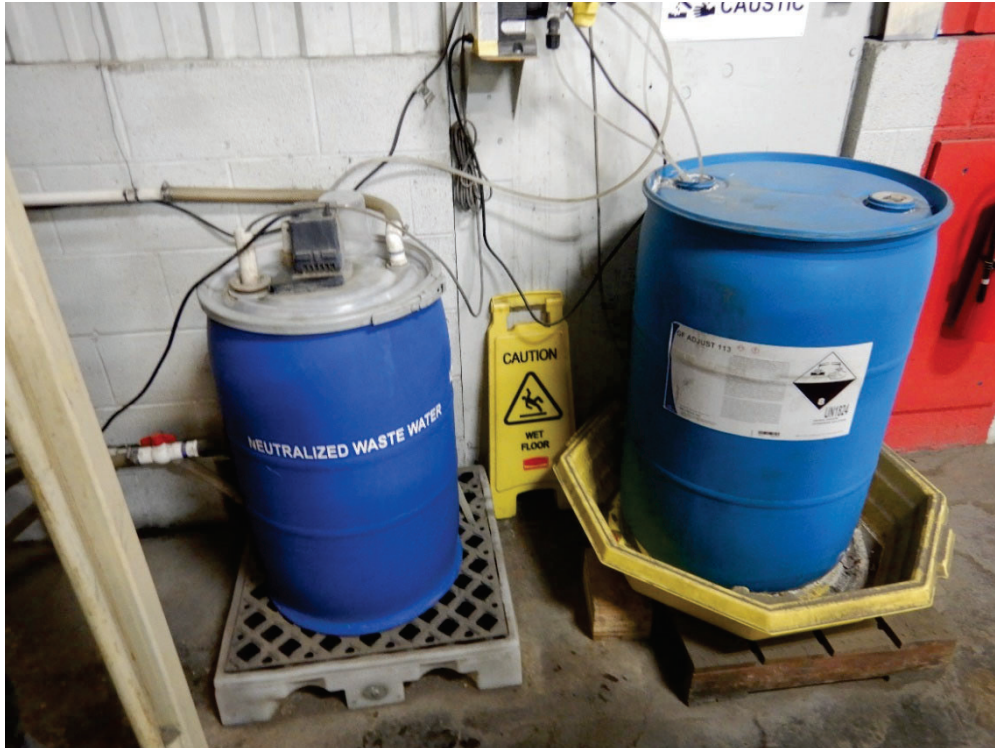
Photograph 3: The final discharge tank used for pH neutralization is on the left side of the photo. The drum at the right side of the photo is the sodium hydroxide, the pH adjustment chemical.
