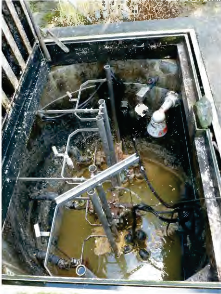
Photo 1 / P1000650 – Lift Station
