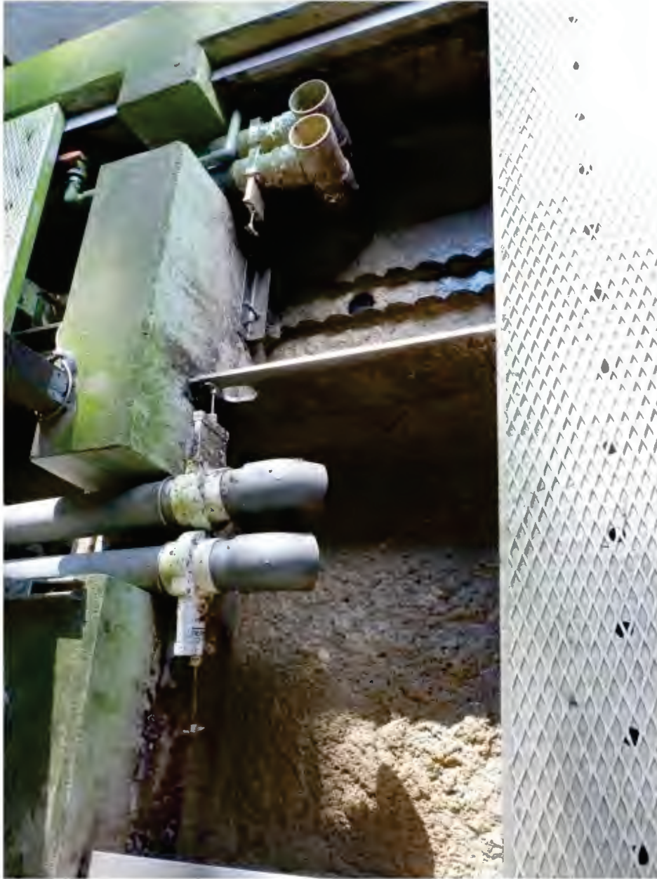
Photo 4 / P1000651 – Sludge Tank
