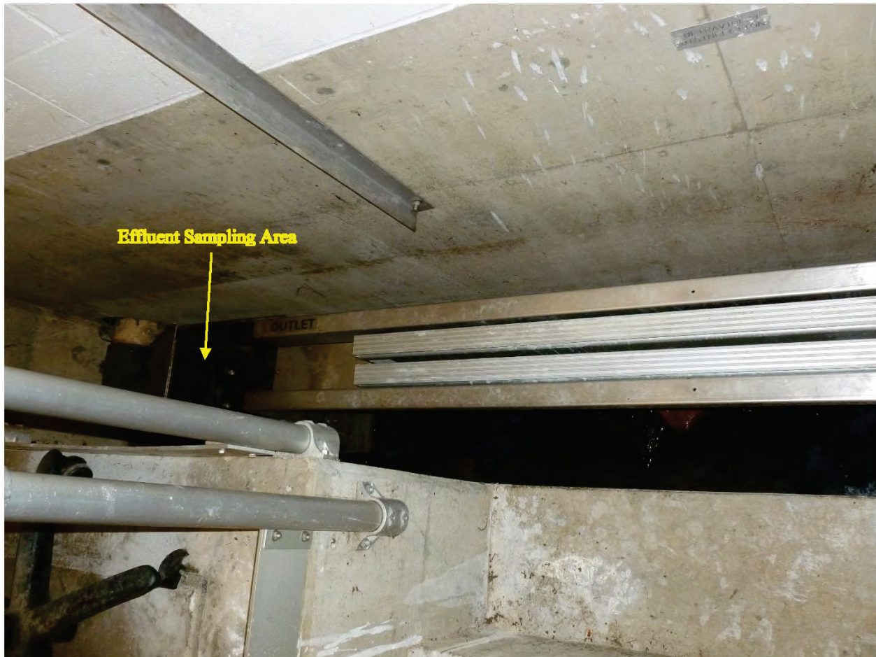
Photo 6 / P1000658 – UV Disinfection, Outlet Side
