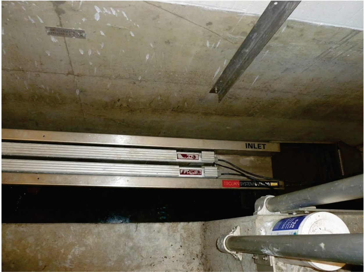
Photo 7 / P1000657 – UV Disinfection, Inlet Side
