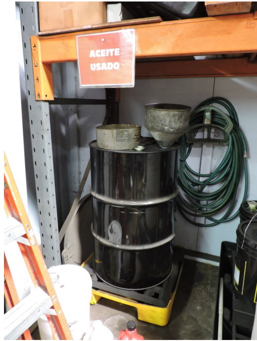
Picture 5— Mechanical Shop Area—Here, a 55-gallon black steel container was observed above a secondary containment. At the time of the inspection, the container was not labeled as used oil.
