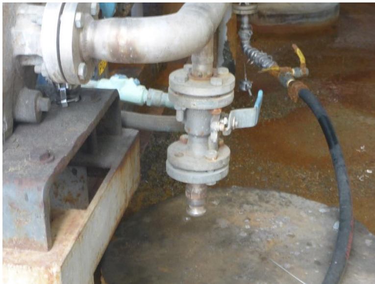
Photo 23: Missing bolt on a connection of ancillary equipment associated with the distillation system at T9-A.
