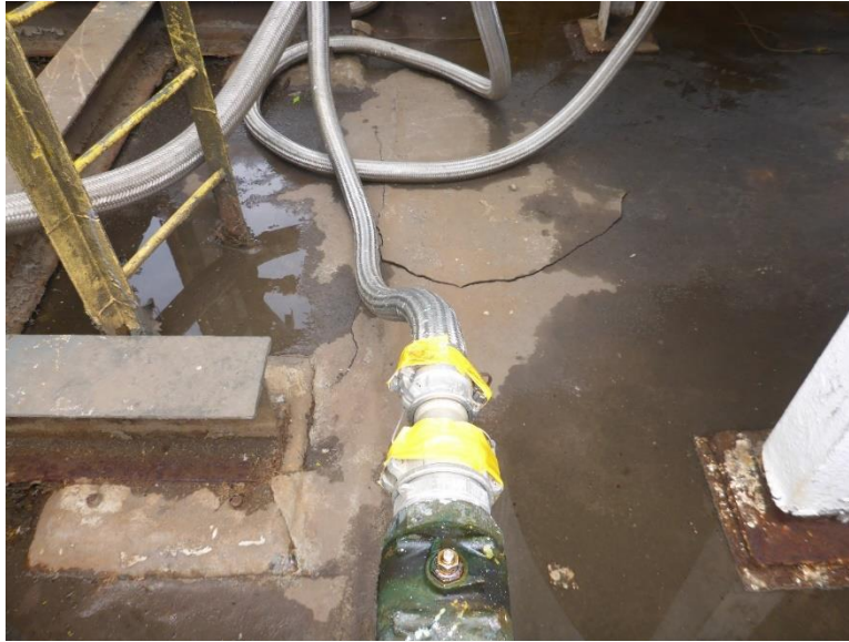
Photo 21: Liquid at the connection identified with tag number 583.
