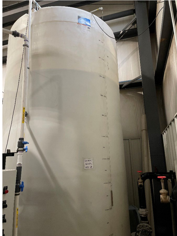
Photo #1. Pretreated process wastewater is stored in the aerated storage tank.
