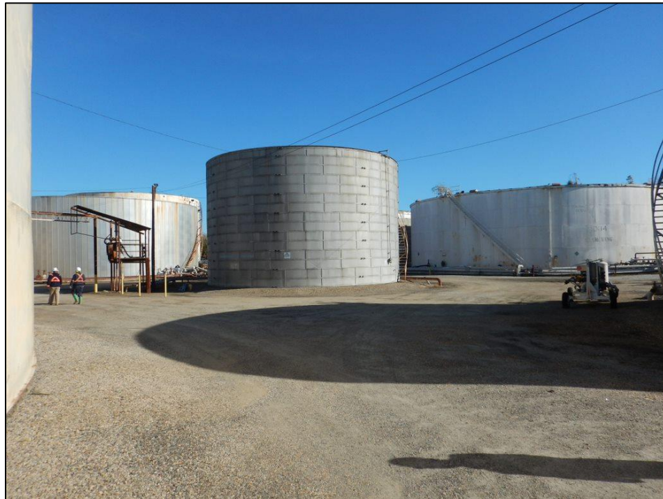
Photograph 6. (DSCN2204) View, facing north, of the Facility's aboveground storage tank (AST) farm (hereafter, tank farm) in the northern portion of the Facility. At the time of the inspection, the Facility was currently only utilizing one tank (Tank 5008) to store sodium hydroxide (caustic soda). The other ten (10) ASTs onsite were classified as out of service.
