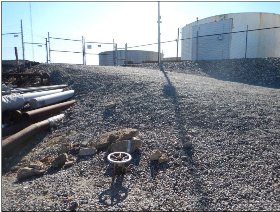
Photograph 11. (DSCN2217) View, facing south, of the manual valve for Outfall 001. Note the tank farm in the background.
