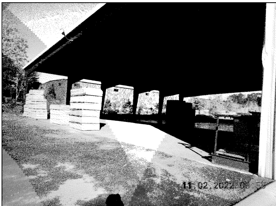
Photograph 10. View, facing northwest, of the drip pad outside the southwest corner of the treatment plant. Raw lumber is stored on the drip pad but not under the roof.
