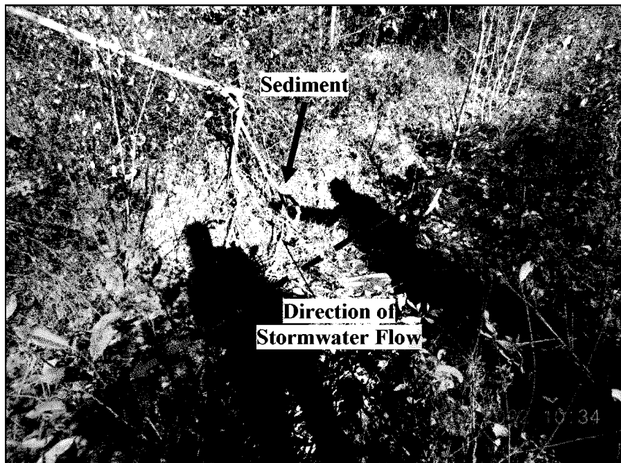
Photograph 22. View, facing northwest, of the trench along the west perimeter. The Facility representative stated stormwater flows along the trench to Outfall 003. The EPA Inspection Team observed sediment in the trench.
