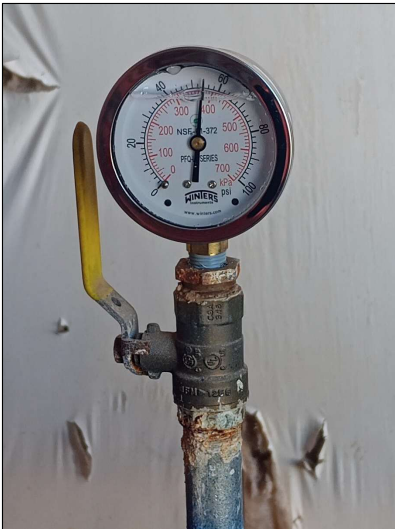
Photograph 20. Booster Station 919 Gauge 1 fix.jpeg
