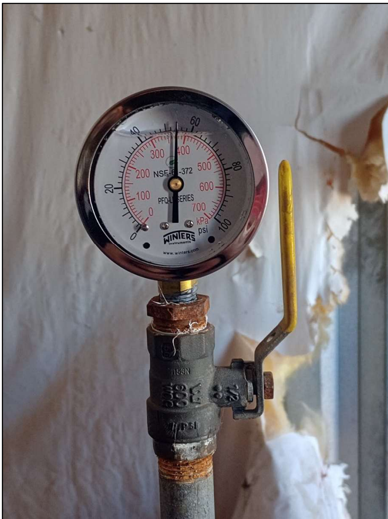
Photograph 21. Booster Station 919 Gauge 2 fix.jpeg
