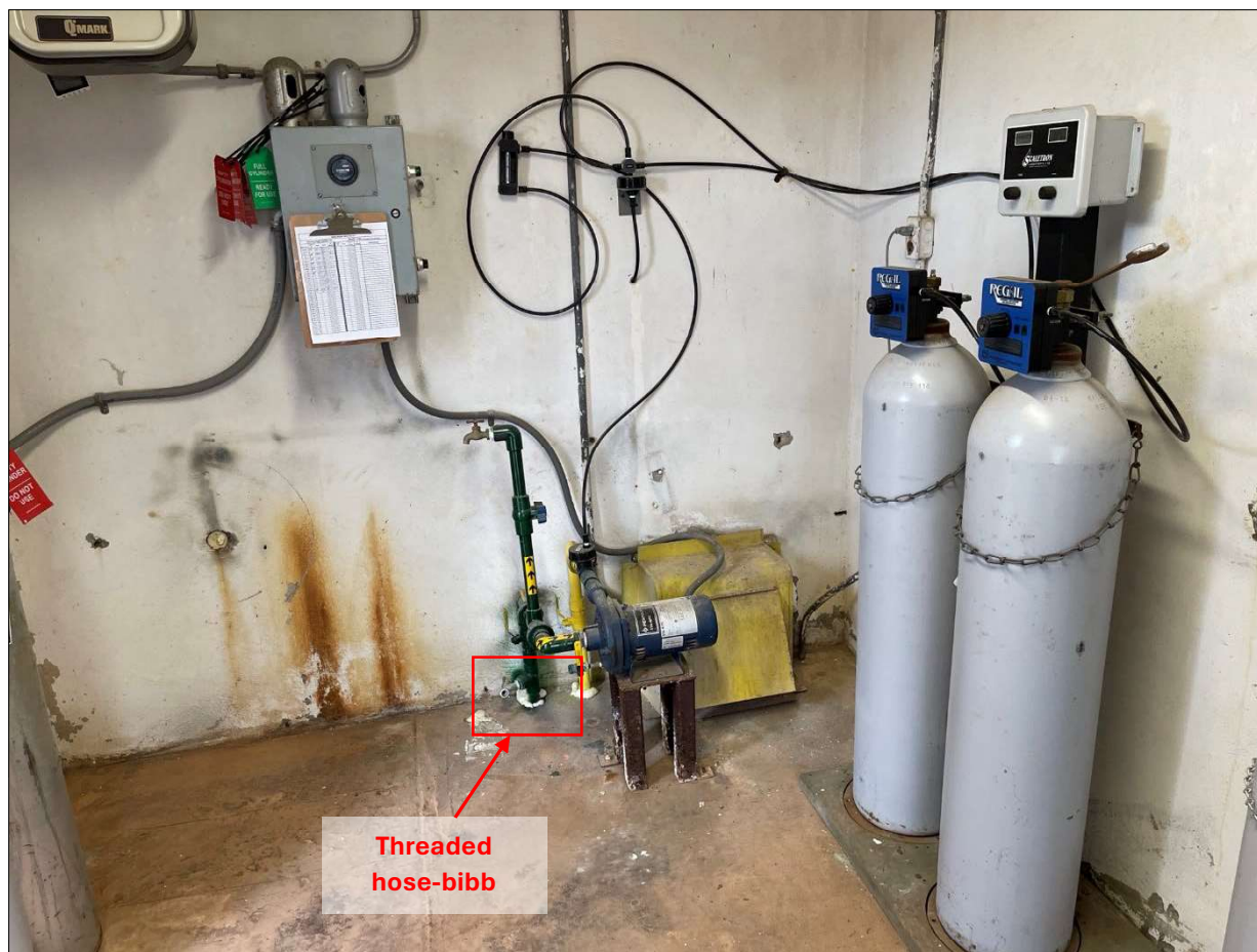
Photograph 2. Chlorination Station 774 IMG_3121.jpeg
