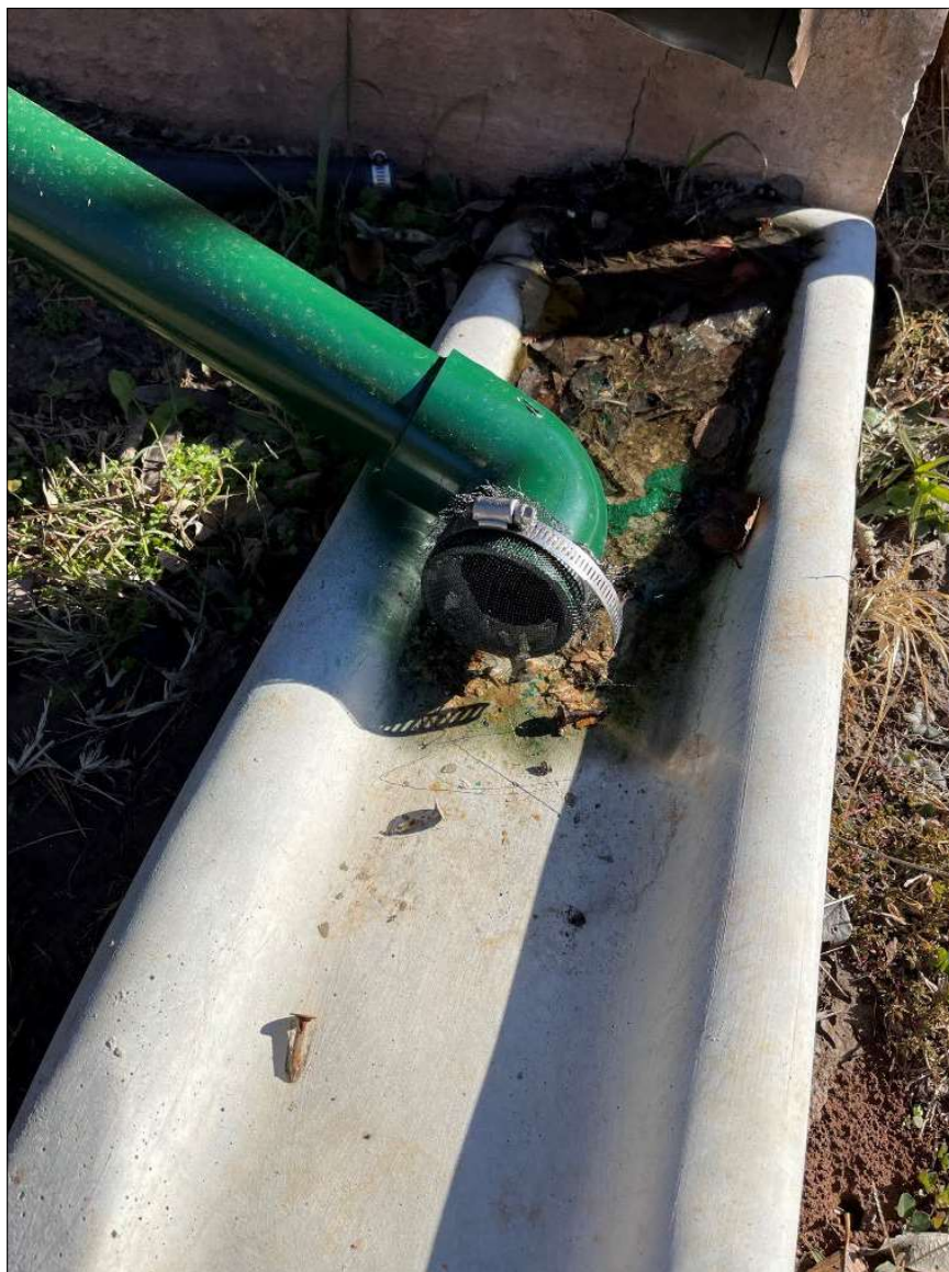
Photograph 10. Well 25 Building 3802 IMG_3166.jpeg
