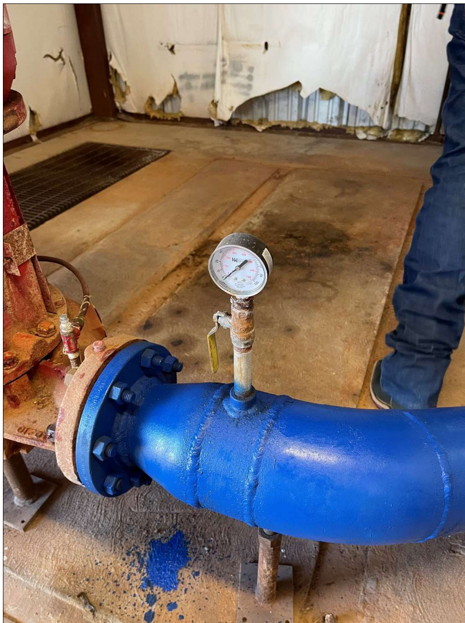
Photograph 18. Booster Station 919 IMG_3158.jpeg
