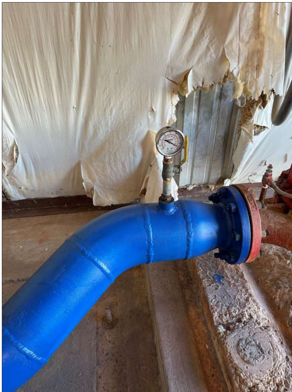
Photograph 19. Booster Station 919 IMG_3161.jpeg
