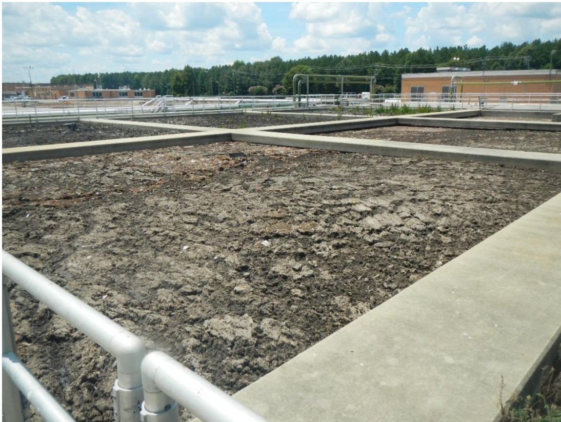
Photo 6: Seven non-operational clarifiers were observed with solids buildup.
