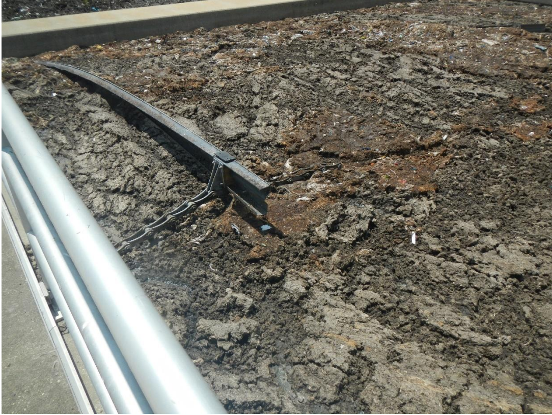
Photo 7: Damaged chain and paddle on primary clarifier.
