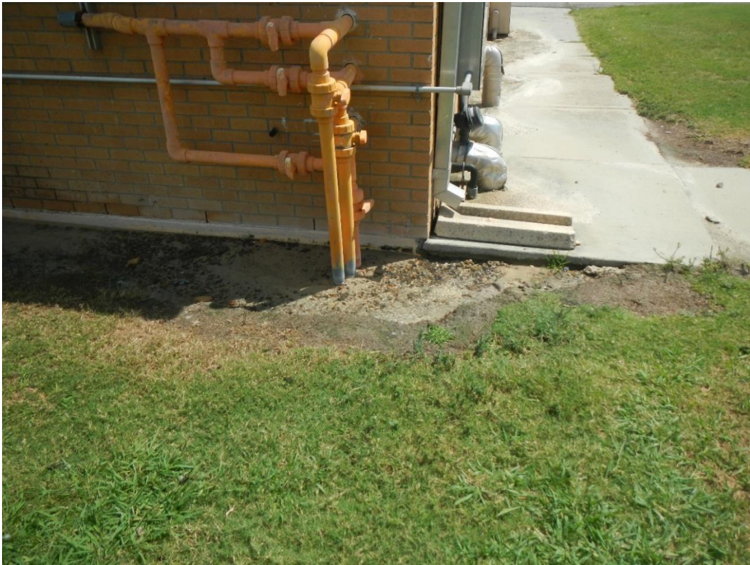
Photo 13: Location of drinking water leak under concrete slab
