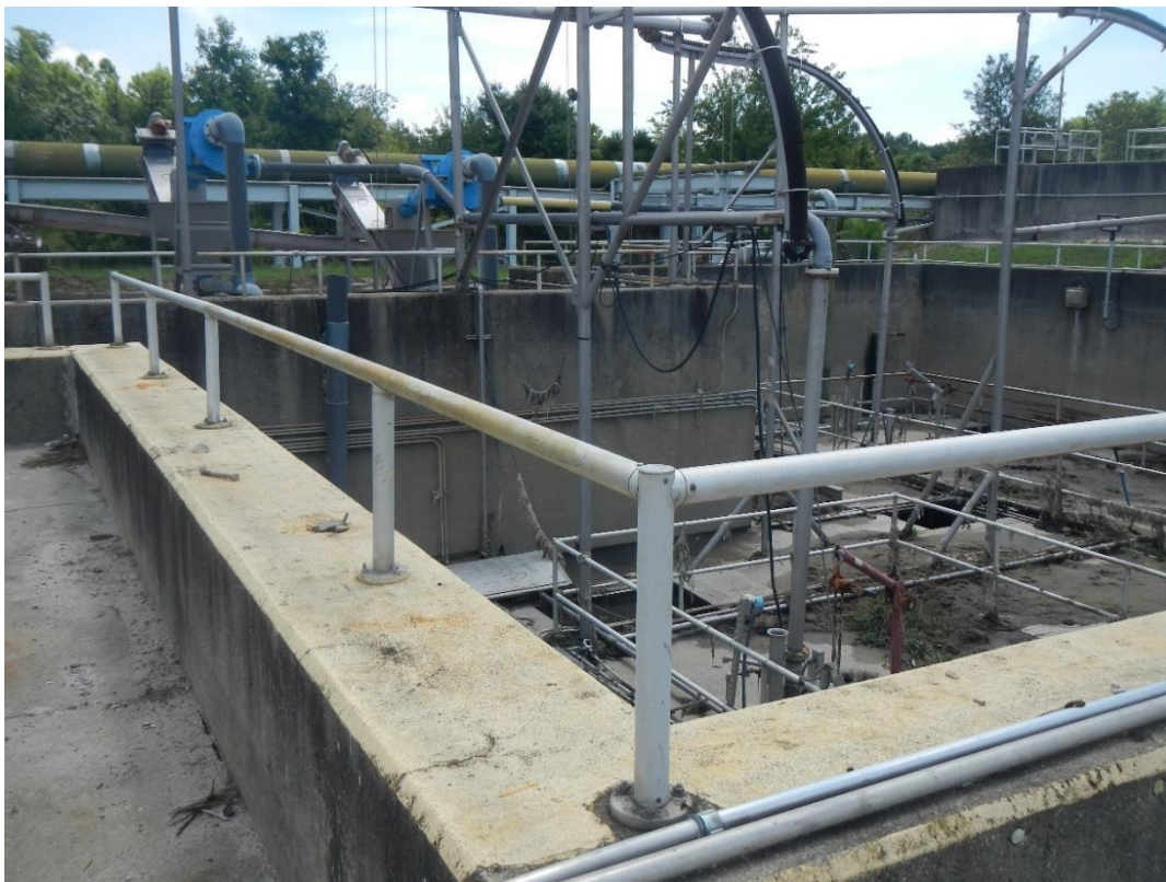
Photo 12: Primary Grit removal was offline at the time of the inspection.
