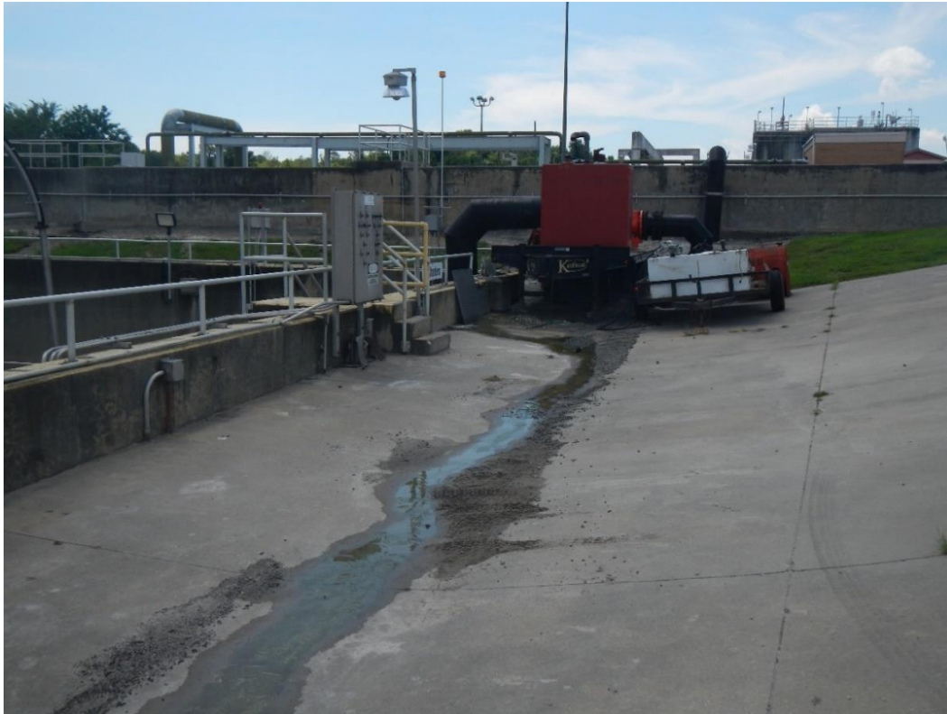
Photo 11: Bypass Pump at primary grit removal to divert flow to constructed wetlands.
