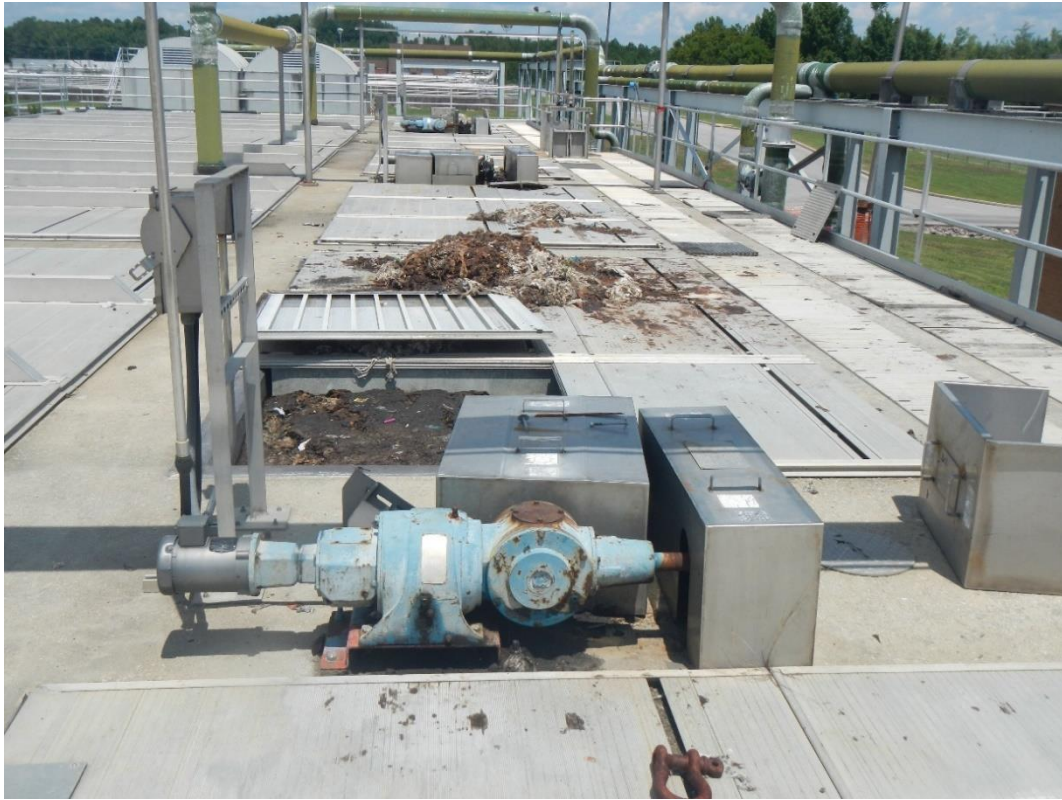
Photo 5: Solids from clarifier maintenance outside of containment.
