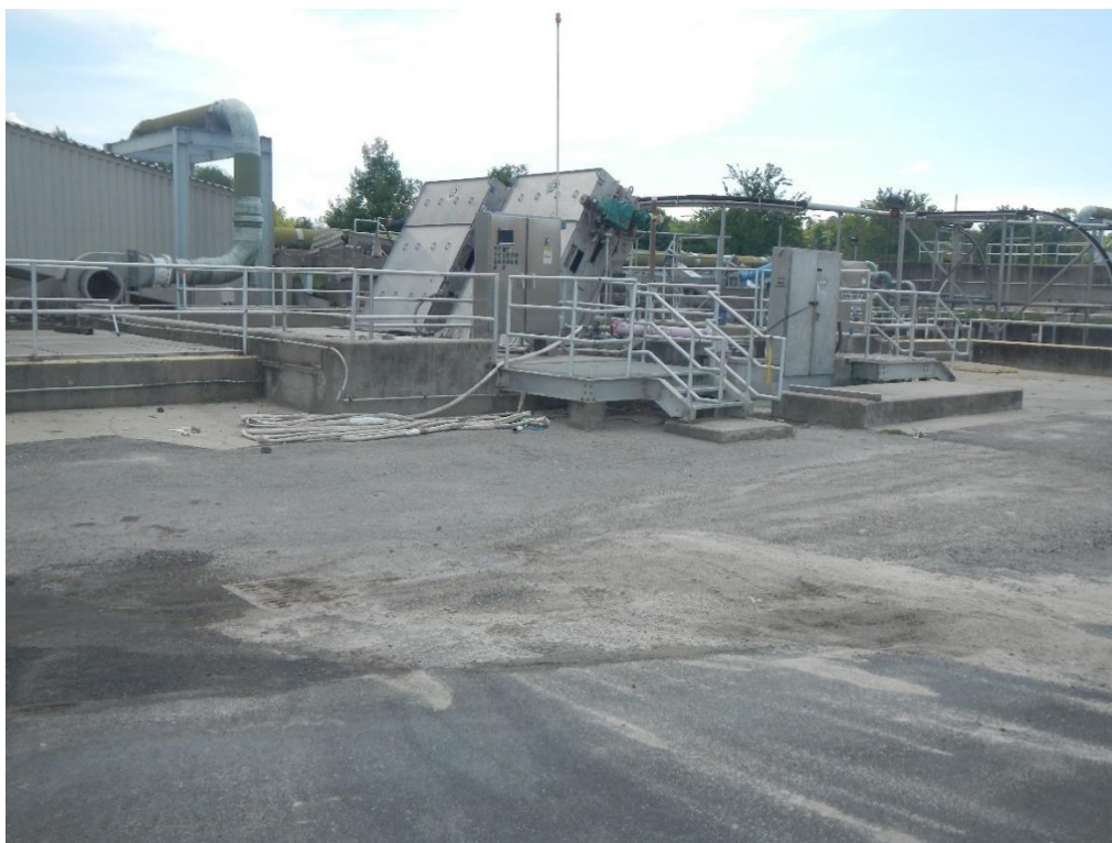
Photo 2: Mechanical bar screens.
