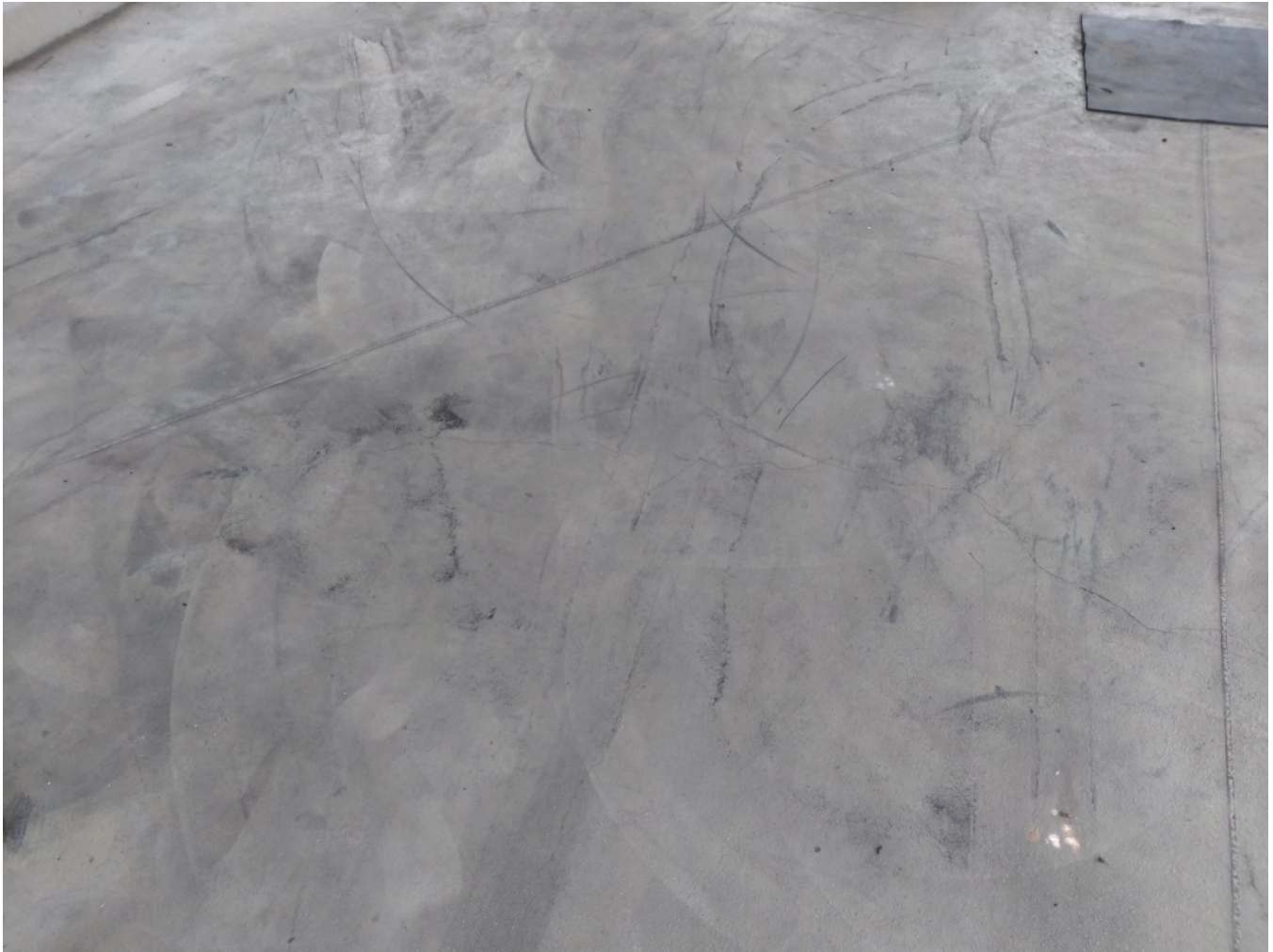
Photograph 8: View of hairline cracks observed in the concrete floor of the hazardous waste storage pad
