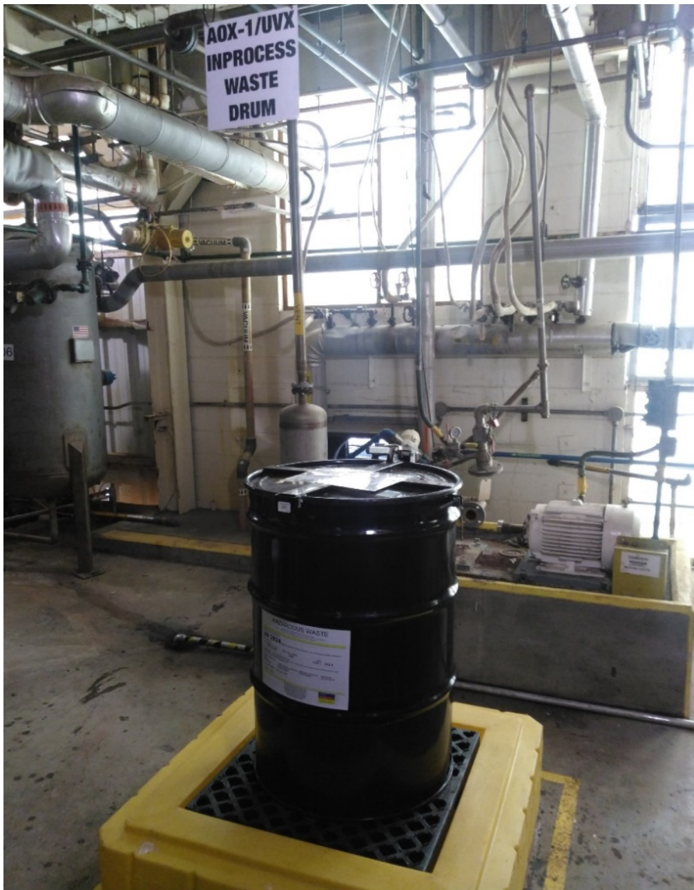
Photograph 2: AOX and UVX sample residues accumulation container in SAA #4 located on the 2nd floor of the main production building.
