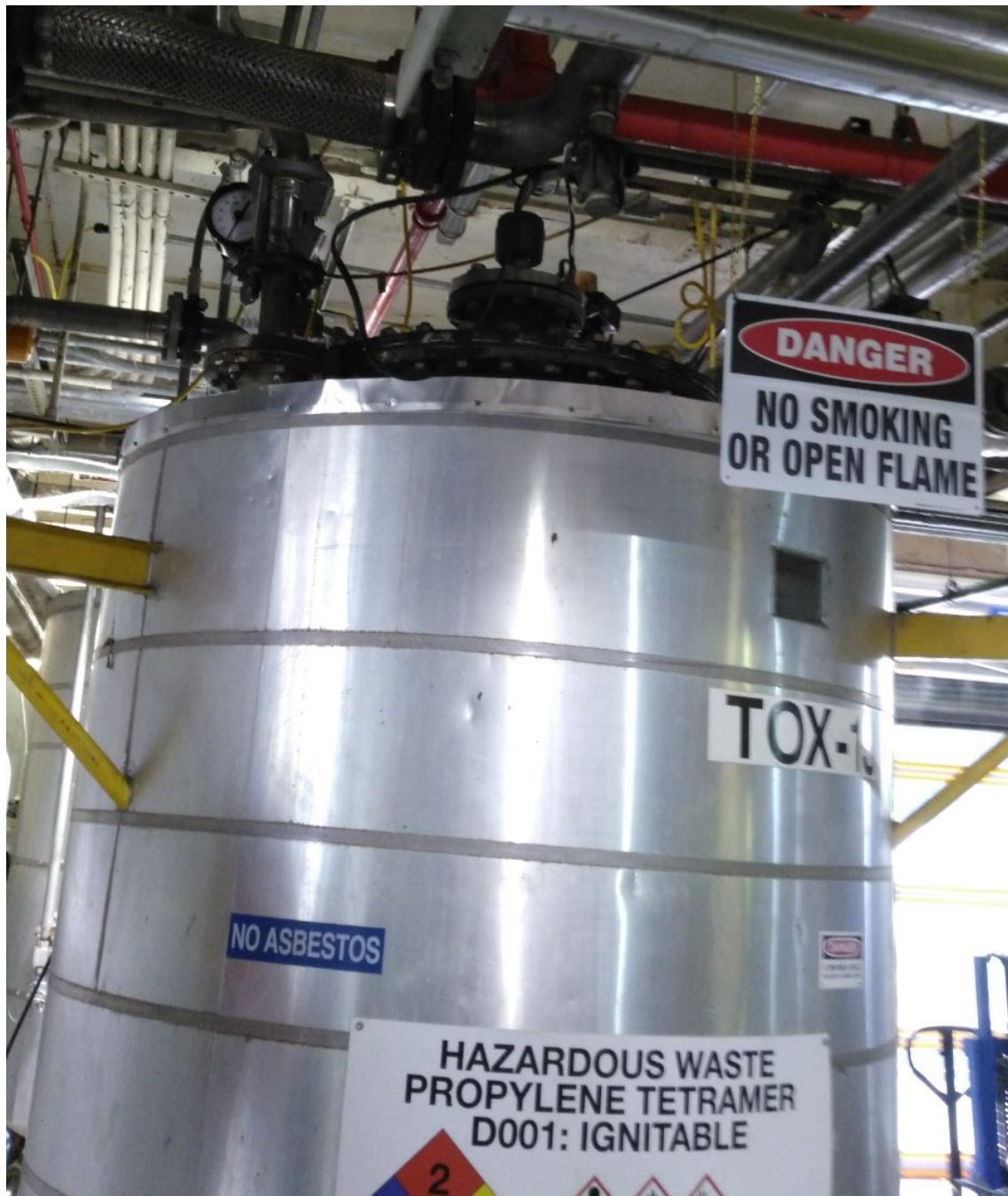
Photograph 5: Aboveground hazardous waste storage tank in the main production building.
