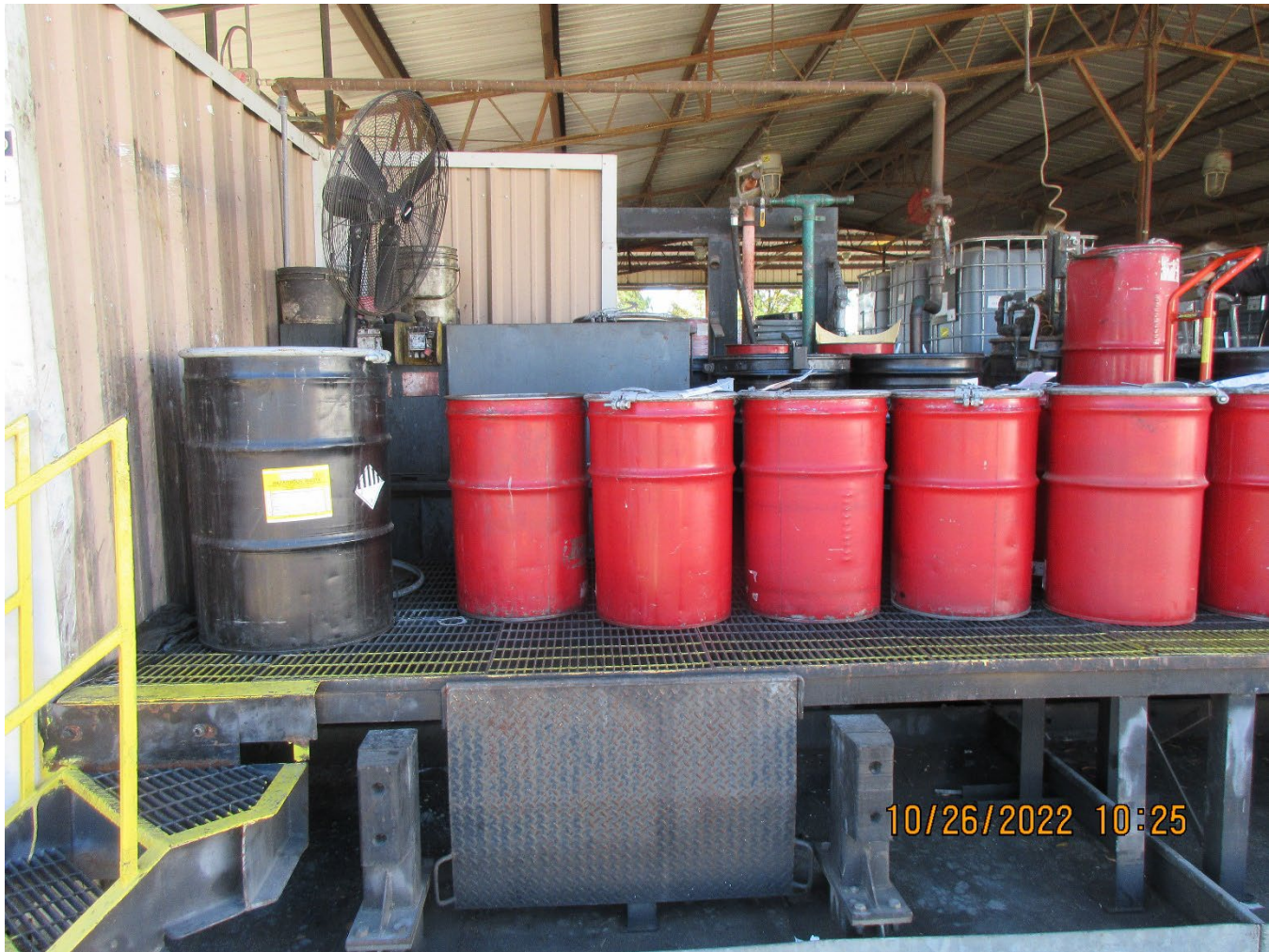
Photo 3 – Northeast Return and Fill Station
