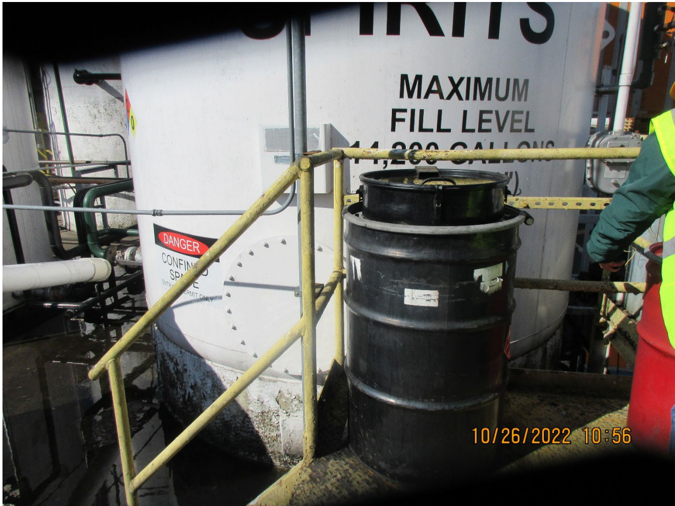
Photo 6 – 55-gallon drum located in SAA in truck loading area
