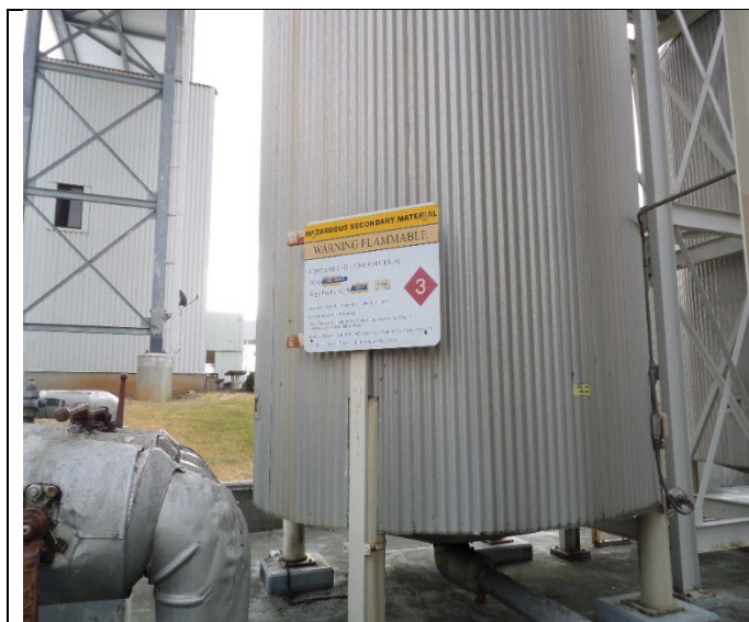
Outdoor Tank Farm. HSM Tank #3 waste paint and solvent from SUV paint line. Photograph 1 taken at 9:59 a.m.
