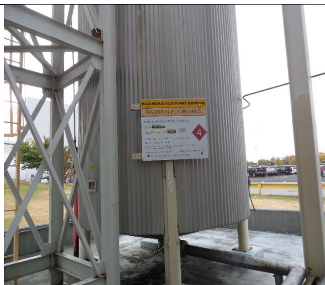
Outdoor Tank Farm. HSM Tank #4 waste paint and solvent from super duty truck paint line. Photograph 2 taken at 9:59 a.m.
