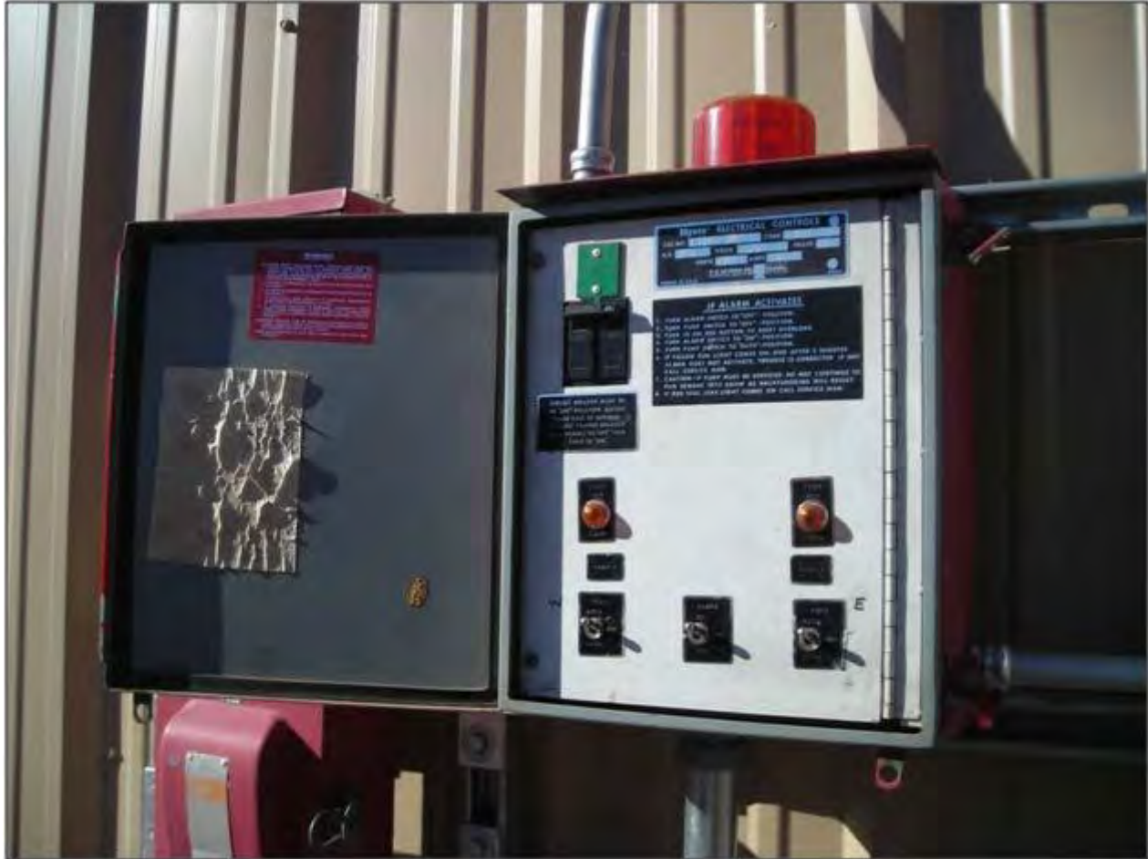
Photo Information: Rain gauge/pump panel. The system does allow for a manual override to pump even when the rain gauge has stopped the system.
