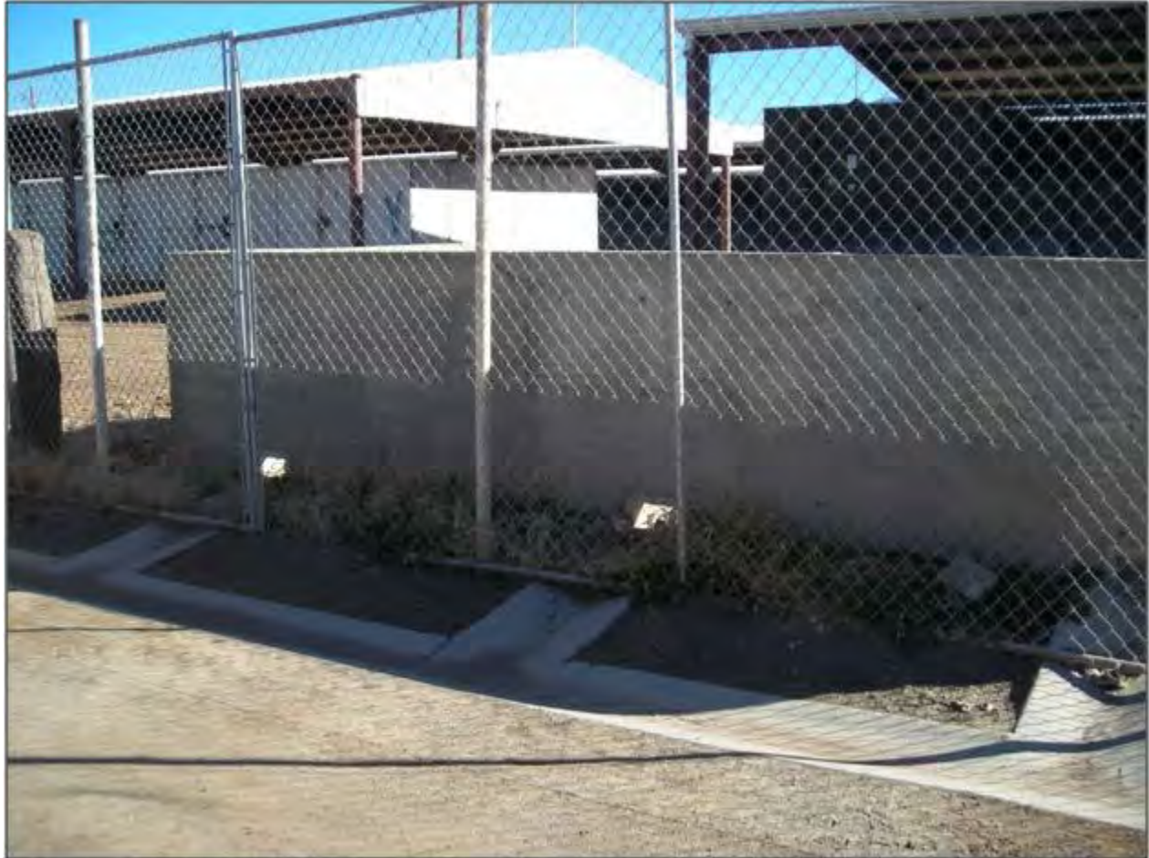
Photo Information: The horse wash racks are directly connected to the new conveyance.
