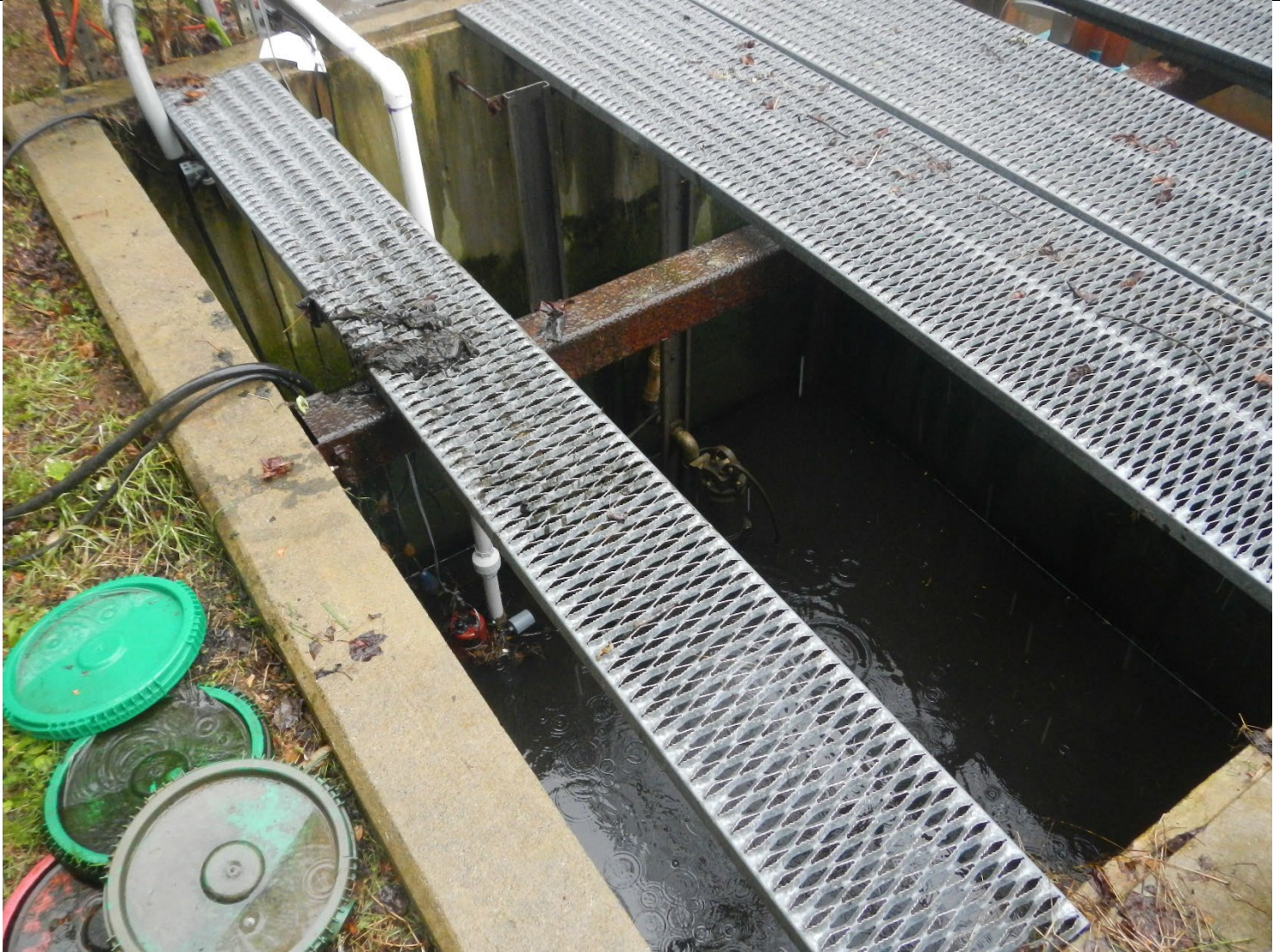
Figure 2 Recirculation system with example of debris buildup.
