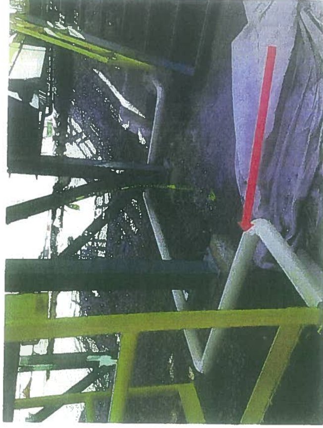
Oleum System Expansion Loop
