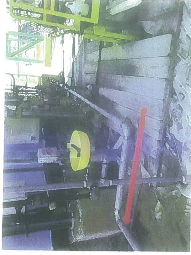
Sulfuric Acid System Expansion Loop
