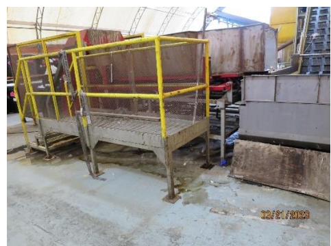
Photo #40 – Spilled liquid pharmaceutical waste Under the shredding unit.
