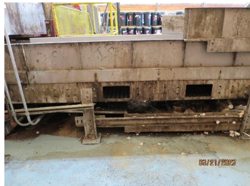
Photo #36 – Spilled pharmaceutical wastes under the shredding unit.
