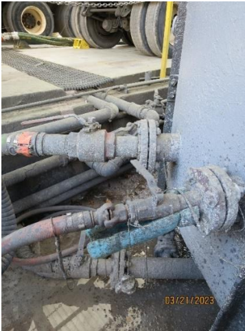
Photo #19 – ancillary equipment connections are not identified with a tag.
