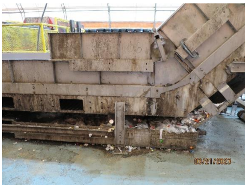
Photo #35 – Spilled pharmaceutical wastes under the shredding unit.
