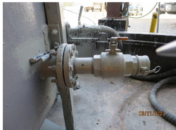
Photo #18 – ancillary equipment connections are not identified with a tag.
