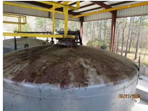
Photo #22 – ancillary equipment connections are not identified with a tag.
