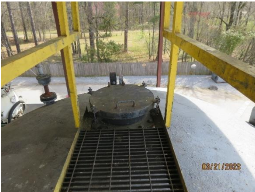
Photo #21 – ancillary equipment connections are not identified with a tag.
