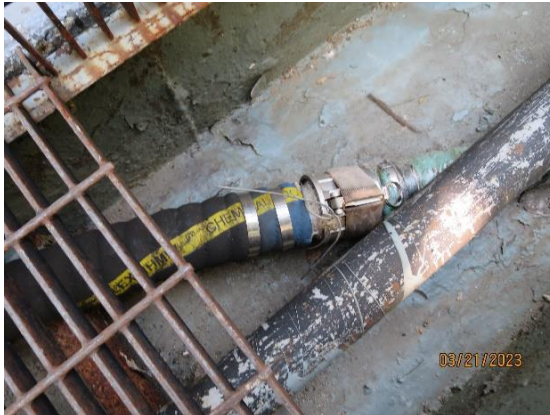
Photo #15 – ancillary equipment connections are not identified with a tag.
