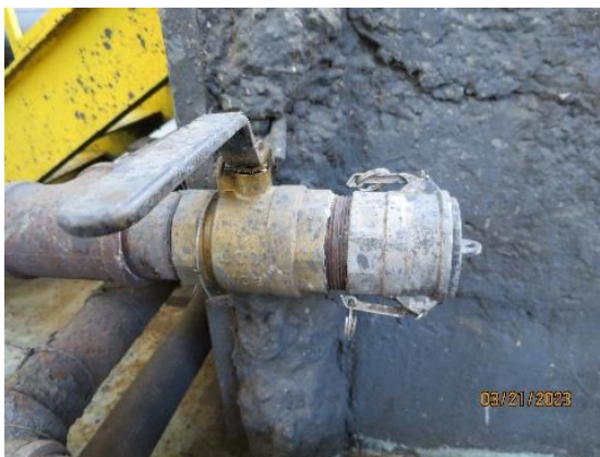
Photo #17 – ancillary equipment connections are not identified with a tag.
