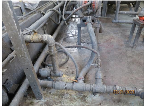
Photo #16 – ancillary equipment connections are not identified with a tag.
