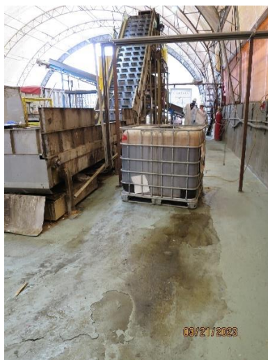
Photo #42 – Spilled liquid pharmaceutical waste From the shredding unit and SAA container.
