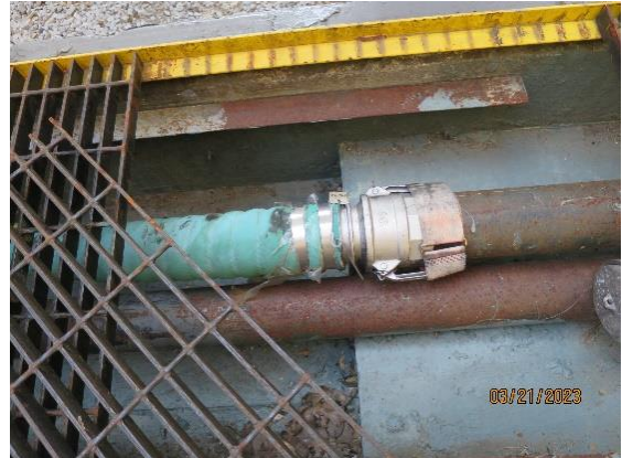
Photo #14 – ancillary equipment connections are not identified with a tag.
