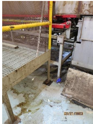
Photo #38 – Spilled pharmaceutical wastes under the shredding unit.
