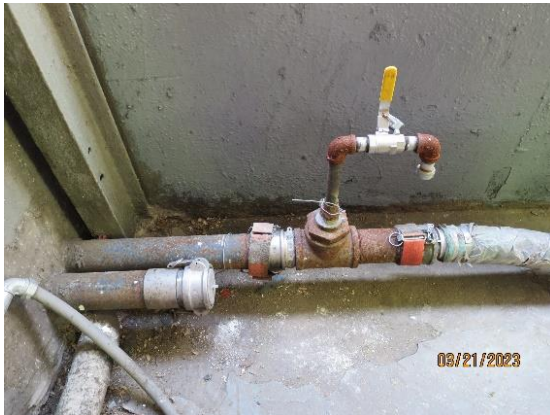
Photo #13 – ancillary equipment connections are not identified with a tag.
