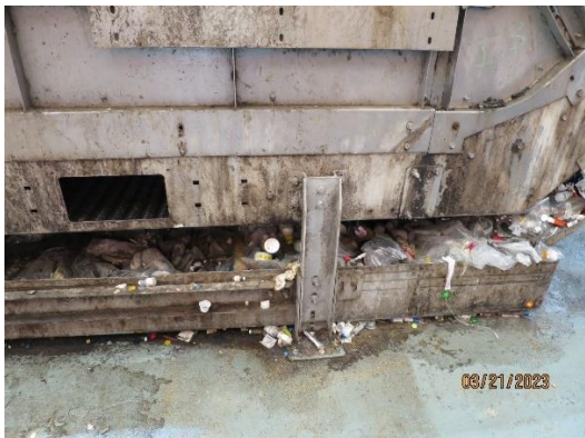
Photo #37 – Spilled pharmaceutical wastes under the shredding unit.
