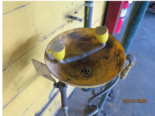
Photo #2 – Eye wash located in Building #1.
