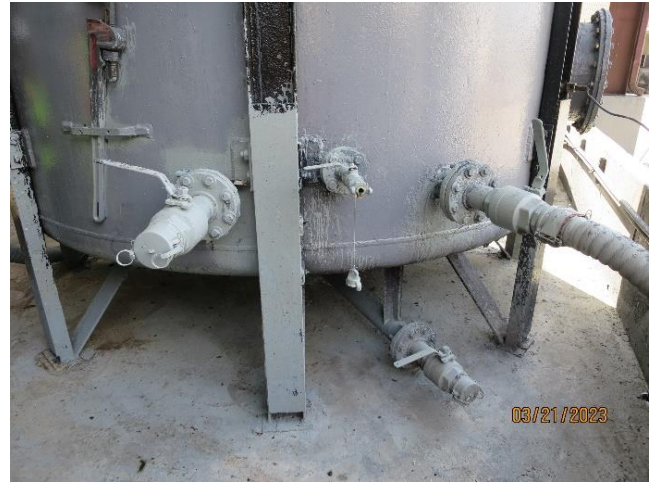
Photo #20 – ancillary equipment connections are not identified with a tag.
