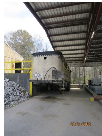
Photo #28 – Missing an indication of the hazards of the contents.
