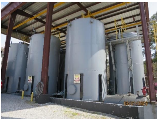
Photo #11 – Hazardous waste tank farm.
