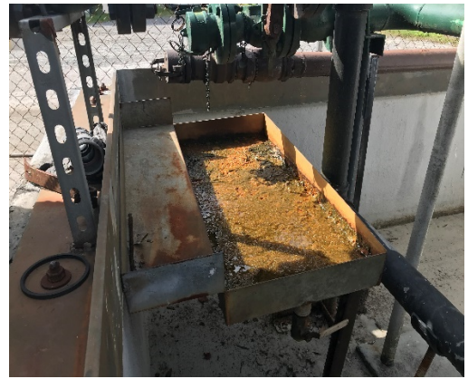
Picture 16: Unknown Residual Waste in a tray in Secondary Containment of Hazardous Waste Tank #1
