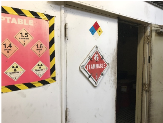
Picture 1: Signage at Flammable Container Storage Area #3 (Main)
