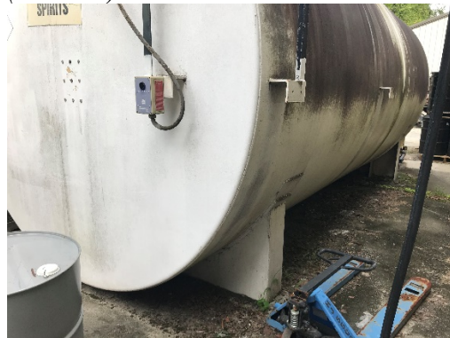
Picture 24: Double walled, 10,000-gallon Clean Solvent Tank
