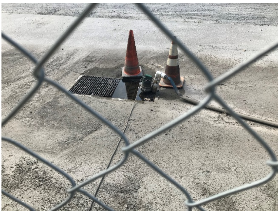
Picture 8: A pump not in service used for pumping the storm water runoff from the tank farm and return and fill unit into an unnamed tributary of a creek.
