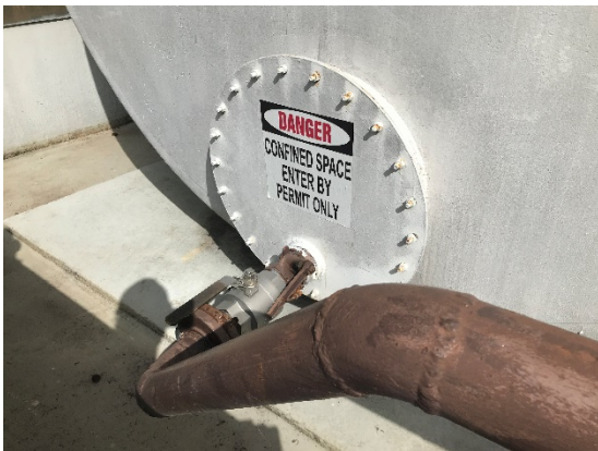
Picture 15: Sign of Rust and Paint Peeling in Ancillary Equipment associated with Hazardous Waste Tank #1
