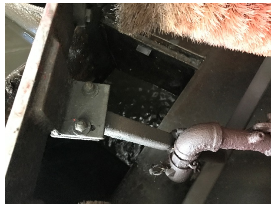
Picture 6: Hazardous Waste Liquid (D001, D006, D008, D018, D039 and D040) in the Waste Sump of the Return and Fill Unit when not in service
