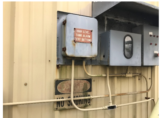
Picture 17: High Level Tank Alarm was not in service for Hazardous Waste Tank #1 at the time of inspection
