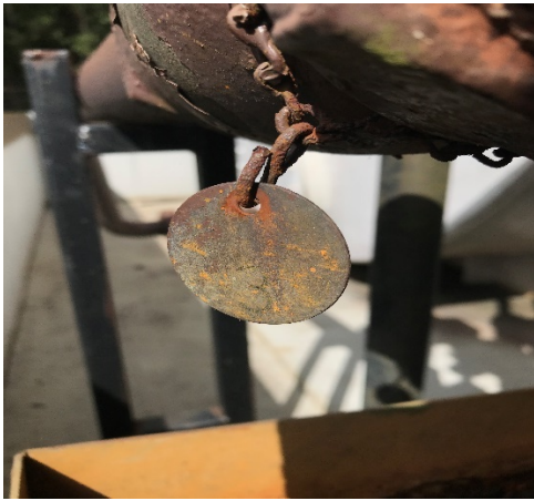
Picture 19: Tags associated with the Ancillary Equipment were not clear and visible
