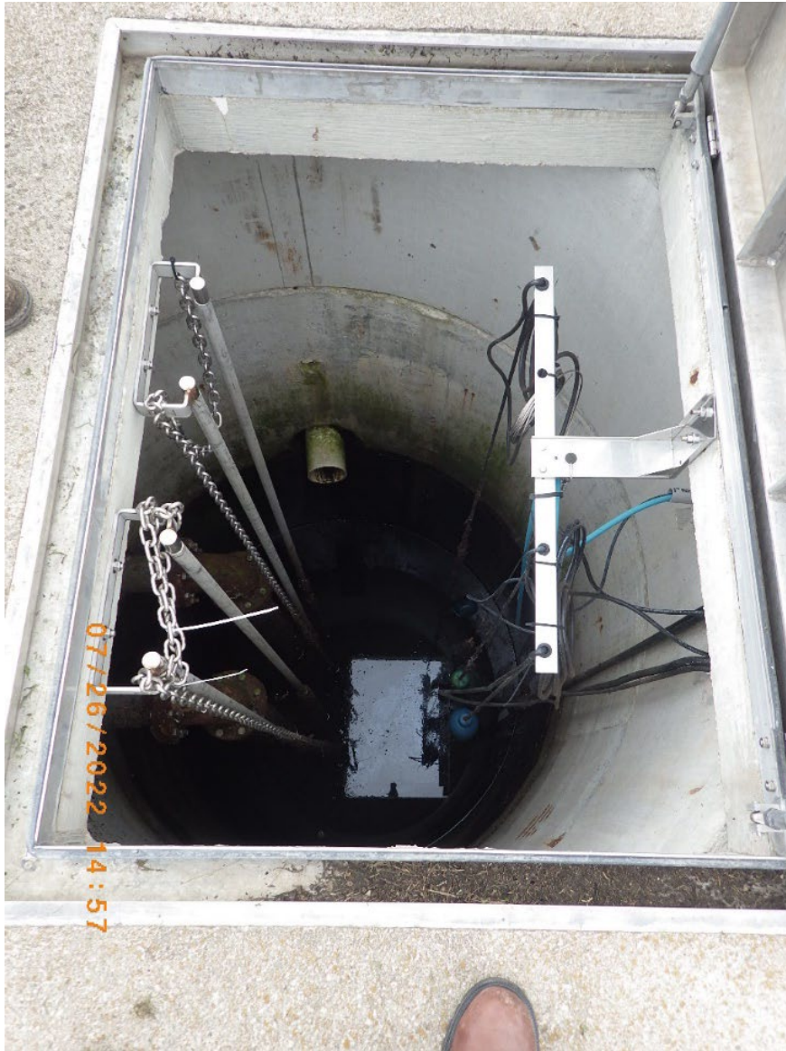
19: ONGA0302 Description: RAS/WAS pump manhole. GPS Latitude: 40° 44' 21" GPS Longitude: 88° 0' 7" Camera Direction: Down Date/Time: July 26, 2022 2:57PM
