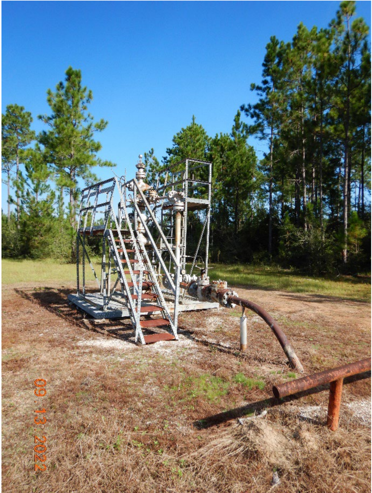
Photograph 2: Looking west, site overview showing well head, pressure gauges, valves, and as stairway.
