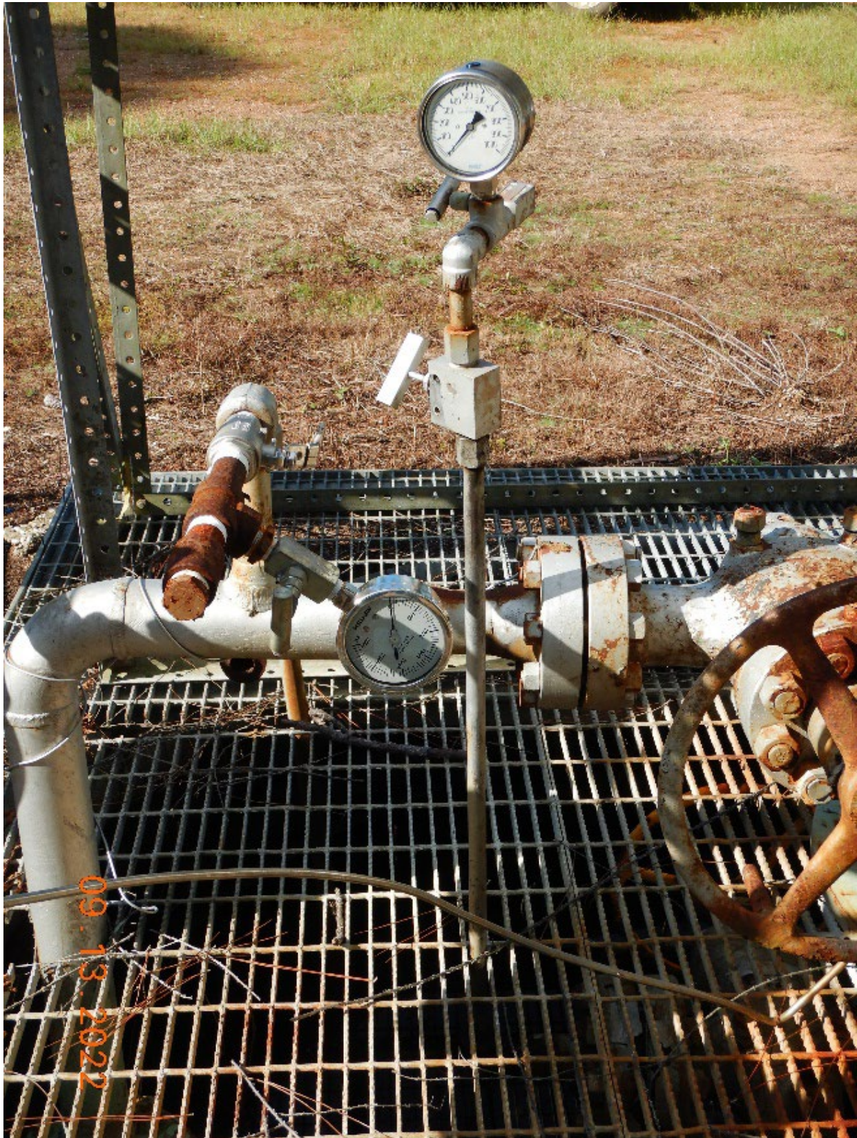
Photograph 3: Looking south, closeup view of surface pressure gauge reading 0 psi.
