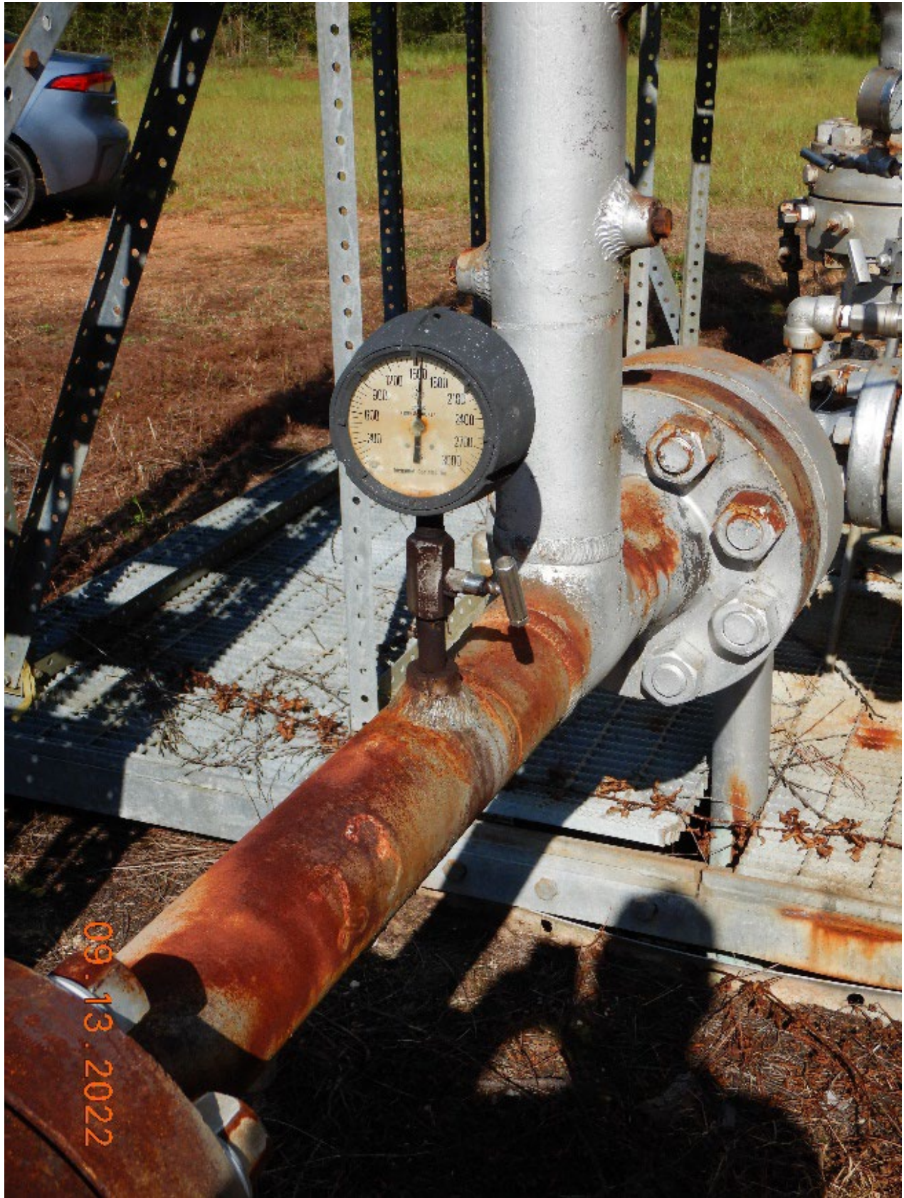
Photograph 5: Looking west, closeup view of line pressure gauge reading 1,600 psi.
