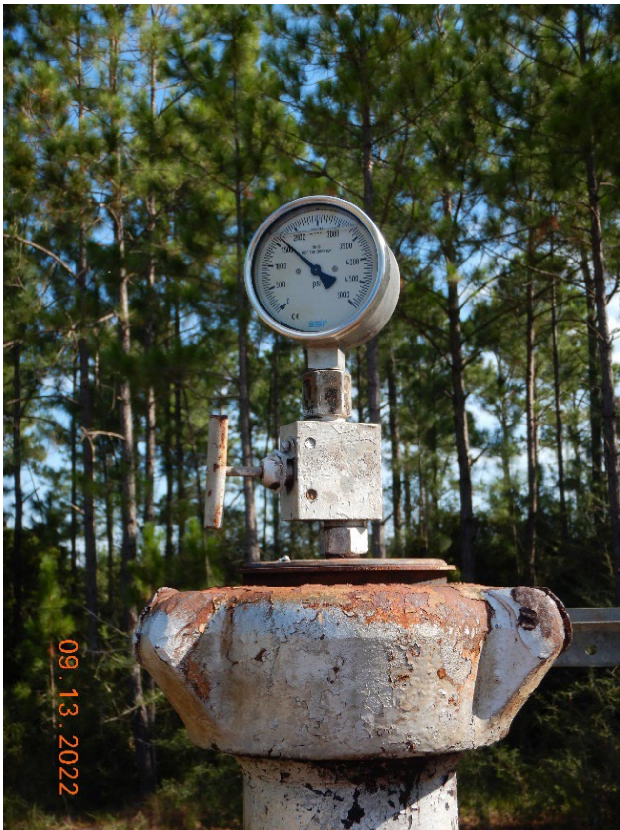
Photograph 6: Looking north, closeup view of internal pressure gauge reading 1,600 psi.
