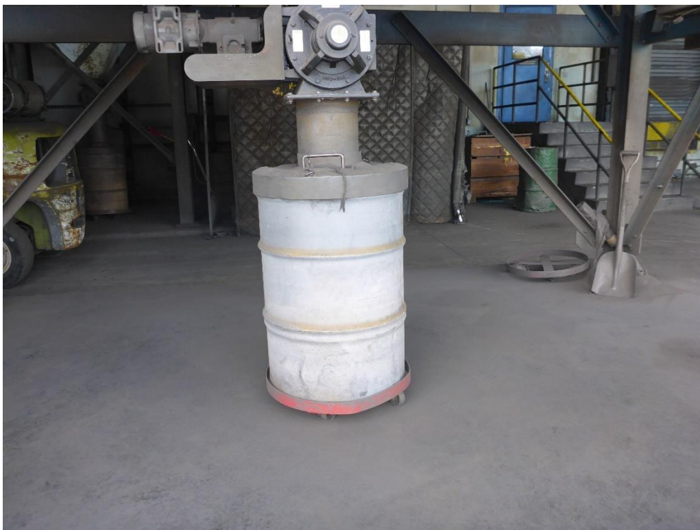
Photo 18: 55-gallon drum under Grinding Baghouse. The drum is not labeled.
