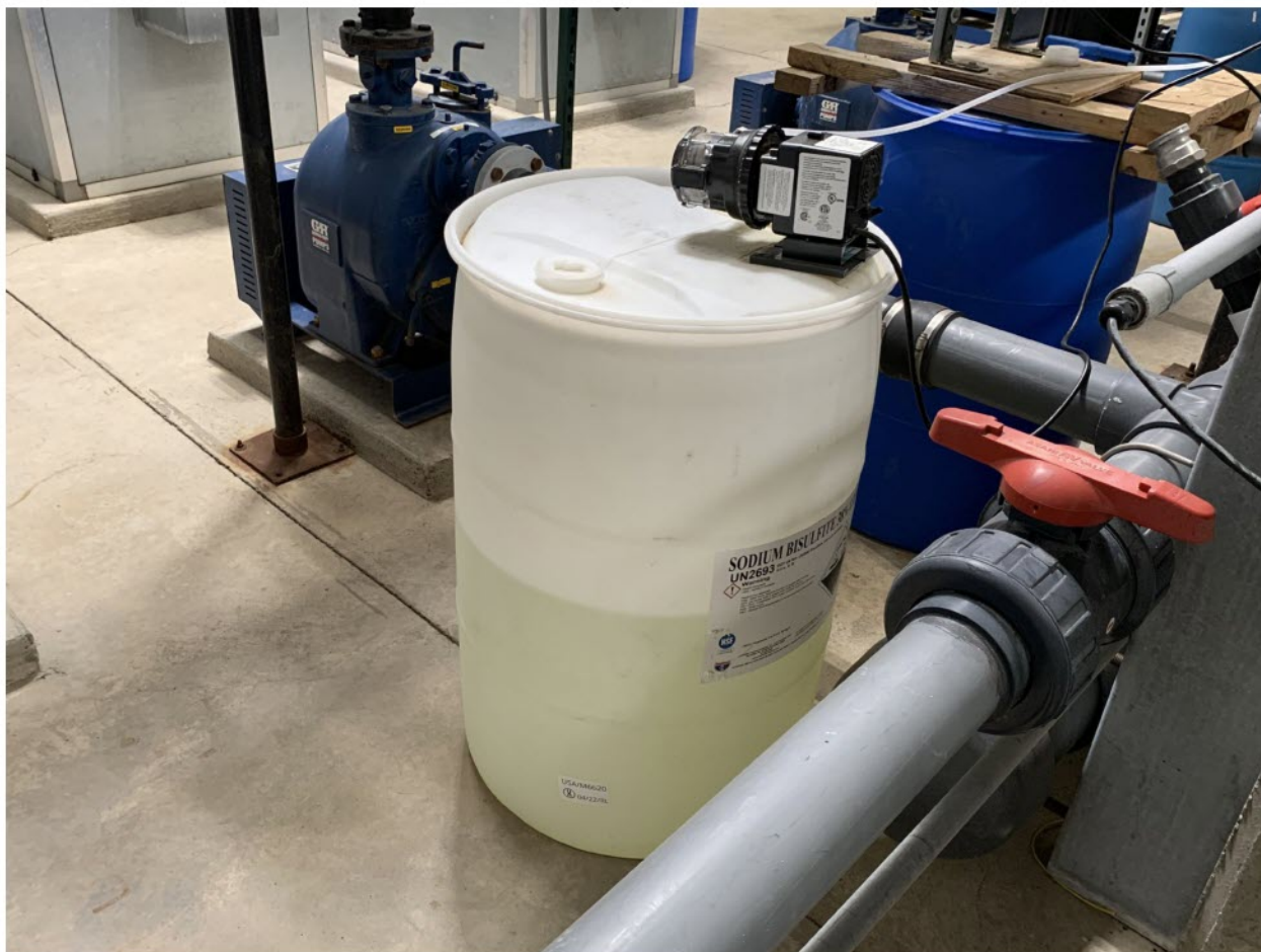
View of the bulk Sodium Bisulfite solution and peristaltic pump used in the treatment process. (IMG0149). September 13, 2022. Photographed by D. Esparza
