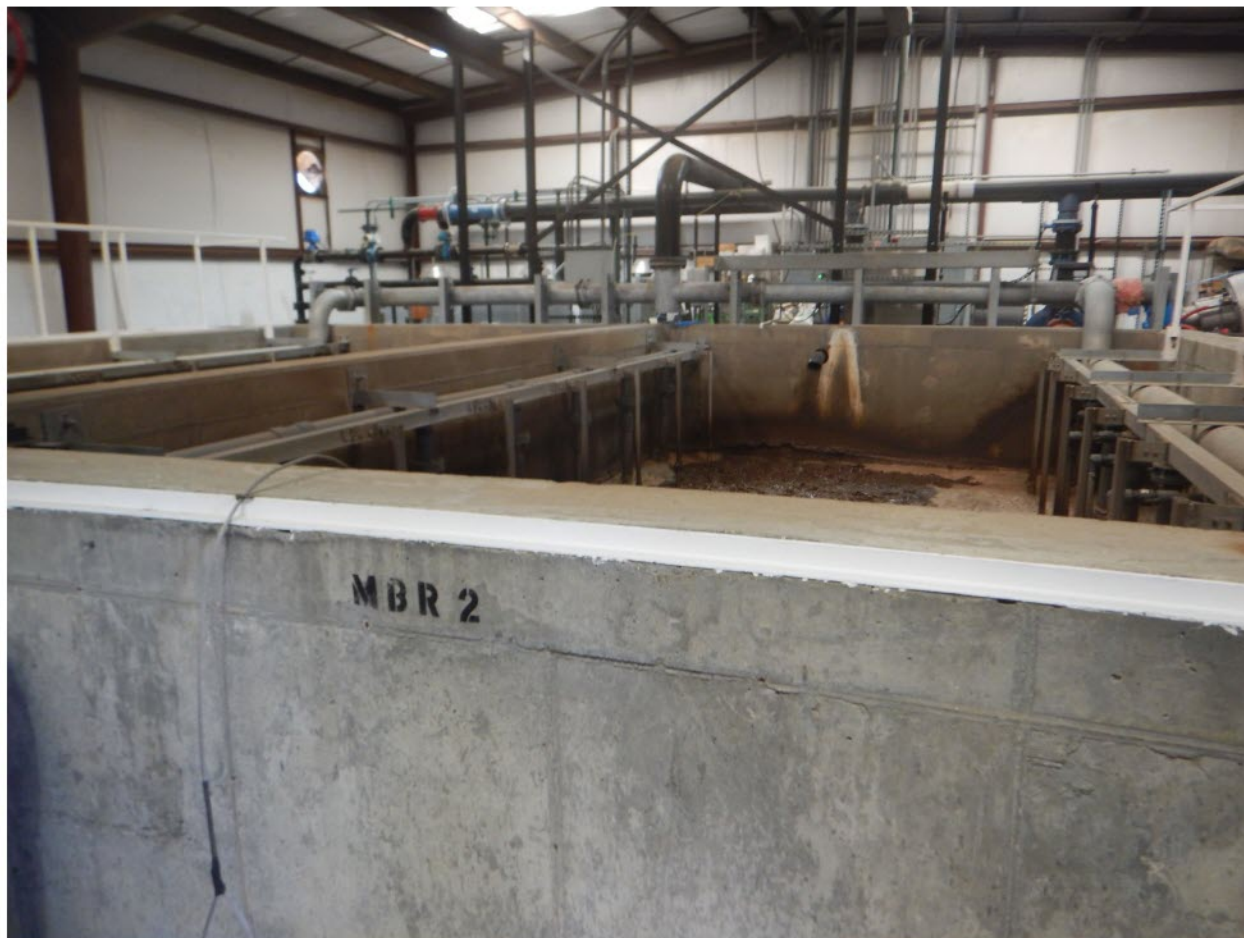
Overall view of the Casa Blanca membrane bioreactor (MBR) basin #2. (DSCN1662). September 13, 2022. Photographed by D. Esparza
