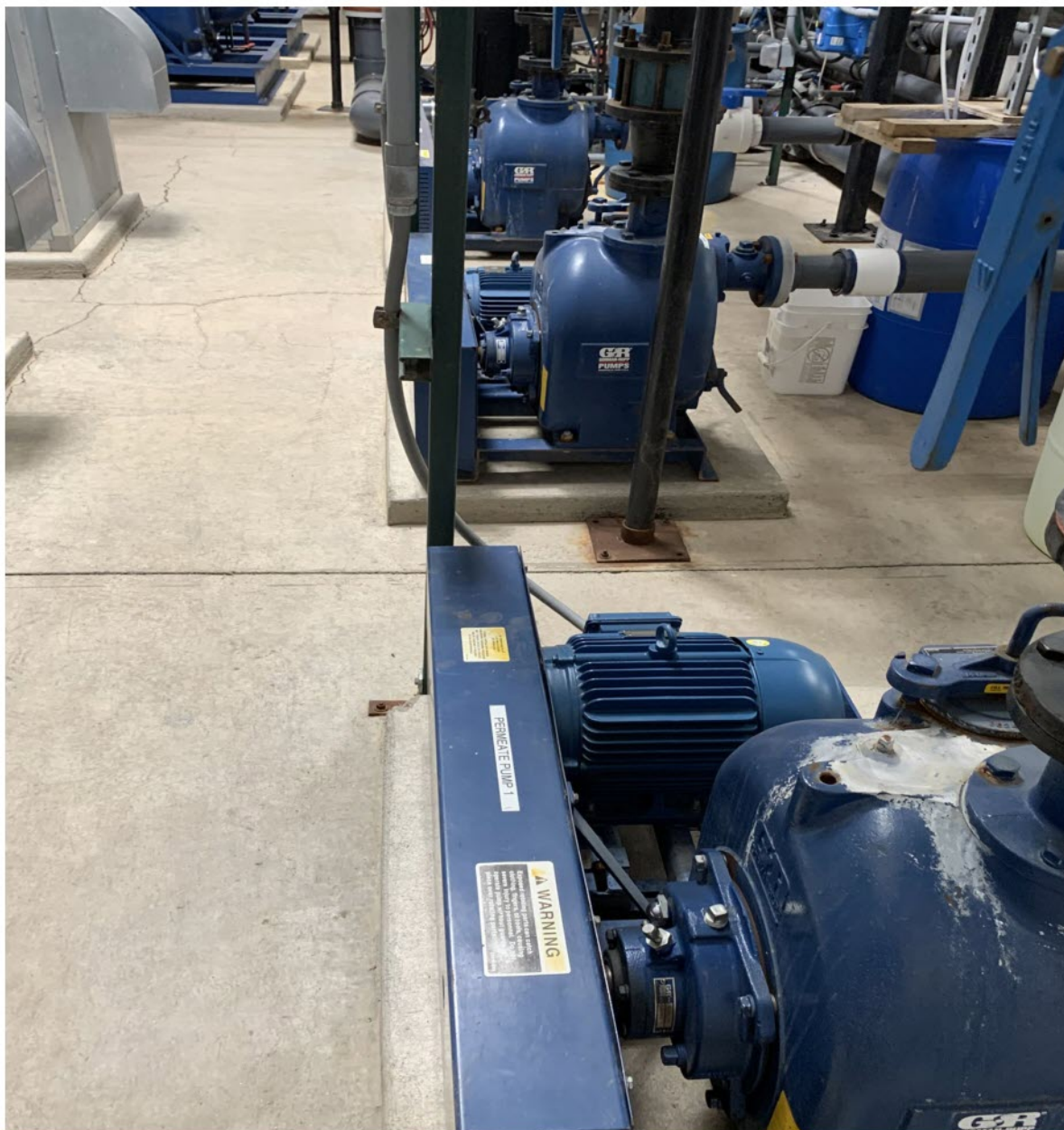
Overall view of the WWTPs permeate pumps. (IMG0148). September 13, 2022. Photographed by D. Esparza
