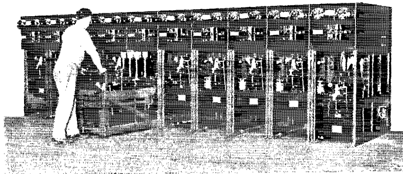
Figure 7. A "roll out" carbon circuit breaker installation.
