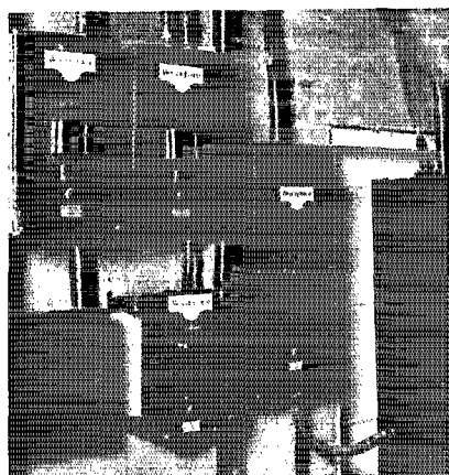
Figure 4. A group of ABI De-ion circuit breakers for industrial feeder circuits.
