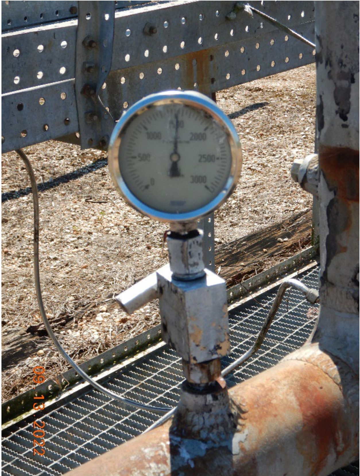
Photograph 5: Looking south, view of incoming line pressure gauge reading 1,520 psi.
