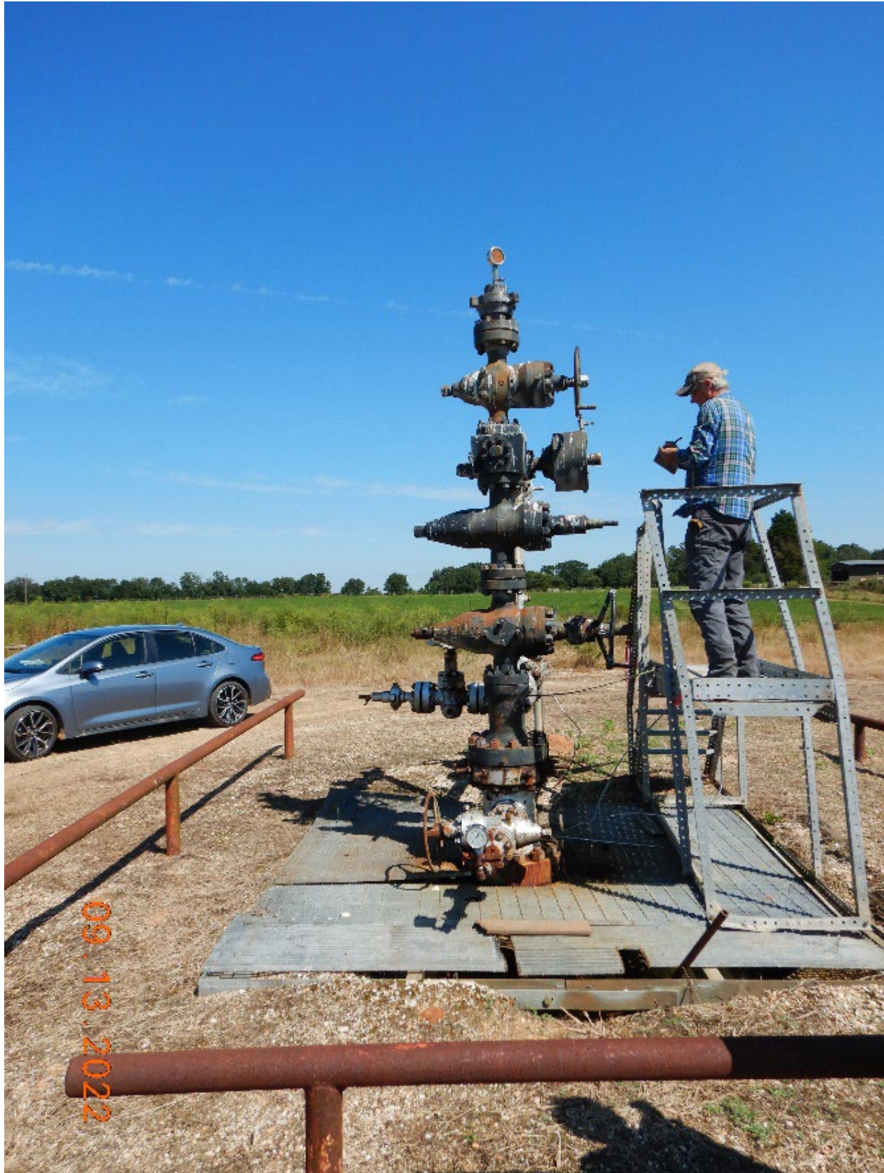
Photograph 2: Looking north, site overview, showing well head, pressure gauges, valves, and access stairs.
