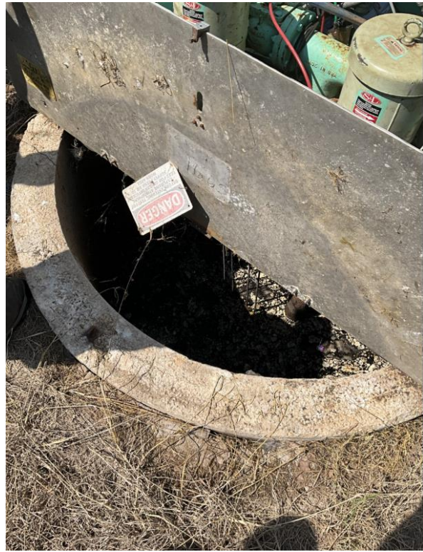
Photo 2: Lift station no.1 well full.
