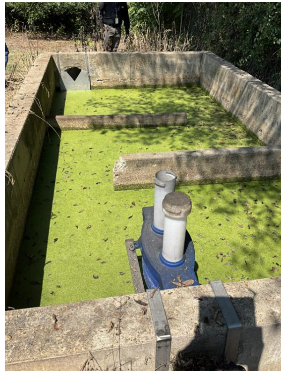
Photo 4: V-notch weir & Chlorine contact chamber
