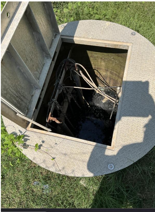
Photo 3: Lift station no. 2
