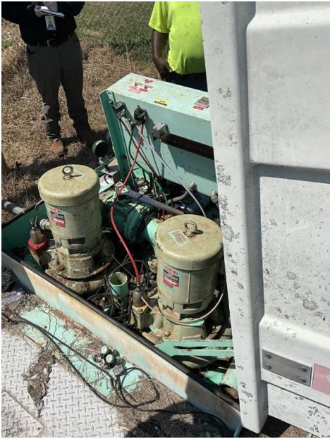
Photo 1: Inoperable pump at lift station no.1.
