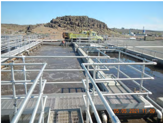
Photo #:03 (DSCN2135) Description: Facing northeast, photo of the first and second aeration basins from above the surge tank.
