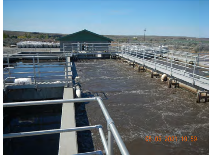
Photo #:02 (DSCN2134) Description: Facing southwest, photo of the first stage aeration basin.
