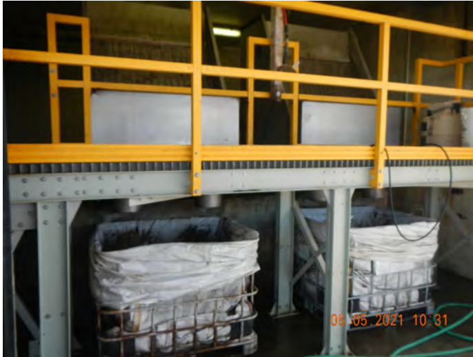
Photo #:01 (DSCN2127) Description: Facing northeast, photo of the two hydrasieve screens
