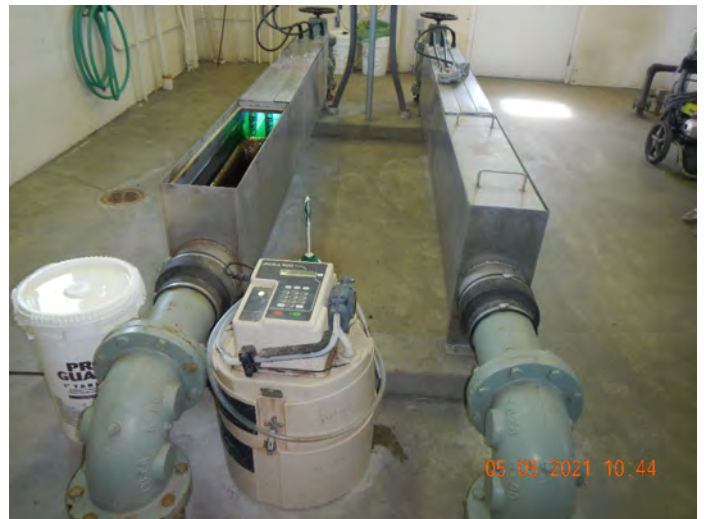
Photo #:04 (DSCN2128) Description: Photo of the UV disinfection system.
