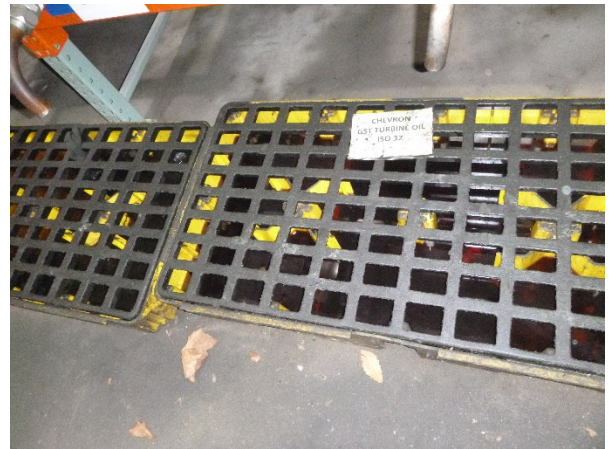
Photograph 30: Oil Building with oil accumulated in floor drains.
