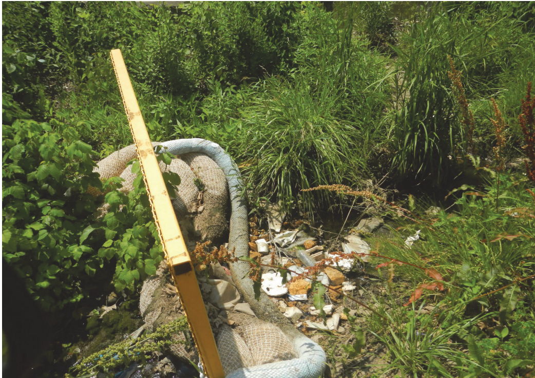
Photo 26, Floatables accumulating at Outfall 001
