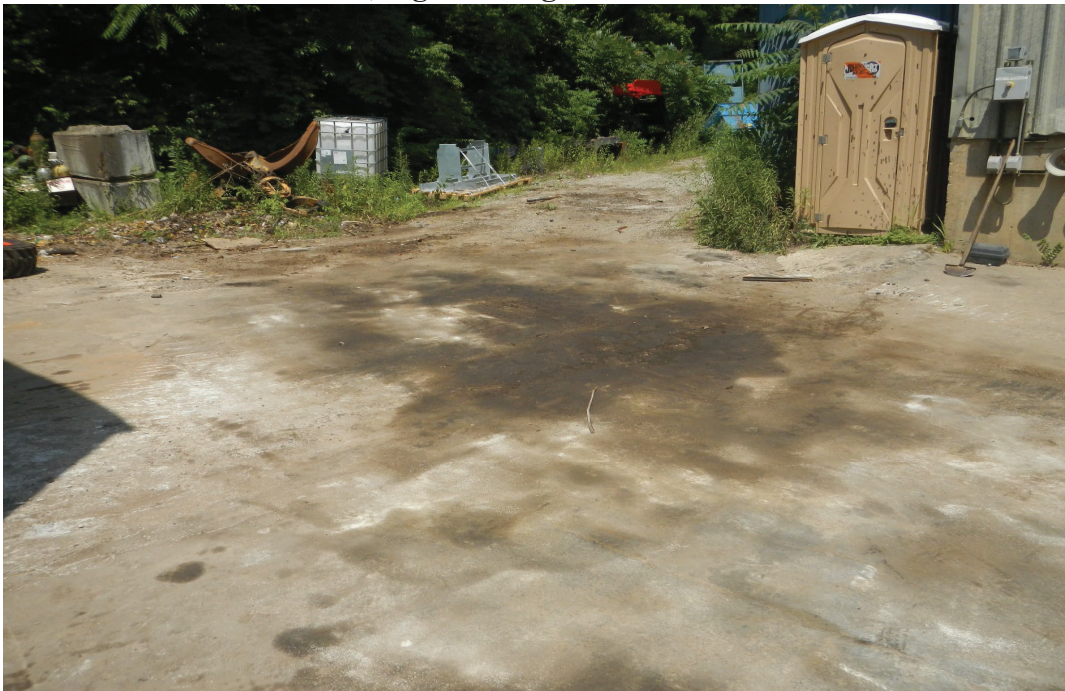
Photo 17, Significant ground discoloration
