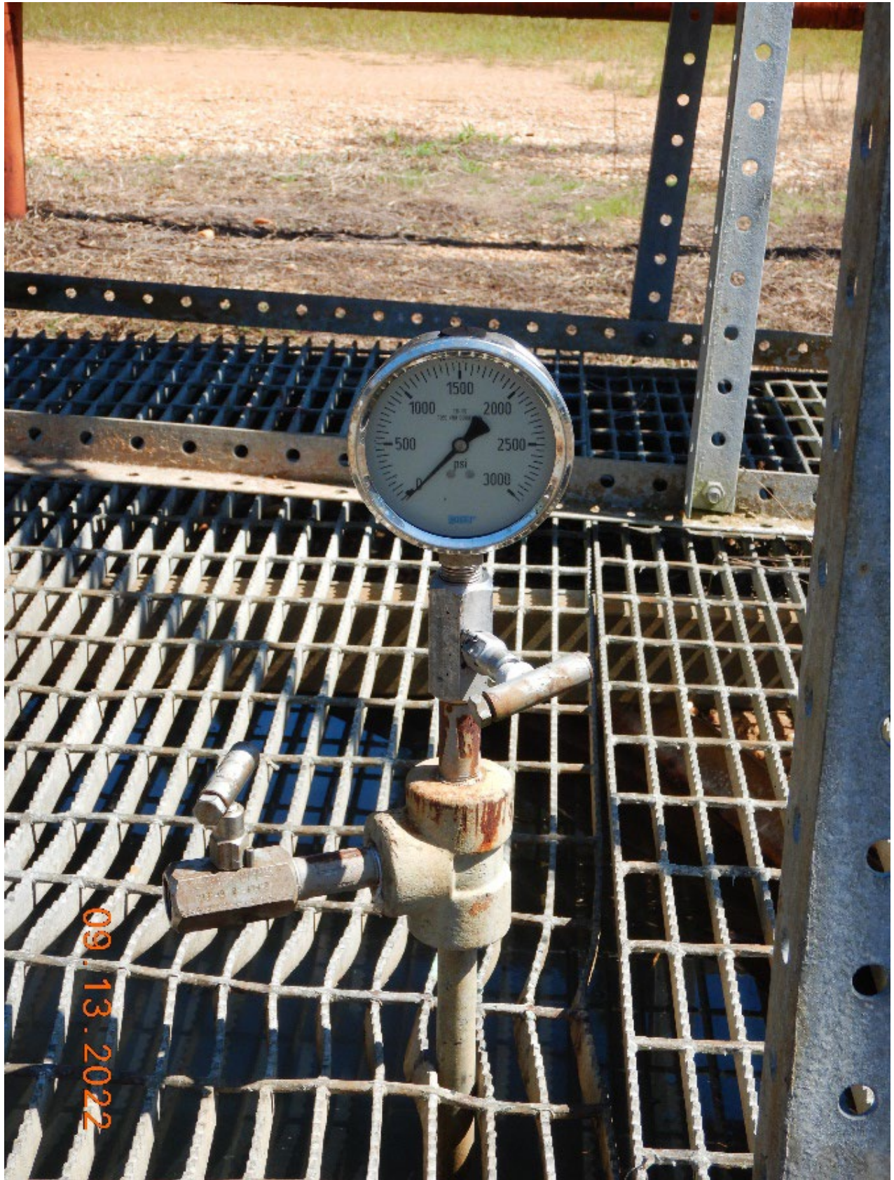
Photograph 3: Looking north, closeup view of surface pressure gauge reading 0 psi.
