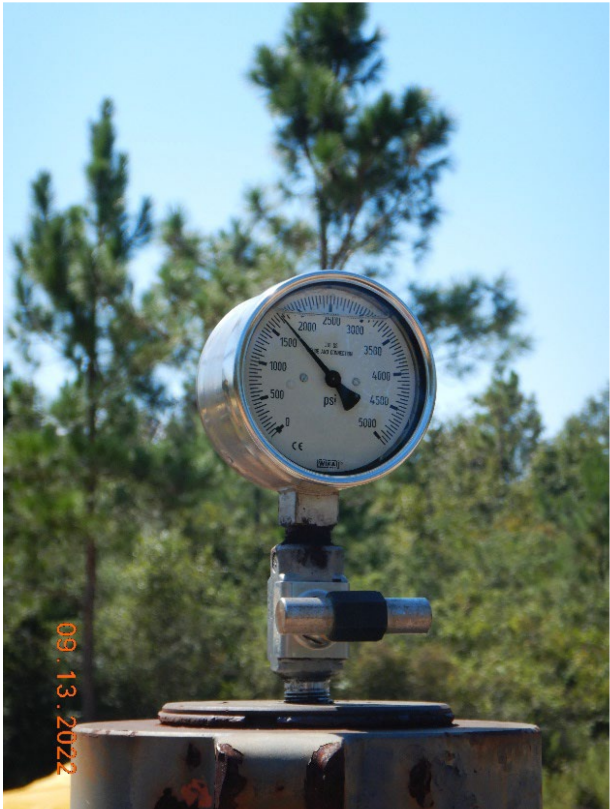
Photograph 6: Looking east, view of internal pressure gauge reading 1,700 psi.
