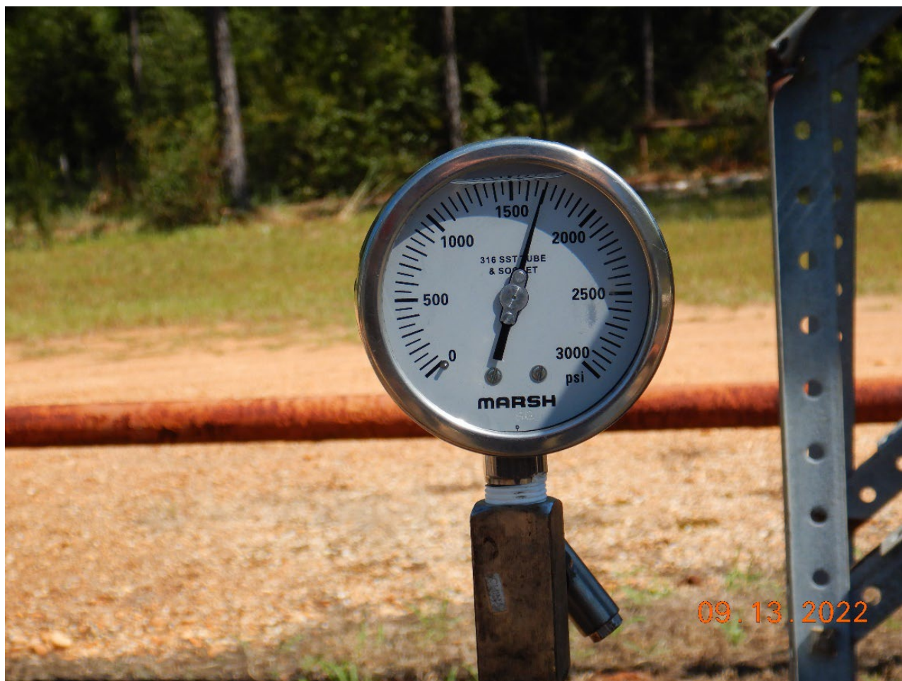
Photograph 5: Looking north, view of incoming line pressure gauge reading 1,700 psi.
