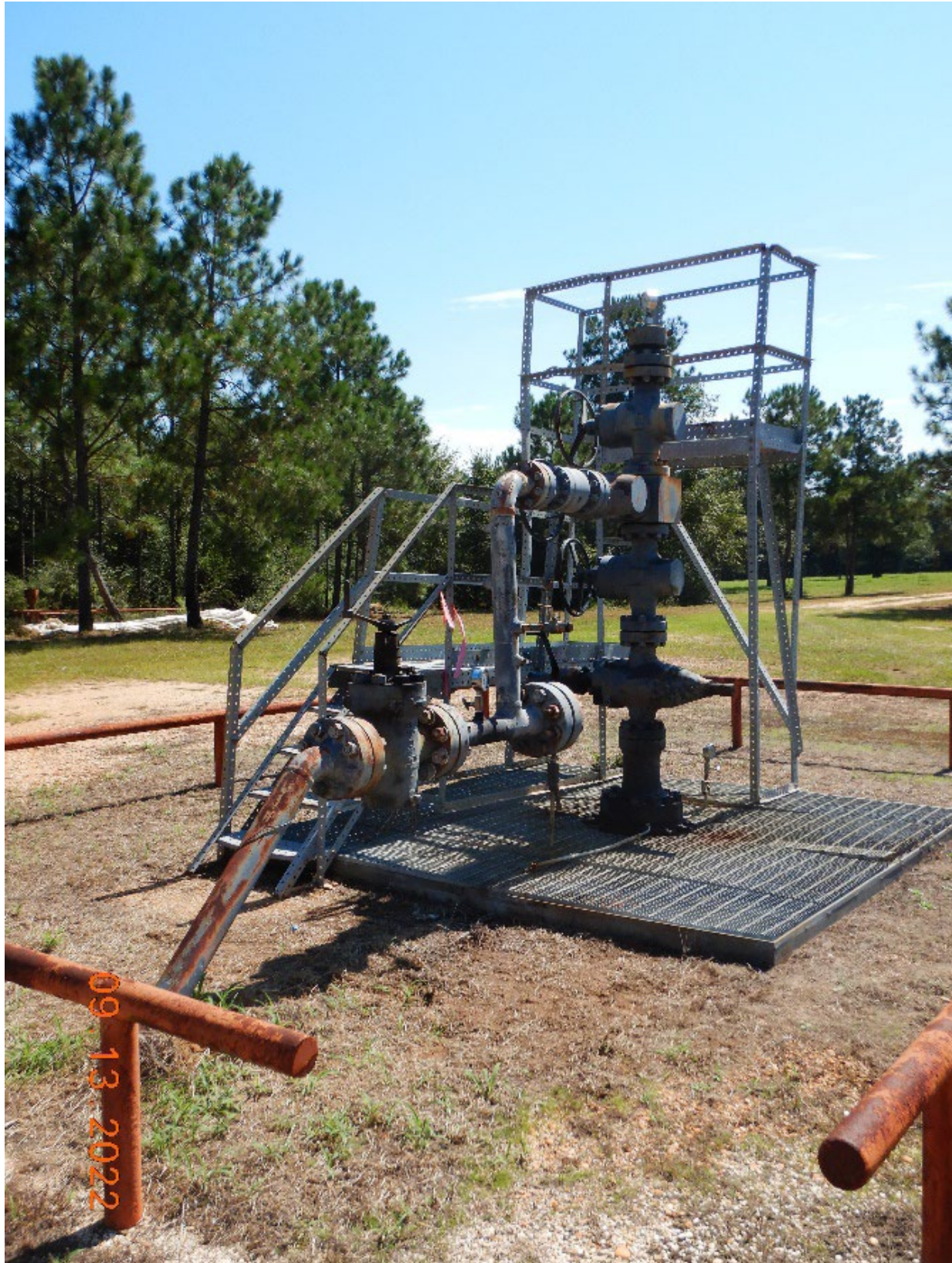
Photograph 2: Looking east, site overview, showing well head, pressure gauges, valves, and access stairs.
