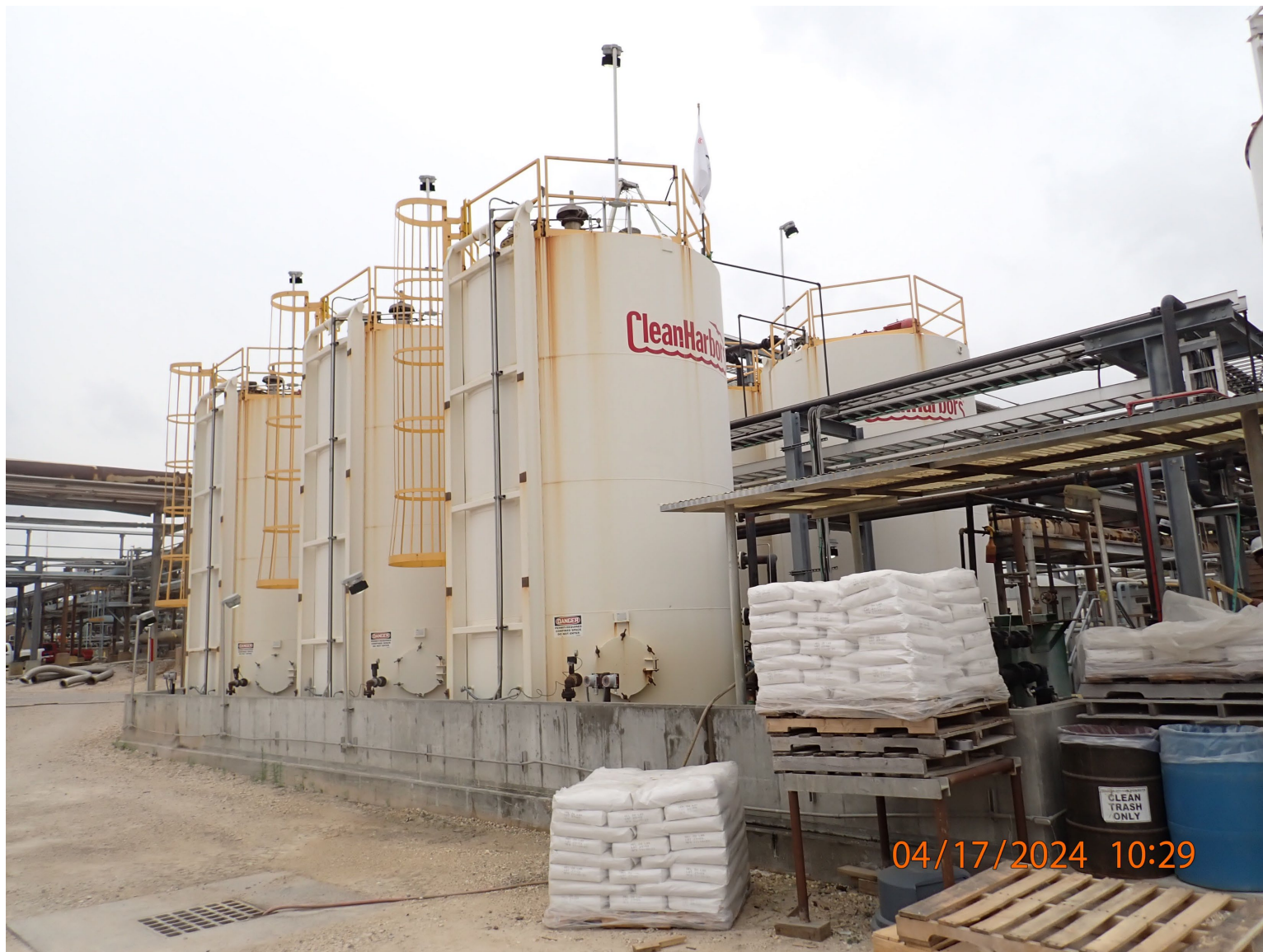
Photo 017: Clean Harbors sludge holding tanks 4/17/2024 10:29 P4170017.jpg
