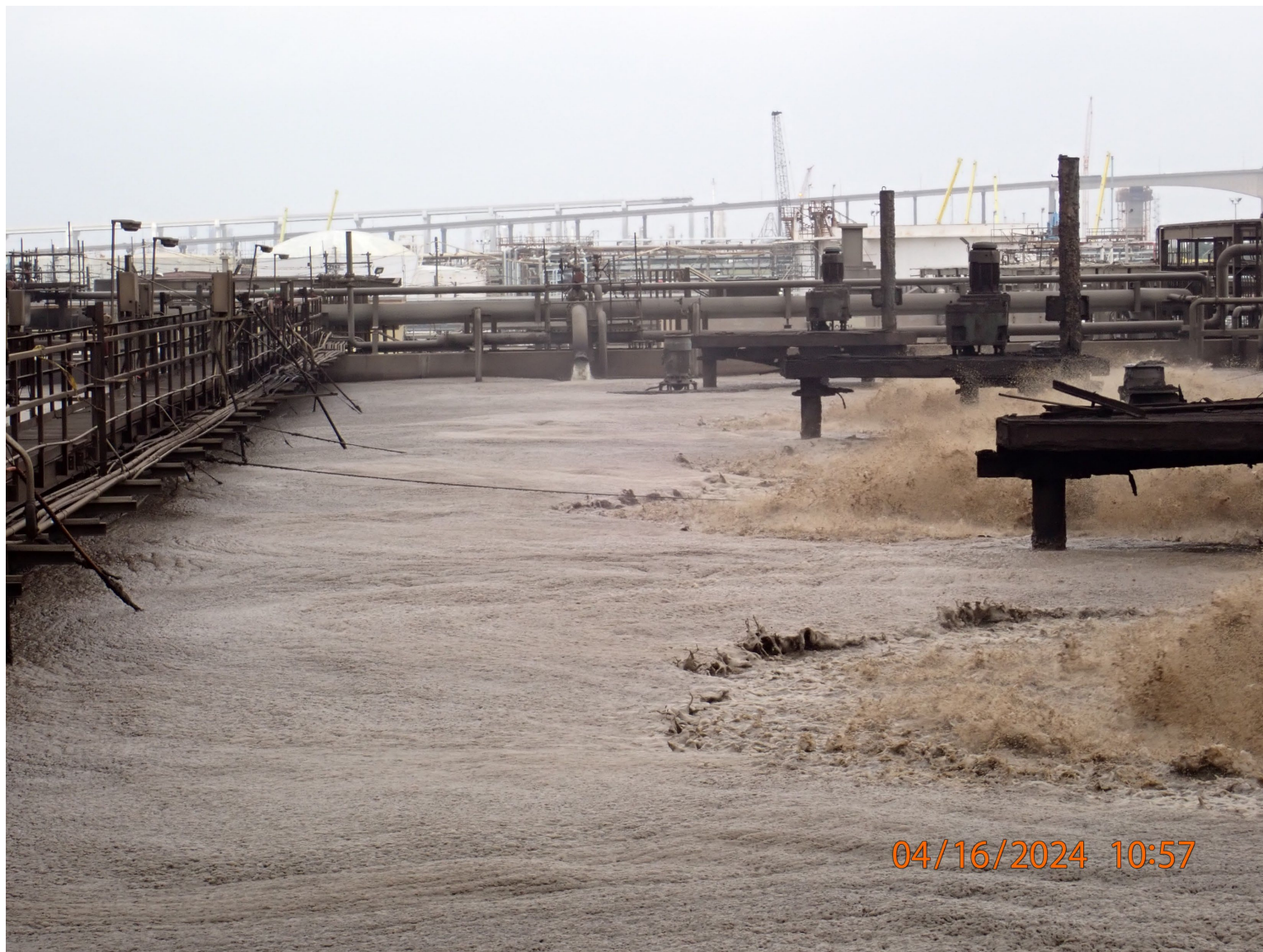
Photo 002: NET Aeration Basin and “Pour” Inlet, North Section 4/16/2024 09:57 P4160002.jpg
