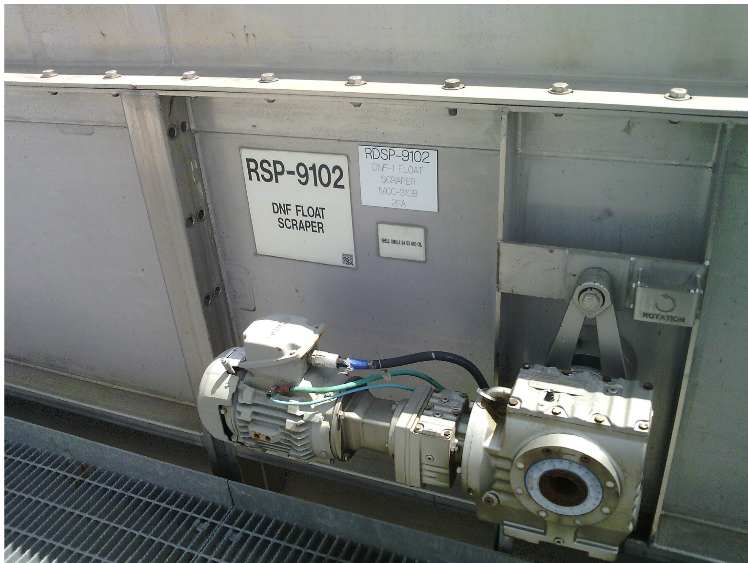
Photo 051: DNF TN-80010 float scraper RSP-9102 - 4/18/2024 12:03 FLIR0051.jpg
