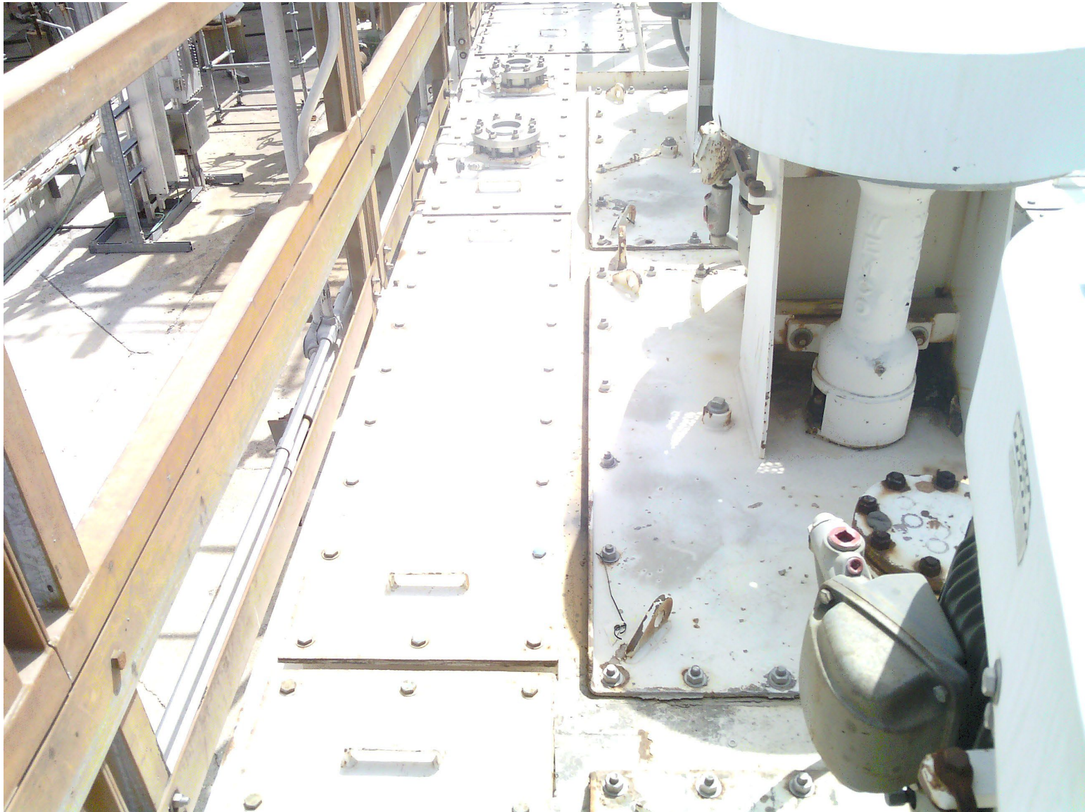
Photo 043: IGF #2 flange leak; 4/18/2024 11:27 FLIR0043.jpg
