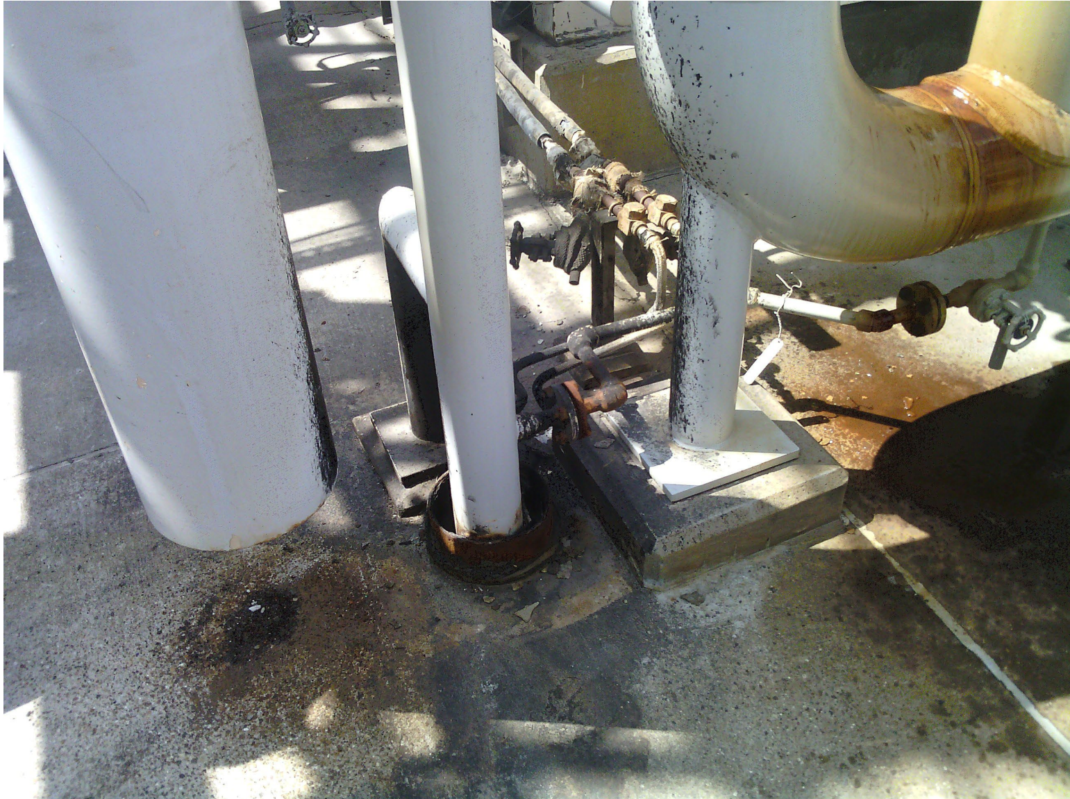
Photo 046: IGF #1 water seal drain - 4/18/2024 11:31 FLIR0046.jpg
