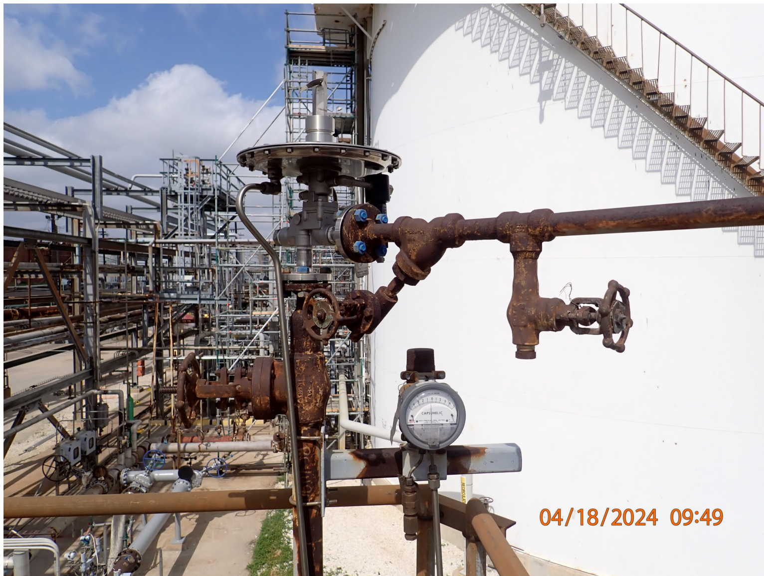
Photo 027: CPI #1 nitrogen blanket pressure gauge - 04/18/2024 09:49 P4180027.jpg
