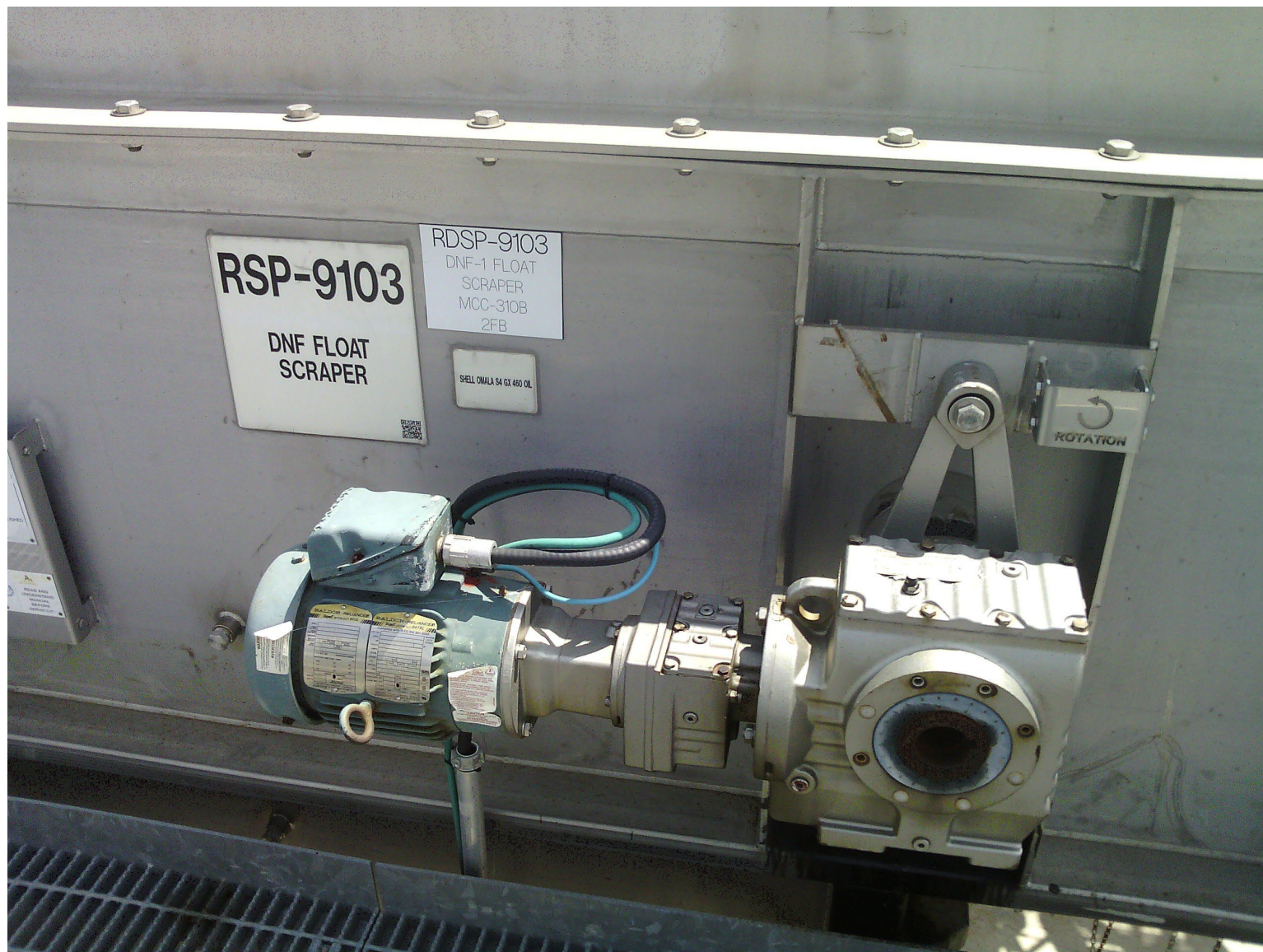
Photo 050: DNF TN-80010 float scraper RSP-9103 - 4/18/2024 12:03 FLIR0050.jpg
