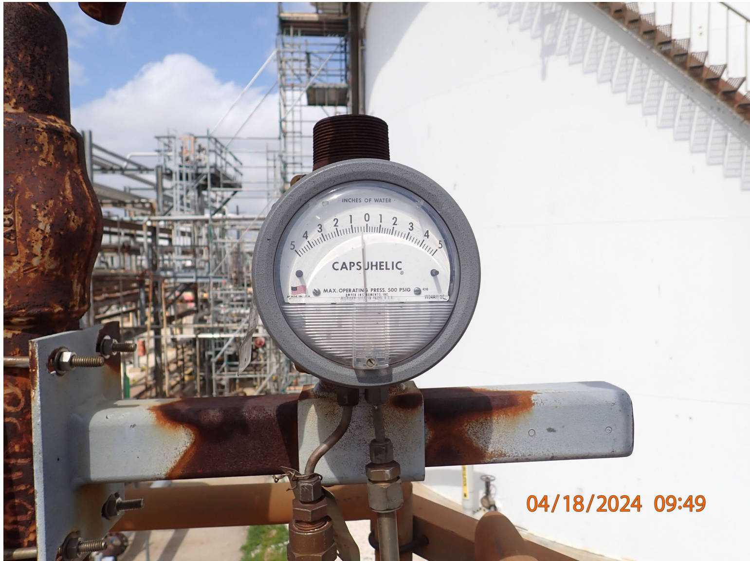
Photo 026: CPI #1 nitrogen blanket pressure gauge - 4/18/2024 09:49 P4180026.jpg
