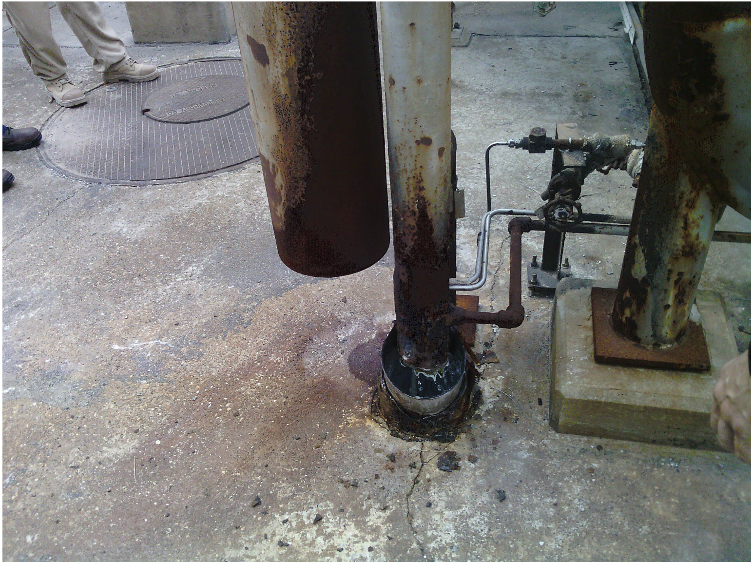
Photo 036: IGF #2 water seal drain - 4/18/2024 10:09 FLIR0036.jpg
