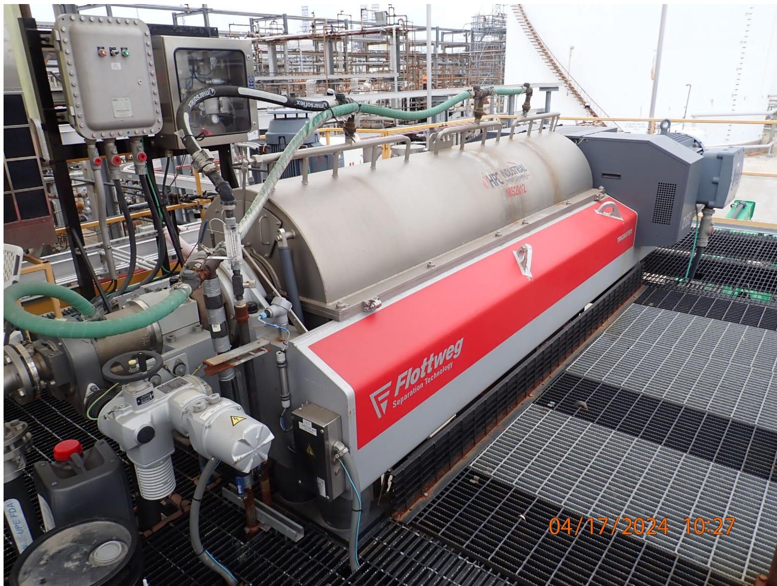
Photo 016: Clean Harbors sludge removal centrifuge 4/17/2024 10:27 P4170016.jpg
