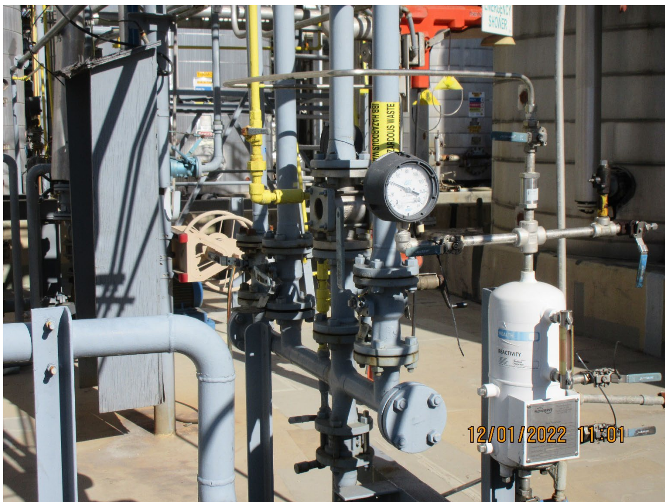
Photograph 4 – Ancillary equipment to Tank T8155
