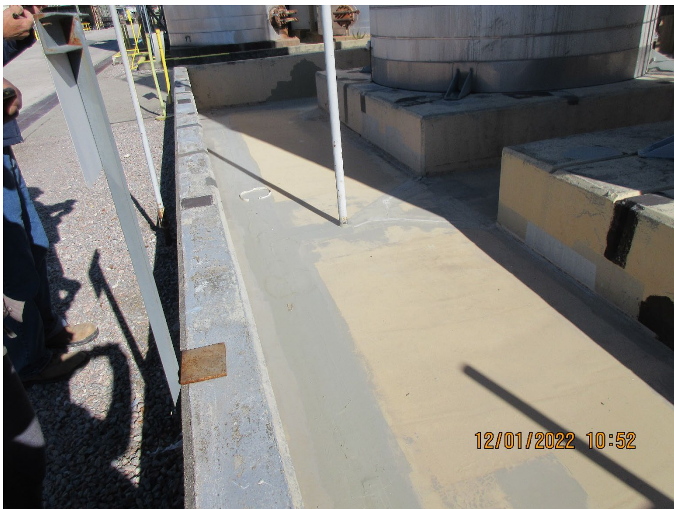
Photograph 3 – Secondary Containment for Tank 8155
