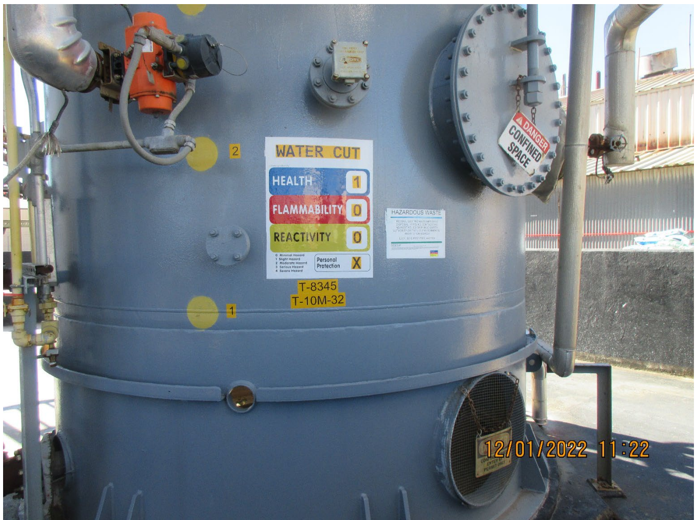
Photograph 7 – Hazardous Waste Tank T-8345
