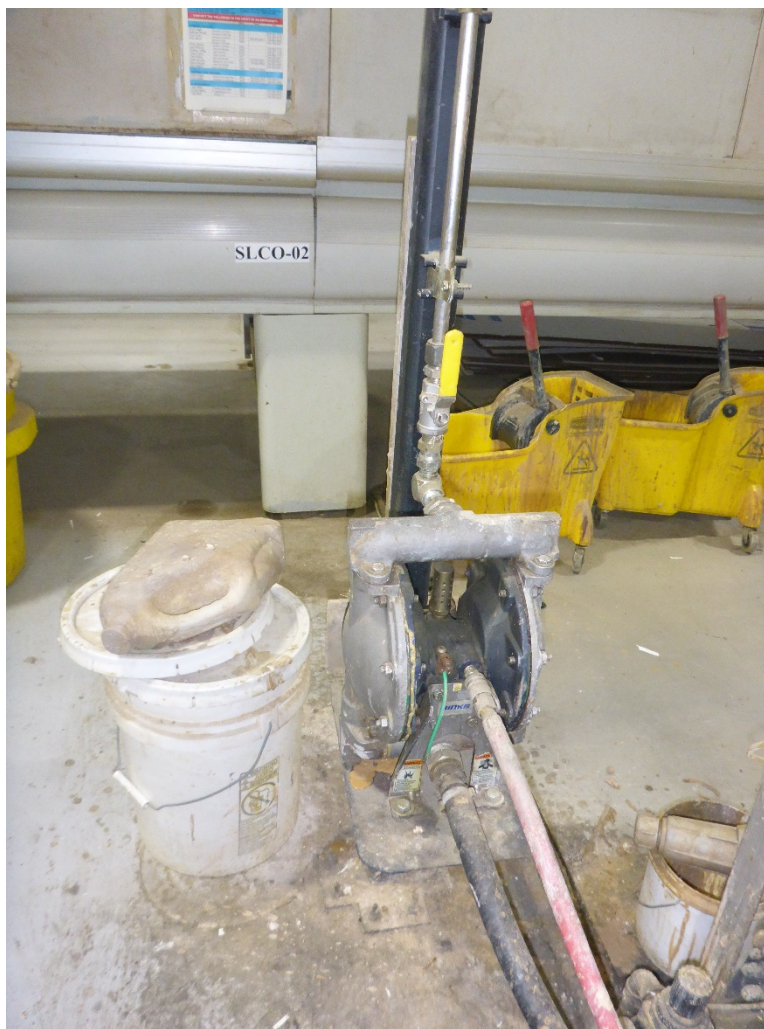
Photo 8: Dedicated pump and piping line to transfer spent solvents from the storage tank into the distillation unit.
