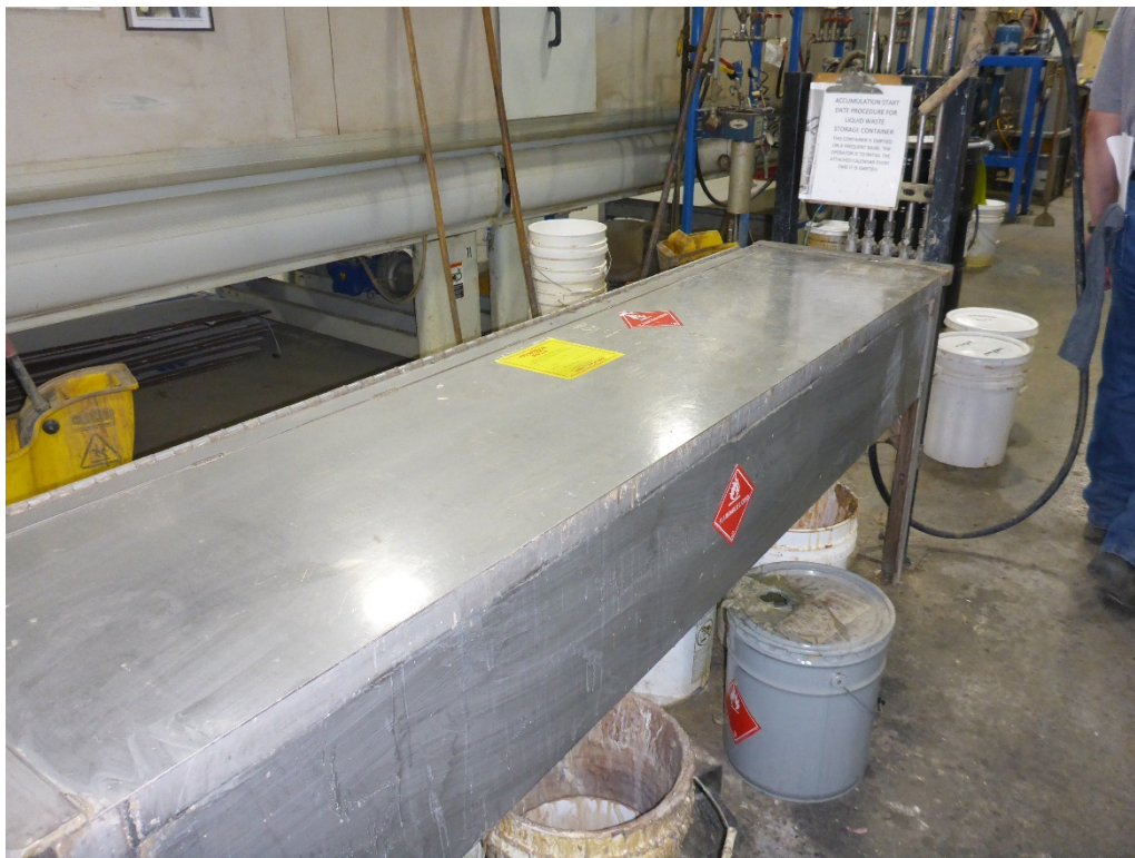
Photo 6: Small tank located between the spray coat line and the roll coat line in the Wood Plant. Tank is labeled D001 / F003 / F005 hazardous waste acetone and identified with a flammable liquid hazard placard.
