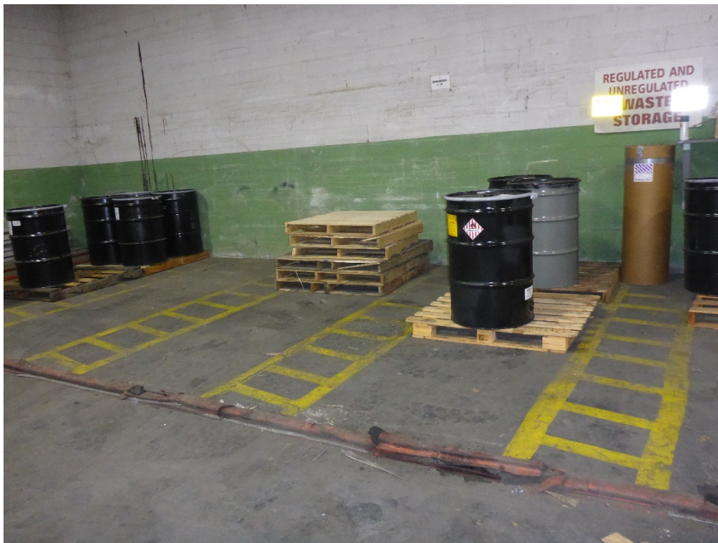
Photo 15: Main hazardous waste central accumulation area. Several gaps in the secondary containment berm around the perimeter of the area.
