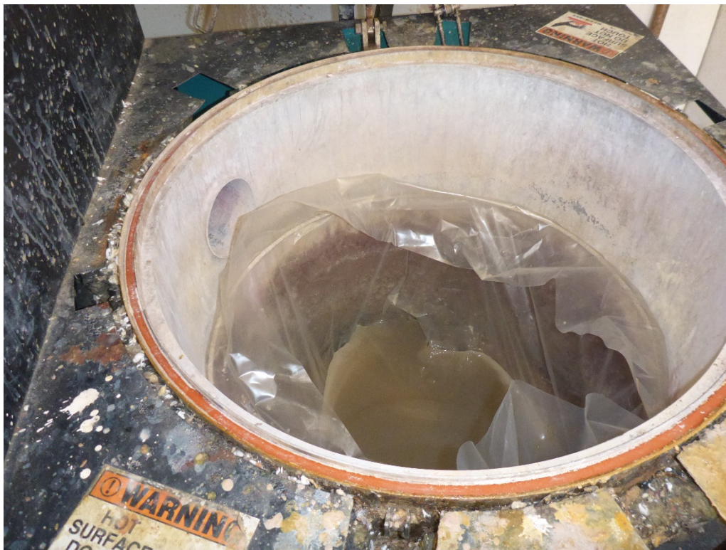
Photo 2: Spent solvent liquids inside the open distillation unit.
