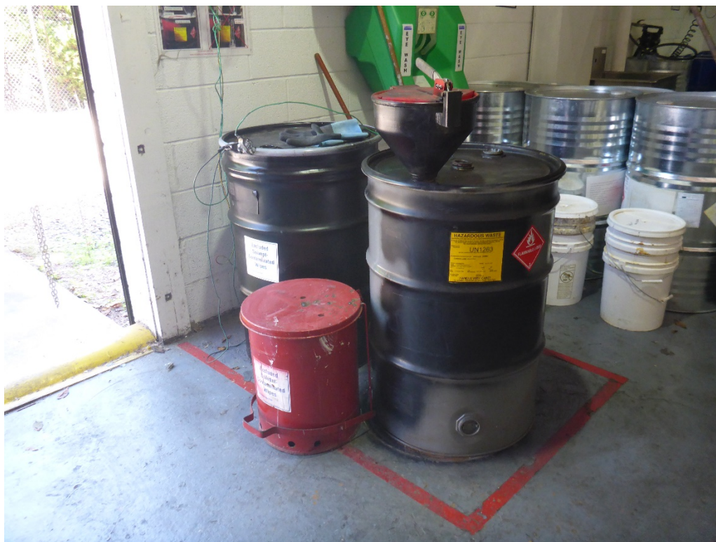
Photo 5: Wood Plant SAA for accumulating waste in the stain pump room. One 55-gallon drum and one red flip-top flammable can each labeled excluded solvent contaminated wipes located on the left, and one 55-gallon drum for accumulating waste paint related material located on the right. Drum on the right labeled D001 / F003 / F005 hazardous waste paint related material and identified with a flammable liquid hazard placard.
