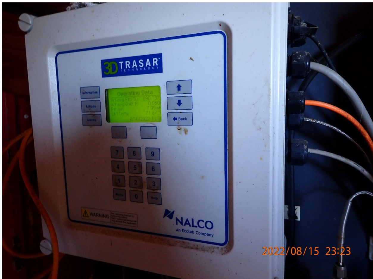
Photo 5 - 3DT Control Panel
