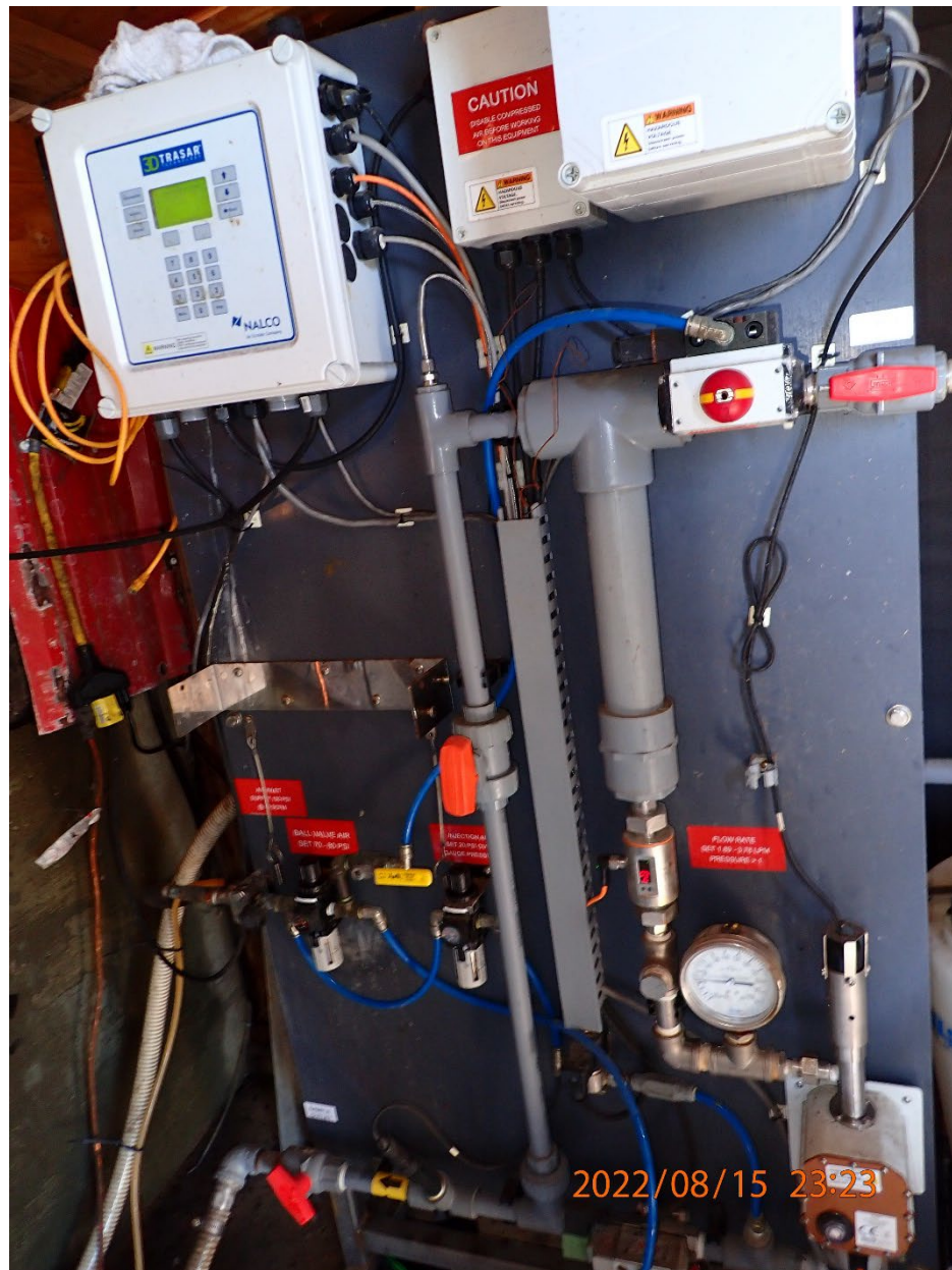
Photo 6 - Pressurize Air Control System
