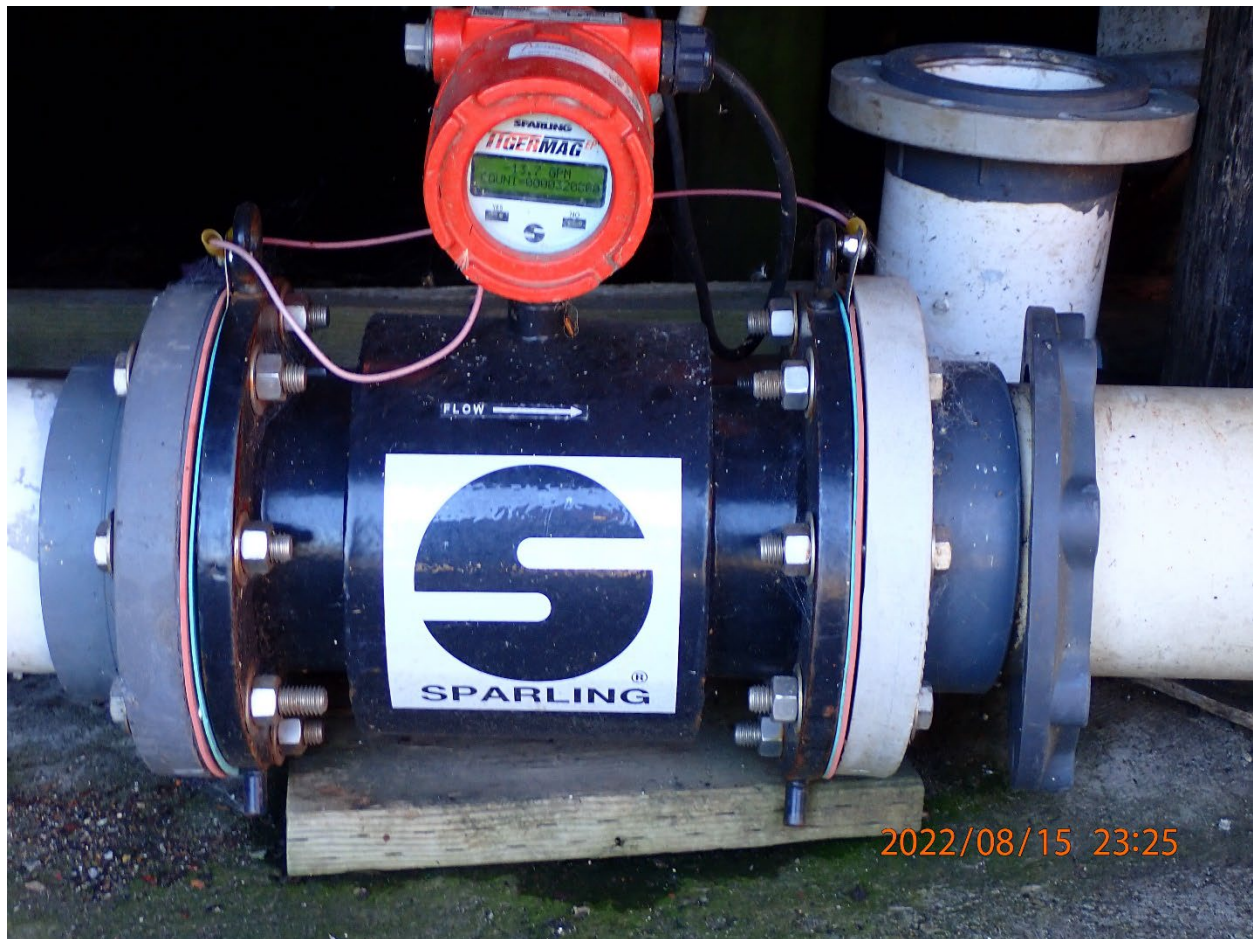
Photo 9 - Sparling Flow Meter
