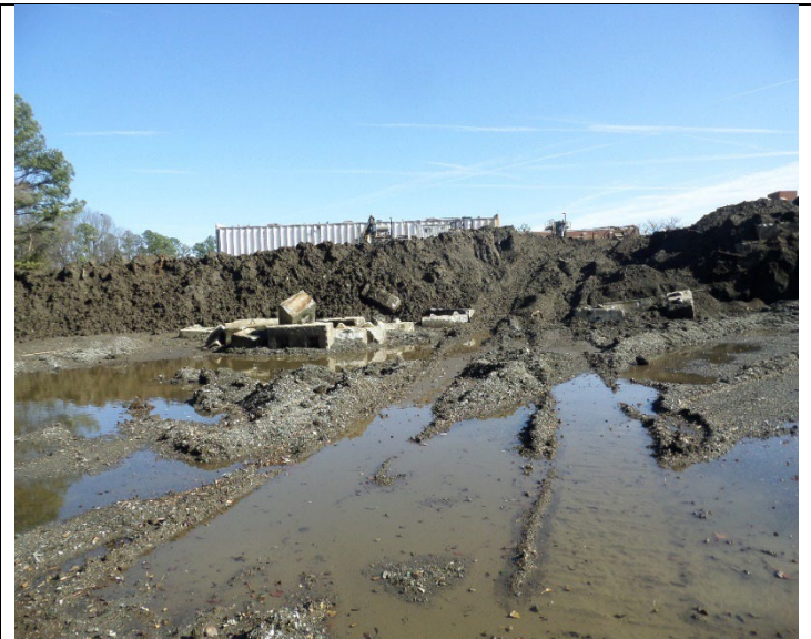
Keebler West Pile Area. The inspectors observed ASR material accumulating on the ground in piles. Photograph 32 taken at 1:47 p.m.
