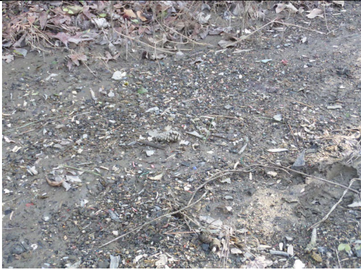
Access Path Next to Wooded Area Behind Keebler North Bunker Area. The inspectors observed a washout containing ASR material flowing from Outfall #3 pipe to the earthen access path. Distance from Outfall #3 pipe approximately 150-180 feet. Photograph 53 taken at 3:13 p.m.
