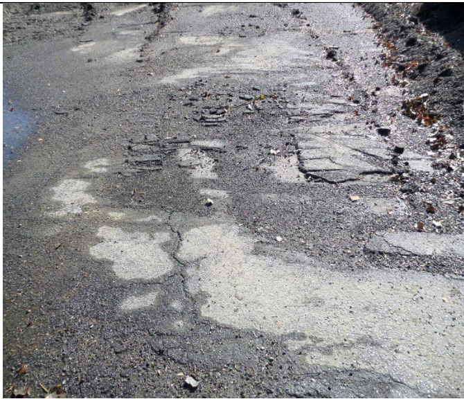
Keebler West Pile Area. The inspectors observed ASR material removed from the Keebler West storage area. The inspectors observed the original asphalt lot appeared worn, cracked and in disrepair. Photograph 31 taken at 1:38 p.m.
