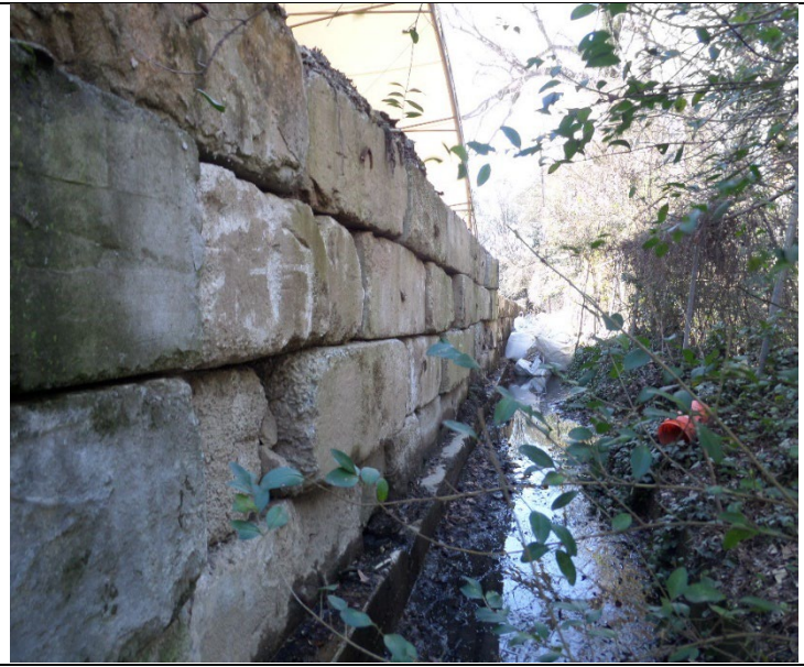
Keebler North Concrete Conveyance for Outfall #3. The inspectors observed ASR material accumulating on top of the Bunker block wall. Photograph 50 taken at 3:06 p.m.
