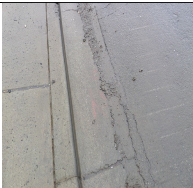
3320 Empire Boulevard. The inspectors observed ASR material on the east side of the road and north down the hill. Photograph 2 taken at 9:30 a.m.
