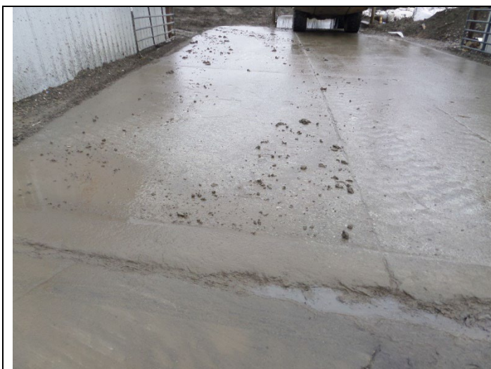
3320 Empire Boulevard. The inspectors observed the release of ASR material was from the 3320 Empire Boulevard south gate entrance. Photograph 5 taken at 9:30 a.m.
