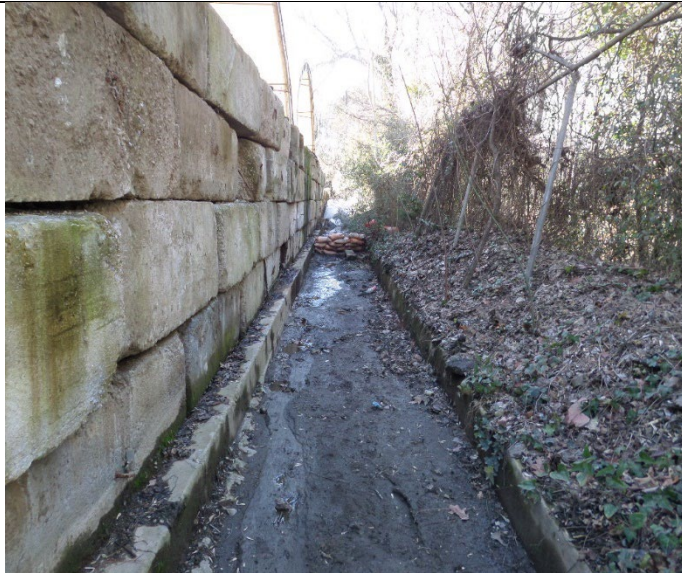
Keebler North Concrete Conveyance for Outfall #3. The inspectors observed ASR material and solids accumulating in the concrete conveyance and on soil surfaces. Photograph 51 taken at 3:07 p.m.
