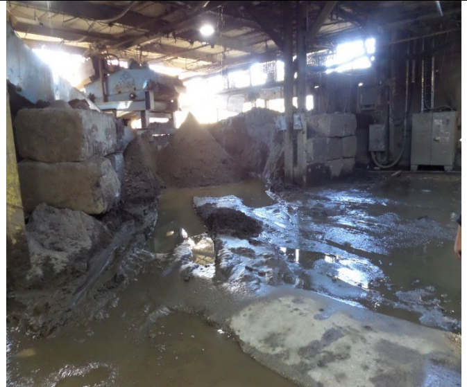
Keebler Plant Building Filter Press Area. The inspectors observed the area next to filter press contained wastewater and solids accumulating on the concrete floor. Photograph 38 taken at 2:07 p.m.
