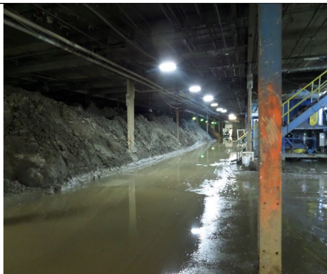
Keebler Plant Building Filter Cake Pile. The inspectors observed wastewater and solids accumulating on the concrete floor next to the Pile. Photograph 42 taken at 2:29 p.m.
