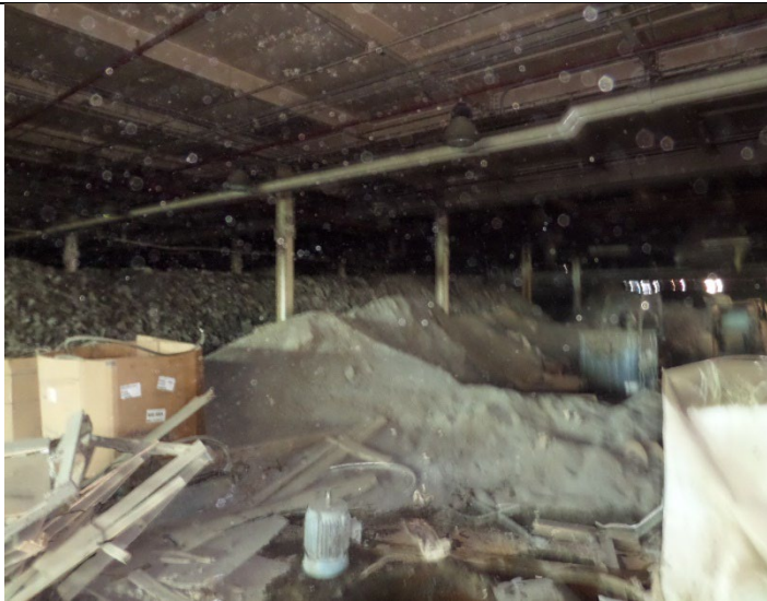
Keebler Plant Building Filter Cake - Backside Pile. The inspectors observed filter cake in this area. Photograph 45 taken at 2:35 p.m.
