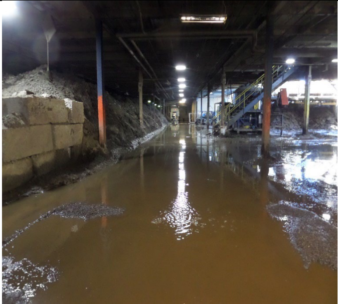
Keebler Plant Building Filter Cake Pile/Alley Way. The inspectors observed wastewater and solids accumulating on the concrete floor in the alley way next to filter cake storage area. Approximated several inches of water throughout the area. Photograph 39 taken at 2:08 p.m.
