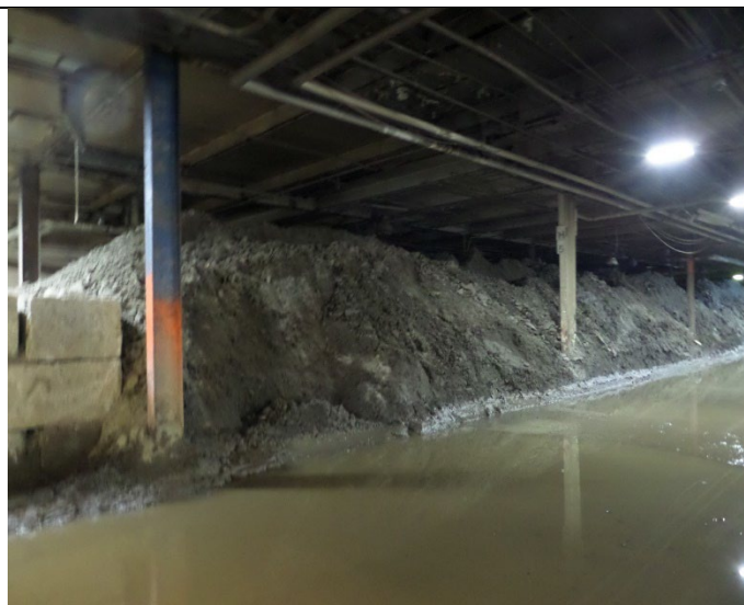
Keebler Plant Building Filter Cake Pile. The inspectors observed wastewater and solids accumulating on the concrete floor next to the Pile. Photograph 41 taken at 2:29 p.m.
