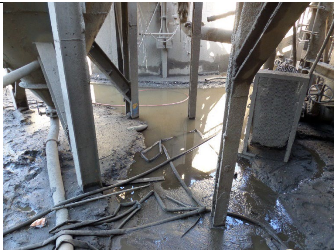
Wastewater Treatment Area. The inspectors observed solids/sludge containing ASR material accumulating in this area. Photograph 35 taken at 2:04 p.m.
