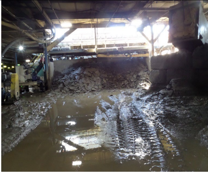
Keebler Plant Building Filter Press Area. The inspectors observed filter cake generated from the filter press accumulating with wastewater and solids on the concrete floor. Photograph 37 taken at 2:07 p.m.
