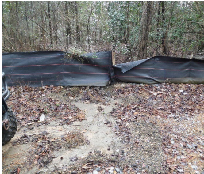
Access Path Next to Wooded Area Behind Keebler North Bunker Area. The inspectors observed a washout containing ASR material flowing from Outfall #3 pipe to the earthen access path. Distance from Outfall #3 pipe approximately 150-180 feet. Photograph 15 taken at 11:09 a.m.
