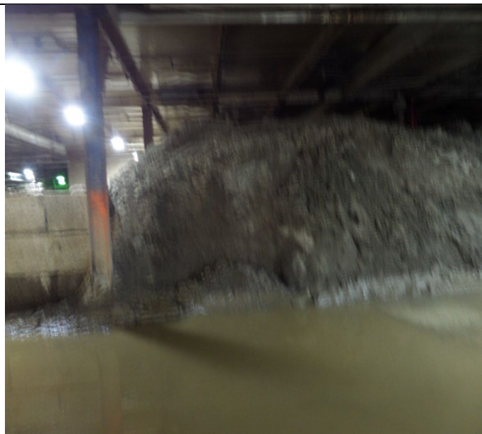
Keebler Plant Building Filter Cake Pile. The inspectors observed wastewater and solids accumulating on the concrete floor next to the Pile. Photograph 43 taken at 2:30 p.m.
