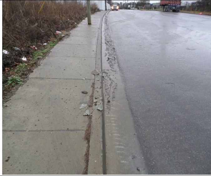
3320 Empire Boulevard. The inspectors observed ASR material on the east side of the road and north down the hill. Photograph 13 taken at 10:29 a.m.
