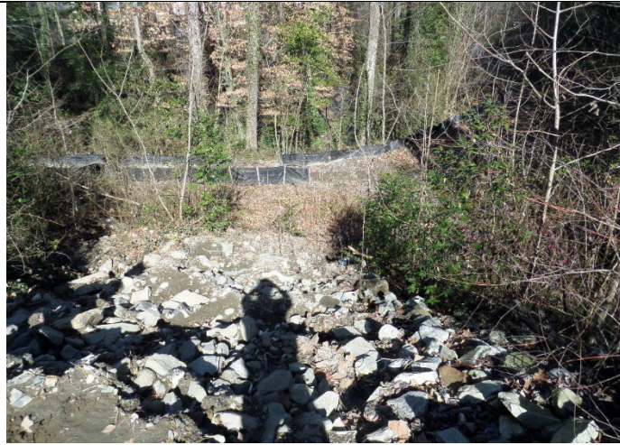
Outfall #2 Area - Keebler West. The inspectors observed apparent ASR material released to rip rap. Rip rap continues downhill to earthen access path and unnamed tributary. Photograph 27 taken at 1:24 p.m.
