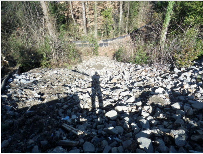
Outfall #2 Area - Keebler West. The inspectors observed apparent ASR material released to rip rap. Rip rap continues downhill to earthen access path and unnamed tributary. Photograph 29 taken at 1:29 p.m.
