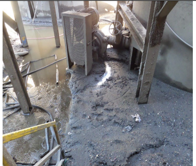
Wastewater Treatment/Area. The inspectors observed solids/sludge containing ASR material accumulating in this area. Photograph 34 taken at 2:02 p.m.
