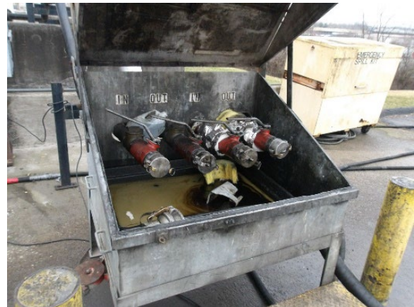
Picture 17: Overflow transfer
