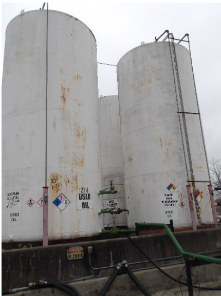
Picture 15: Used oil/oily water tanks (2) and cleaner solvent tank
