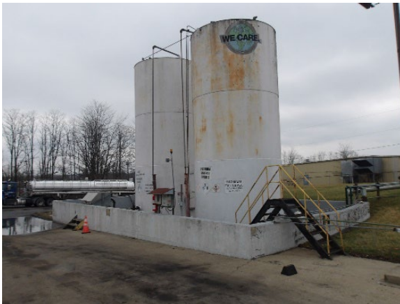
Picture 14 : Spent parts cleaner solvent and clean parts cleaner solvent tanks
