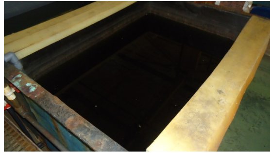
Photo #10 – Out of service zinc plating solutions stored in the large barrel line tank.
