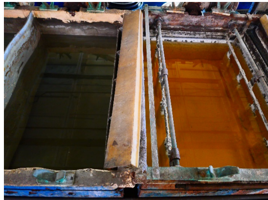
Photo #6 – Out of service zinc plating solutions stored in the large barrel line tanks.
