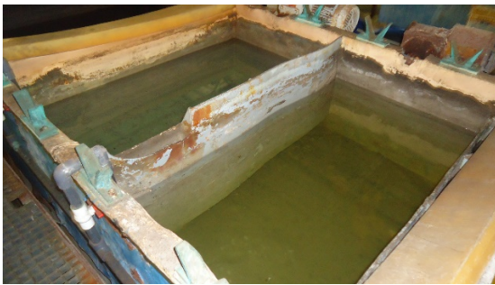
Photo #9 – Out of service zinc plating solutions stored in the large barrel line tanks.
