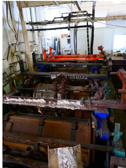
Photo #4 – Out of service/rusted zinc plating large barrel line tanks.
