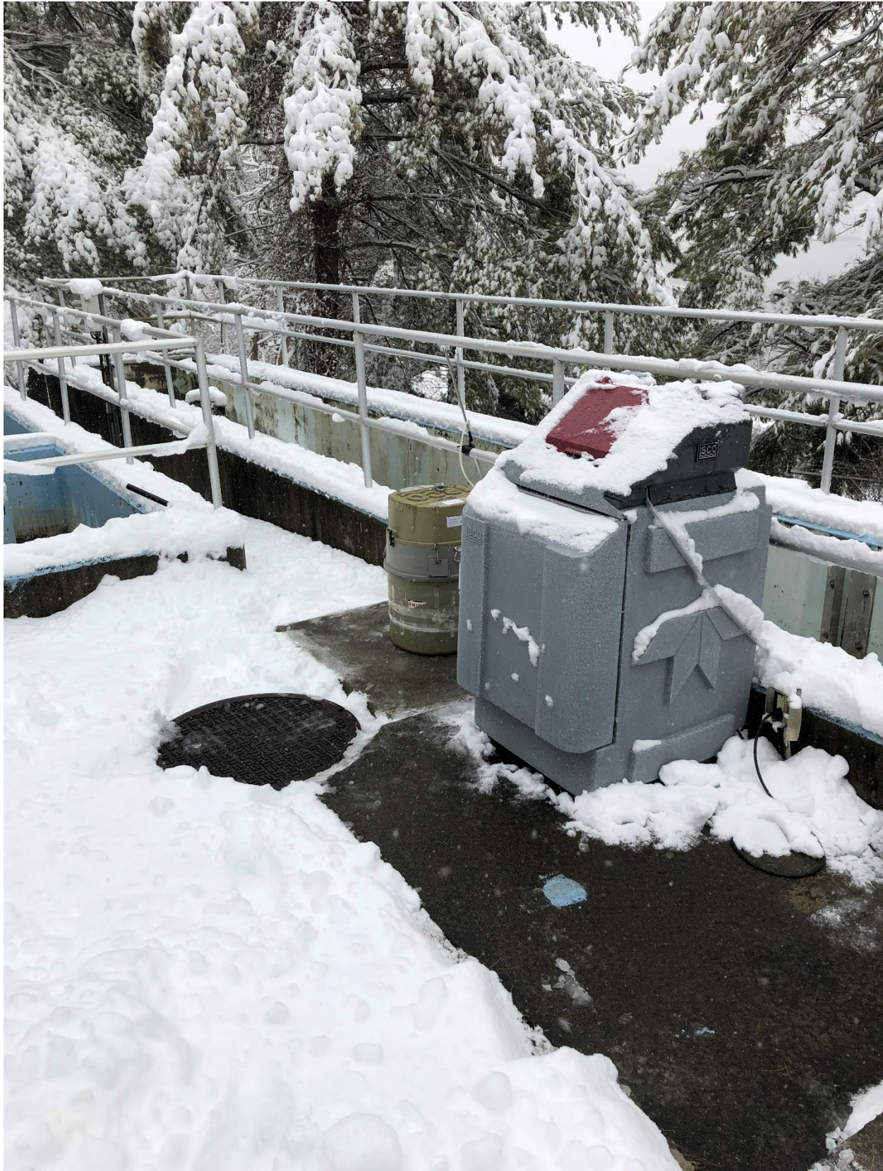
Photo #1: View of the effluent sampling location for Outfall 002.
