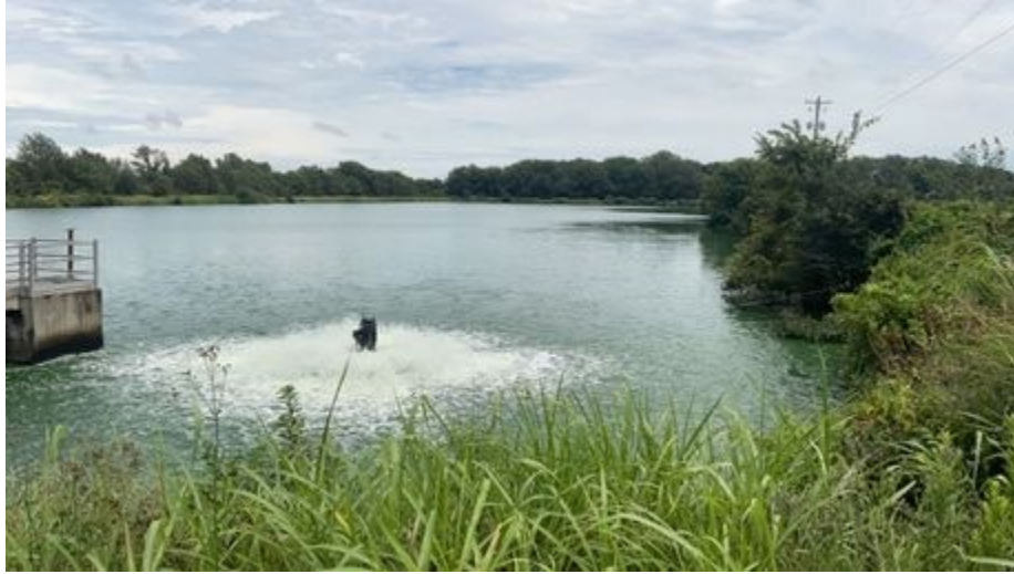
Lagoon with one floating aerator by discharge point. Taken 8/8/23 16:15pm
