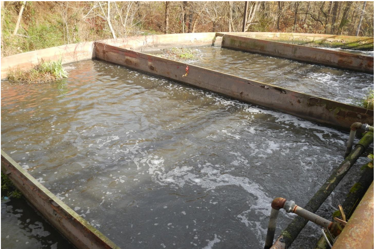
Photo 4. Aeration basin MLSS appears very dilute.
