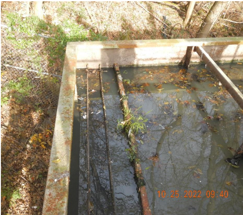
Photo 6. Clarifier chamber. Solids and vegetative growth observed.
