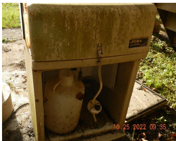
Figure 3: Effluent composite sampler.
