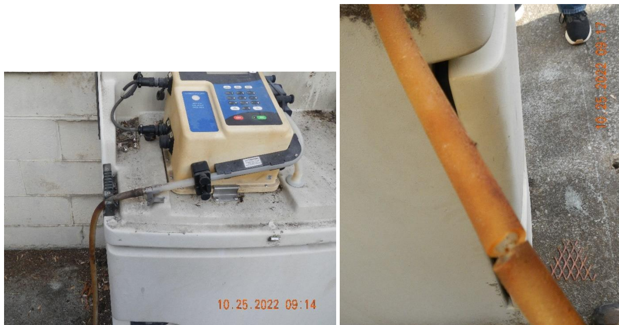
Figure 2: Influent composite sampler. The photo on the right is the suction line from the sampler.
