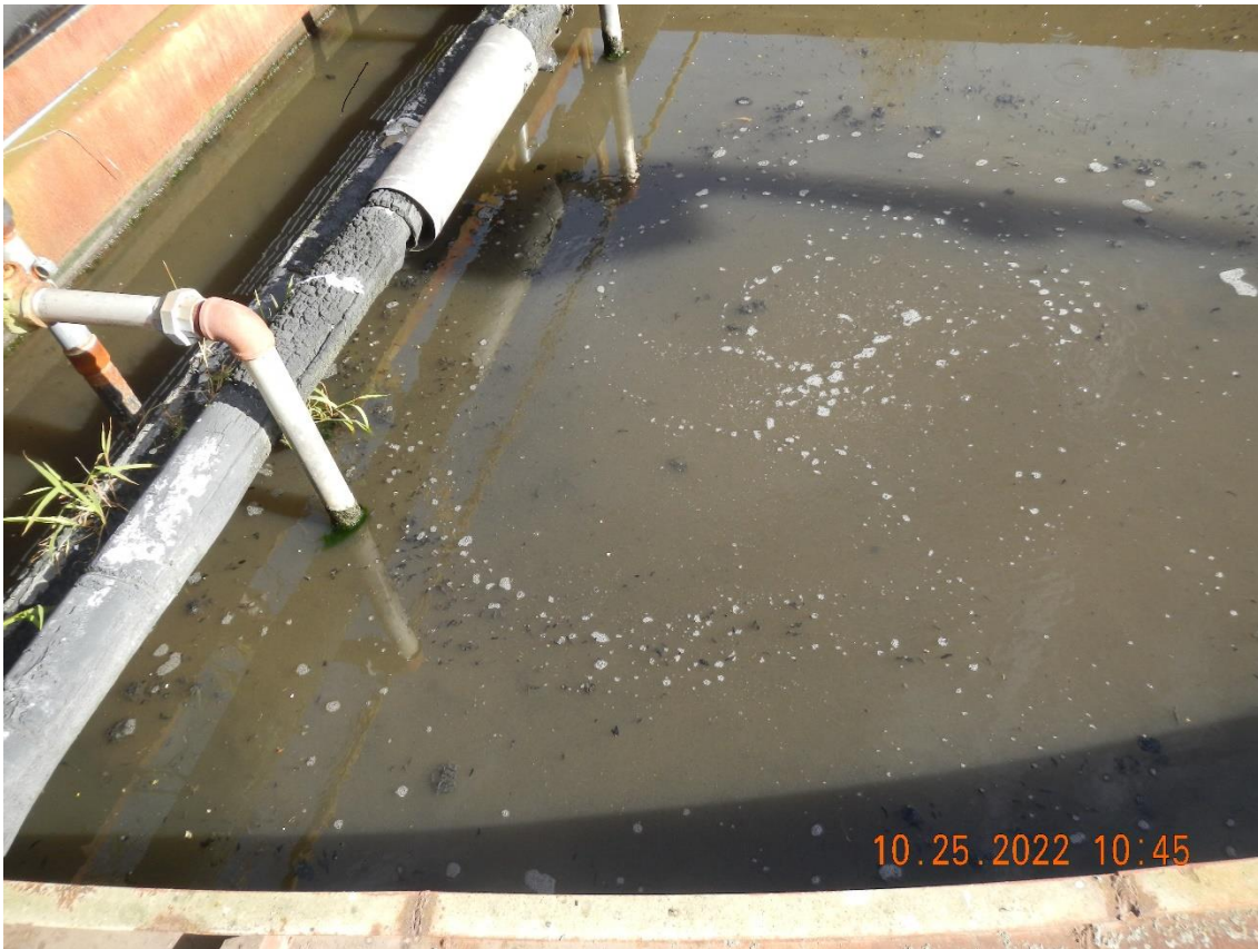
Photo 5. Aeration chamber. Black clumps of solids floating at the surface.
