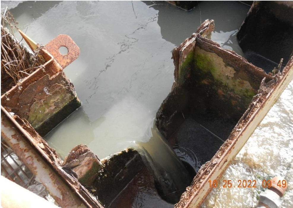
Photo 3. Influent box discharges into the aeration basin.
